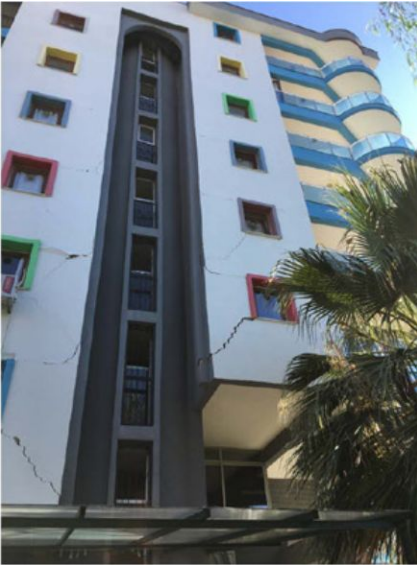
Damage to infills 2
