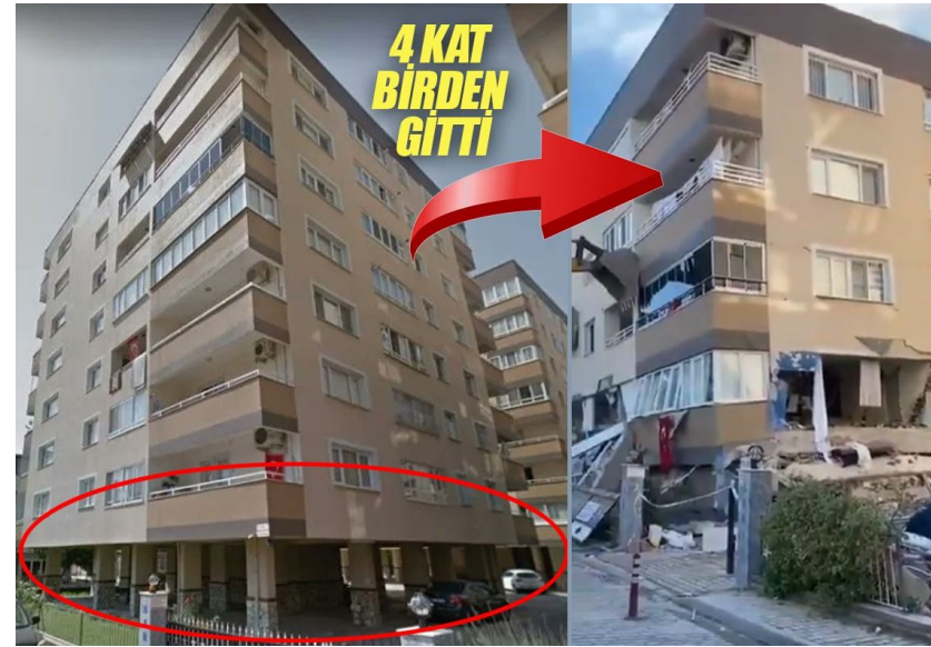
Collapse of two floors on the ground floor of the 8-storey Peace Site in Balled support Bayraklı 5,6
