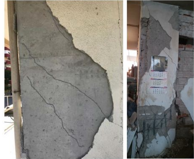
RC Column shear cracks 3
