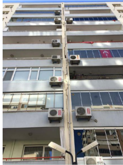
Pounding related damage 2
