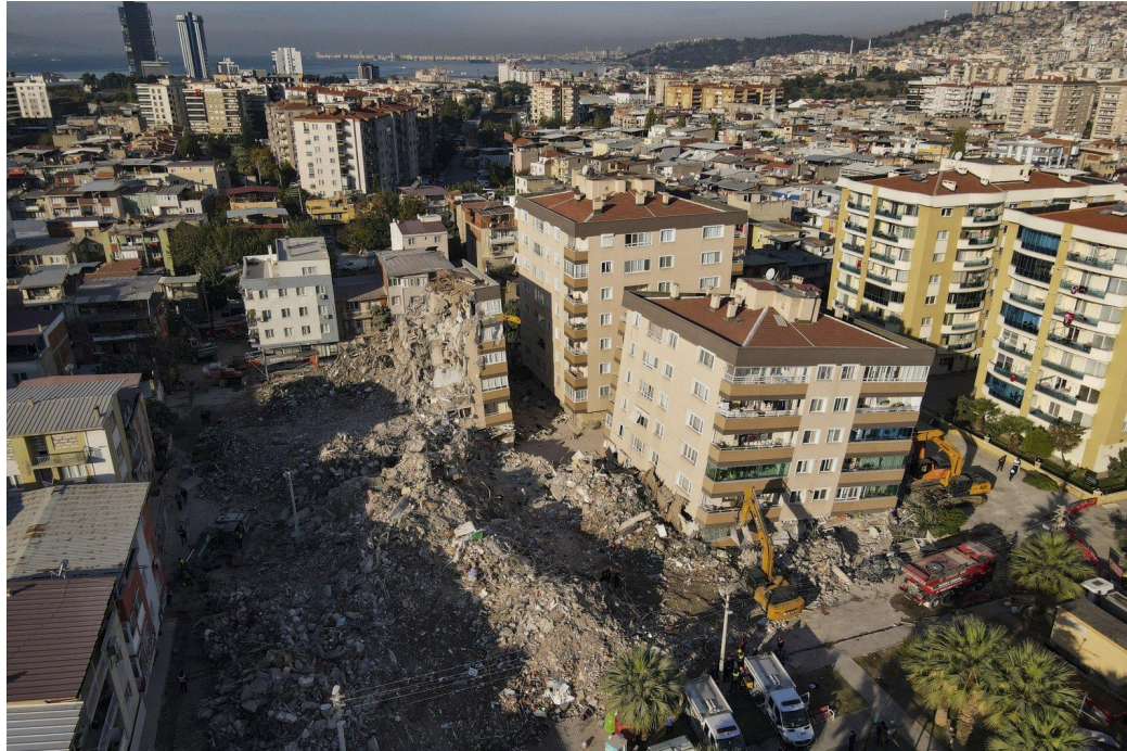
Collapsed buildings in part due to soil amplifications, Izmir 8
