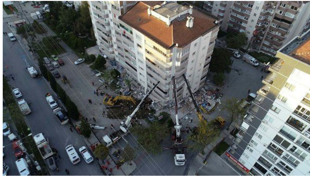
Failure of first 3 floors of a building in Demirkent Site in Bayraklı district 4
