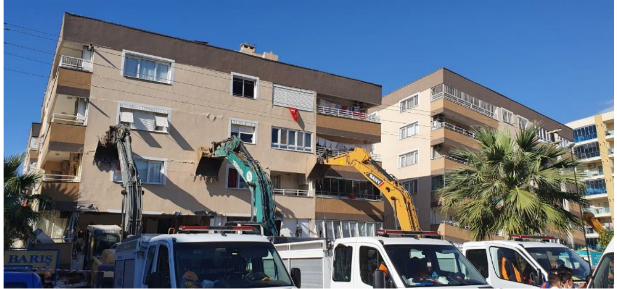
Failure of lower stories in an 8 story building 3
