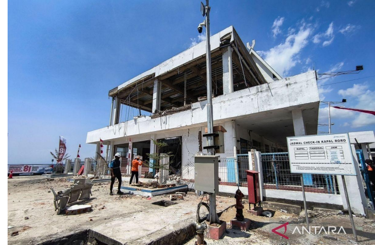
Damage at Laurentius Say Port, Maumere, Aug. 15 [13]
