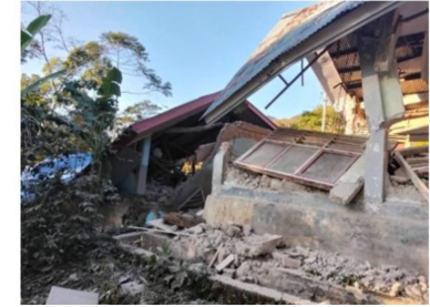
A damaged junior high school in East Manggarai [4]
