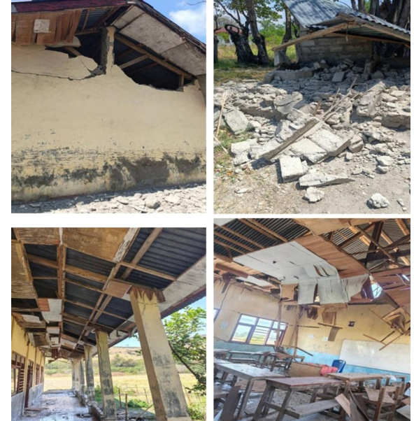
A damaged elementary school in East Manggarai [4]
