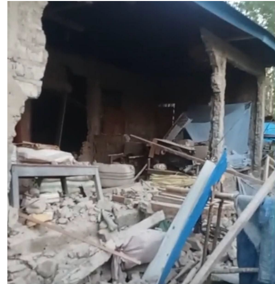
A severely damaged residence in Desa Traslok, Macang Tanggar [3]
