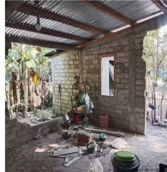
Example of masonry housing performance observed after the earthquake [2]
