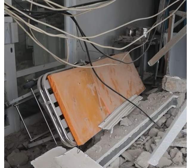
Damaged hospital room [11]
