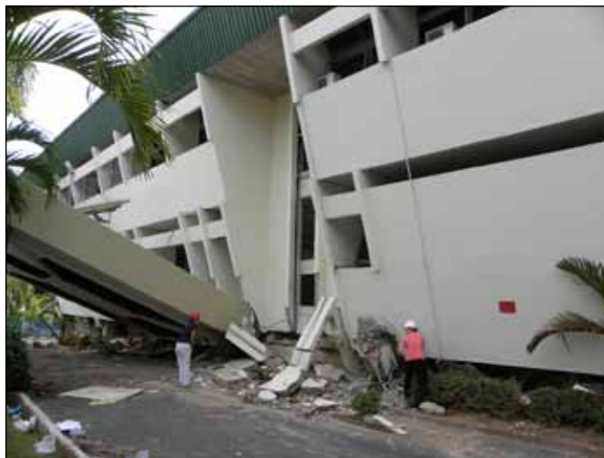
Team members Wood and Cedillos survey a collapsed (first-story) government building where two people were killed and 80 reportedly survived, some by rushing out of the first floor and others who remained in place on the upper floors.
