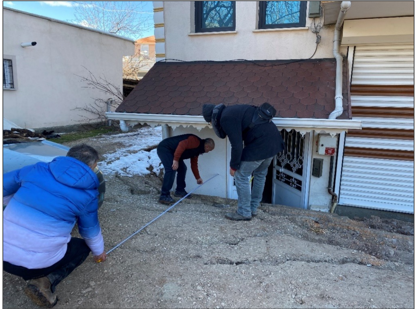
Liquefaction-induced settlement observed at Gölbaşı-Adıyaman
