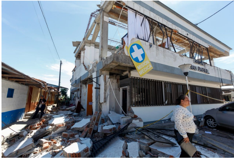
Structural damage in the front side of the San Rafael Hospital building, El Águila, Valle del Cauca region [14]
