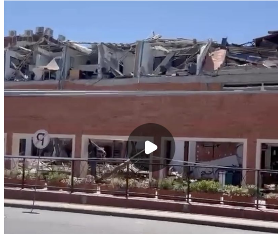
Structural collapse in the second story of the Comfamiliar Clinic administrative building [17]
