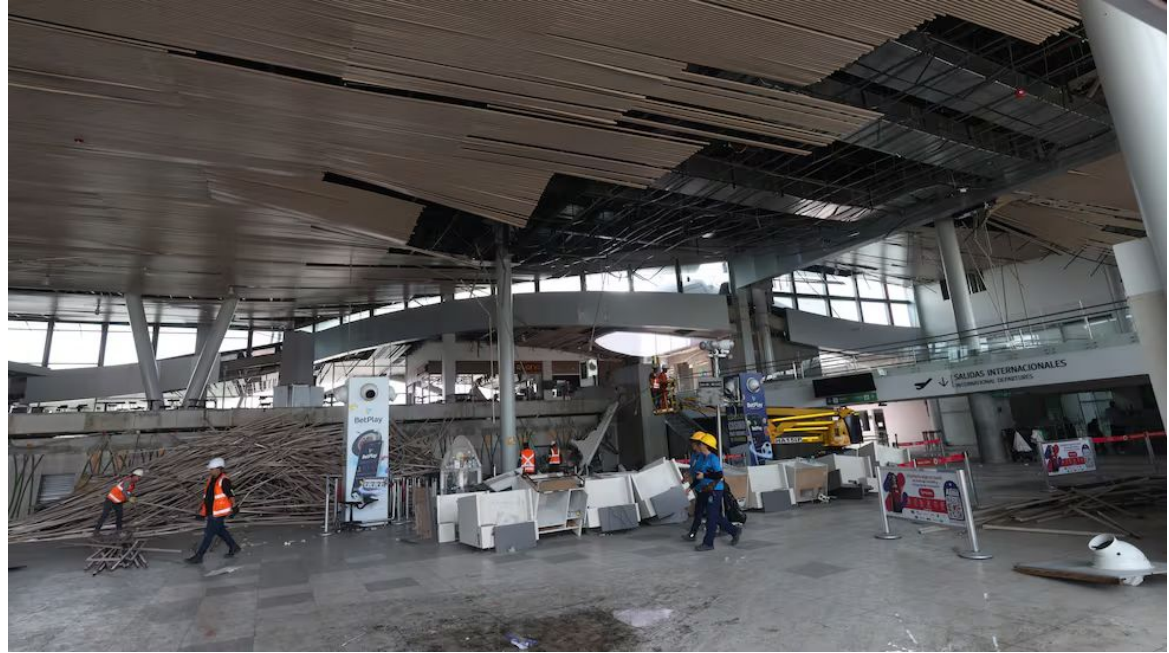
Non structural ceiling collapse during August 10, 2026 earthquake (Source: Semana [13])
