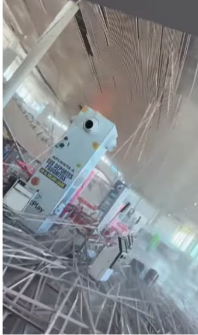
Non structural ceiling collapse during August 10, 2026 earthquake (Source: Sebastian Falla [15])
