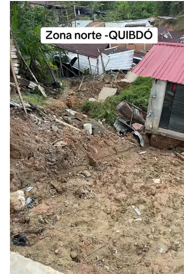
Slope failures, posted on TikTok [24]
