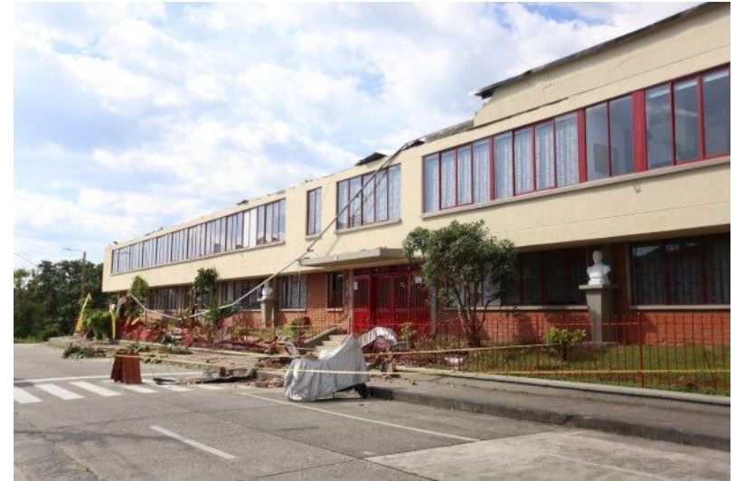
Partial structural collapse at Colegio de Cristo, Manizales, Caldas. Official diagnosis: “collapsed façade, major cracking and structural separation” (Manizales Municipal Government). Photo: Luis Fernando Trejos / [3]
