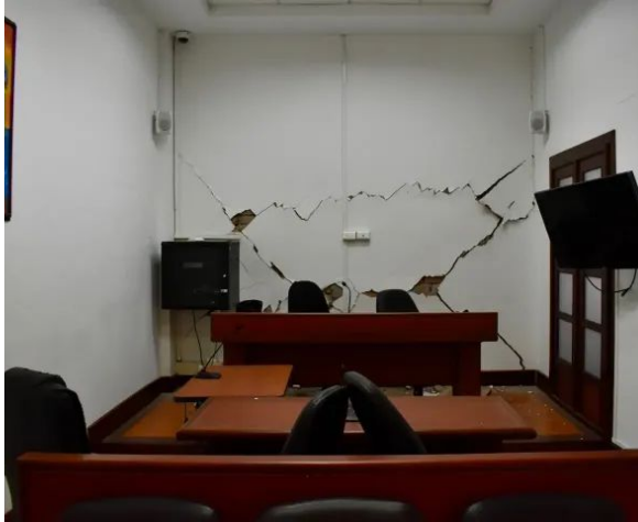
In-plane failure mode of interior masonry walls in The Caldas Governor's Office building in Manizales city (Photo: Government of Caldas; source: La Patria)[6]
