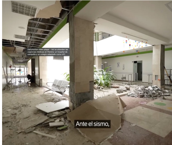
Apparent non-structural damage in the Comfamiliar Clinic building, Pereira city [10]
