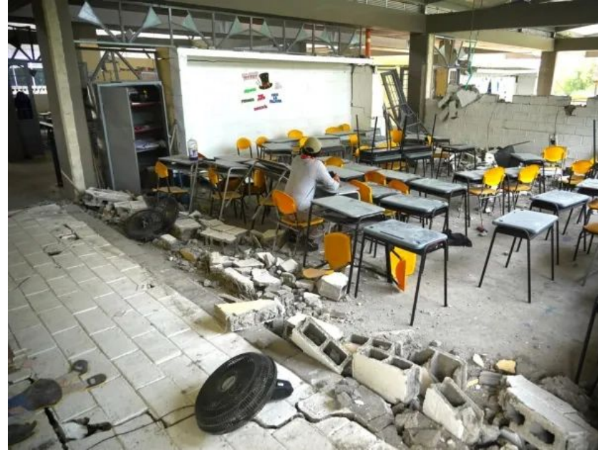
Partial and total collapse of interior walls in Instituto Educativo Integrado Carrasquilla Industrial at Quibdó, Chocó Region (Photo: Daniel Fernando López; source: El Tiempo) [8]
