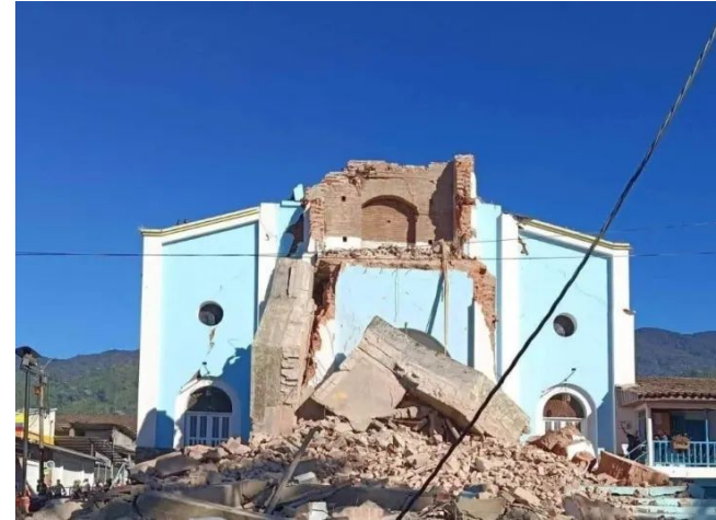
Severe structural damage of Parish Nuestra Señora del Perpetuo Socorro in Calima, Valle del Cauca regio (Photo: Private Archive; source: El Tiempo) [3]
