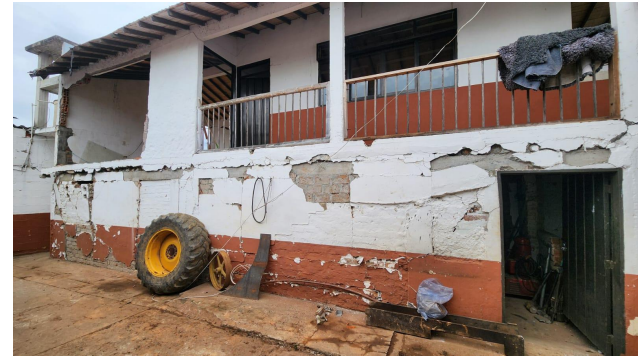
Damages in buildings located in rural areas. Photos: Juan C. Reyes (2026). [9]
