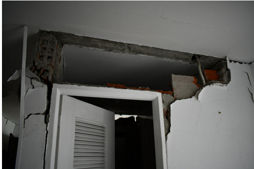
Damages in buildings located in Armenia. Photos: Francisco Galvis and Claudia Ramirez (2026). [8]
