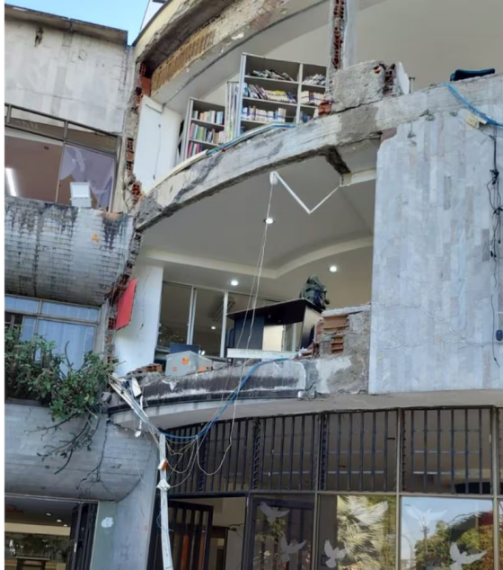
Out-of-plane collapse of part of the facade wall in Universidad Libre at Pereira, Risaralda Region (Photo: Private archive; source: Publimetro) [7]
