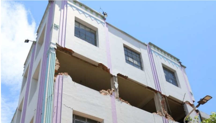
Partial structural collapse at Liceo Isabel la Católica, Manizales, Caldas. Official diagnosis: “collapsed ceilings and walls, major cracking and structural separation” (Manizales Municipal Government). Photo: Luis Fernando Trejos / [3]
