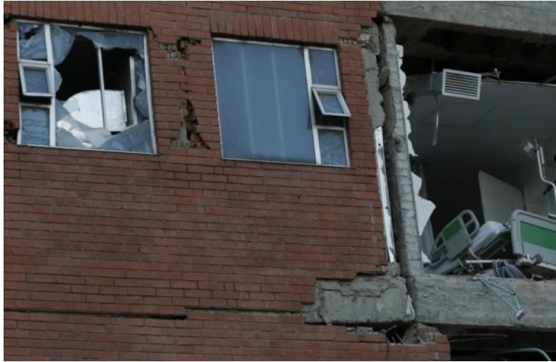
Non-structural damage of the Nuestra clinic building in Cali, Valle del Cauca region [4]
