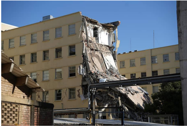
Structural collapse of the University Hospital building (built in 1956) in Cali, Valle del Cauca region [11]
