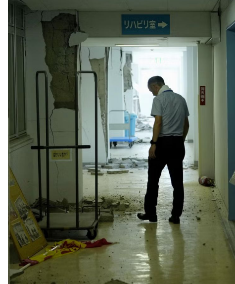
Damage to Minami Hospital in Uki City (Reuters) [8]
