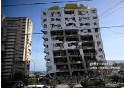
Structural damage in a multistory building in La Guaira. AP Photo/Juan Pablo Arreaz. [6]
