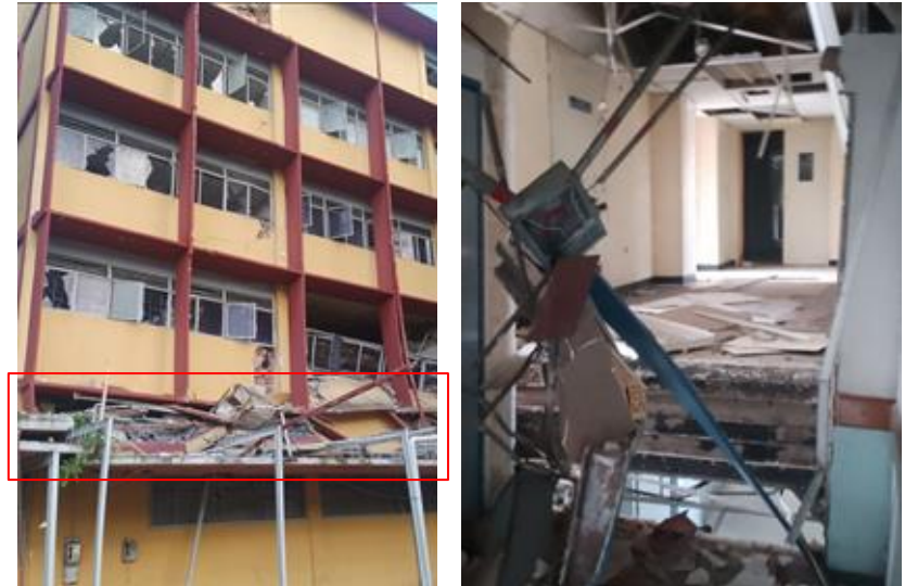
Structural and non-structural damage reported in the Francisco Antonio Ríquez de Cotiza hospital in Caracas. No fatalities were reported due to the collapse, but one three injured people were reported being referred to the Vargas hospital ( @caraotadigital , @dianavasquezve via Instagram). [15 ,16]
