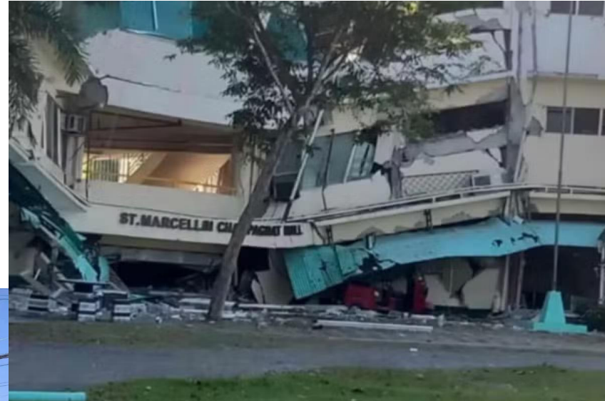
Notre Dame of Dadiangas University building collapse in General Santos, photographed by Br. Manuel de Leon, University President [5]
