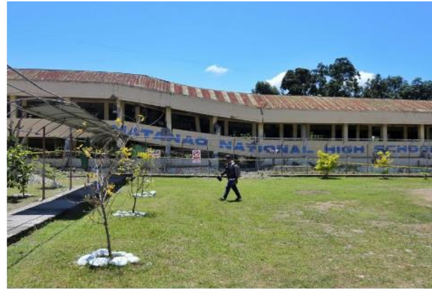
Matanao National High School, damaged by the 2019 earthquakes, collapsed after the earthquake, forcing students to take cover [7].
