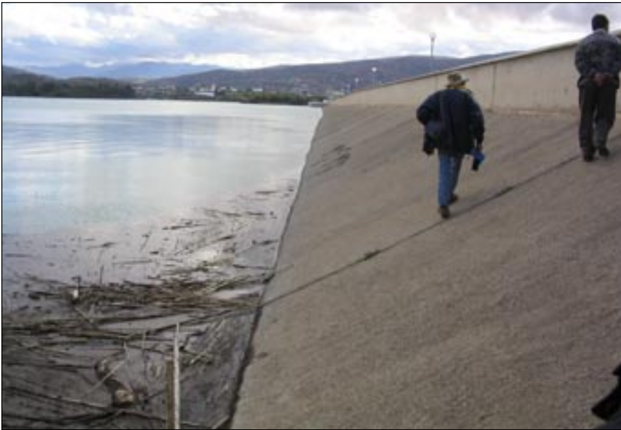
Figure 3. View of reinforced concrete face of the El Khattabi Dam from right abutment (photo: Youd).
