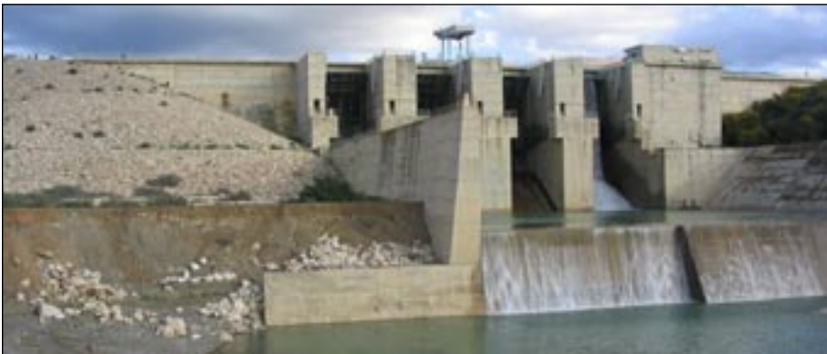
Figure 4. Junction between gravel embankment and concrete gravity sections of the El Khattabi dam (photo: Youd).
