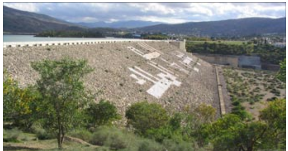
Figure 2. Post-earthquake view of the El Khattabi dam from right abutment (near the strong-motion instrument) (photo: Youd).
