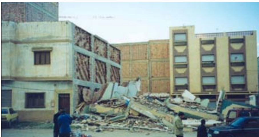
Figure 7 Collapsed building in foreground and undamaged buildings with typical construction in background (photo: Youd).
