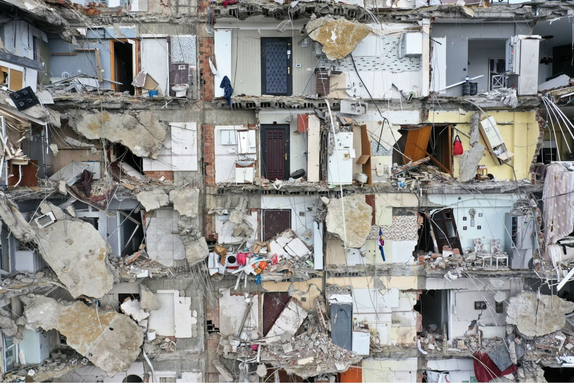
This aerial photo shows a damaged building in Adana. Oguz Yeter/Anadolu Agency via Getty Images
