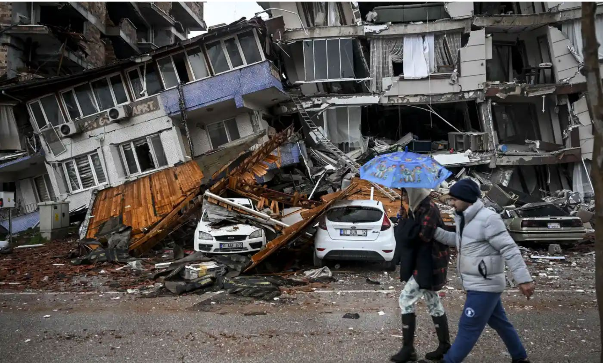
A view of a damaged building in Hatay, Turkey. Photograph: Anadolu Agency/Getty Images
