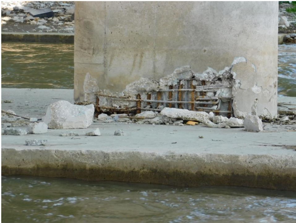
Figure 5-29 Plastic hinging at base of RC column, Bridge 2
