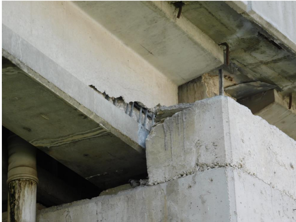
Figure 5-35 Close-up view of damage at end of Bridge 3 precast girder
