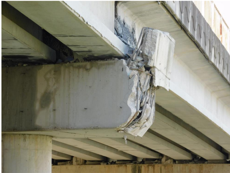
Figure 5-15 Closer view of failed exterior shear key and end-of-girder damage, Bridge 2
