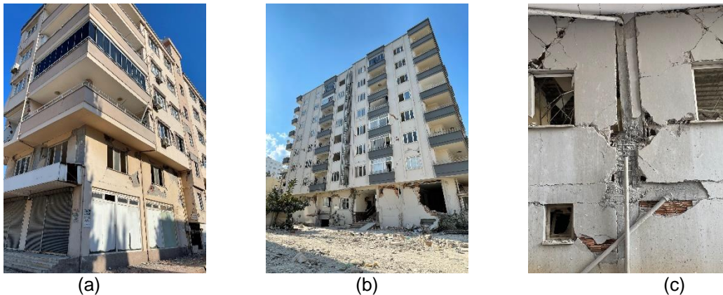
Figure 4-8 Residential building damages (a) due to overhangs, (b) captive/short column due to strong infill walls
