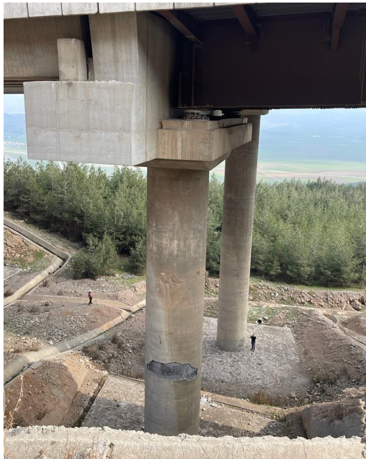
Figure 5-6 Overall view of bent with 10' diameter RC bridge columns and plastic hinge for one column at about 1/4 the way up its height, Bridge 1
