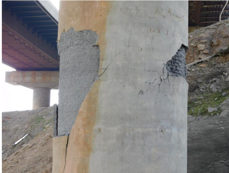
Figure 5-8 Side view of plastic hinge region of 10' diameter RC bridge column, Bridge 1
