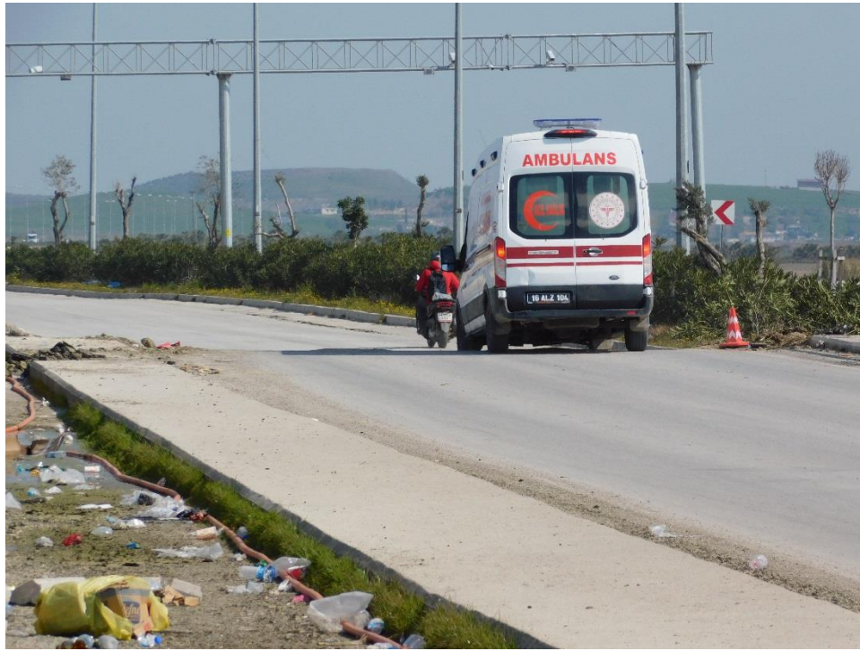
Figure 5-31 Settlement of approach to bridge, View 2, Bridge 2
