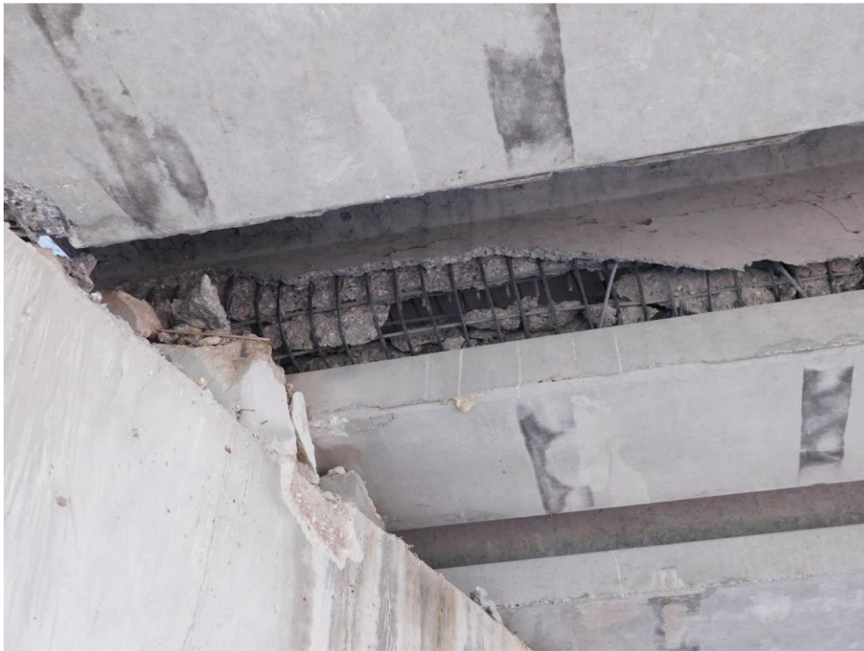
Figure 5-25 Significant interior girder damage at end of precast girder, Bridge 2
