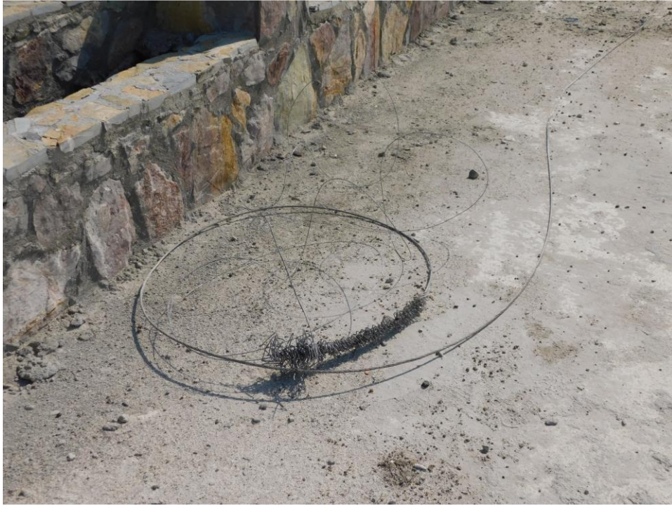
Figure 5-21 Prestressing cable at end of precast girder, Bridge 2
