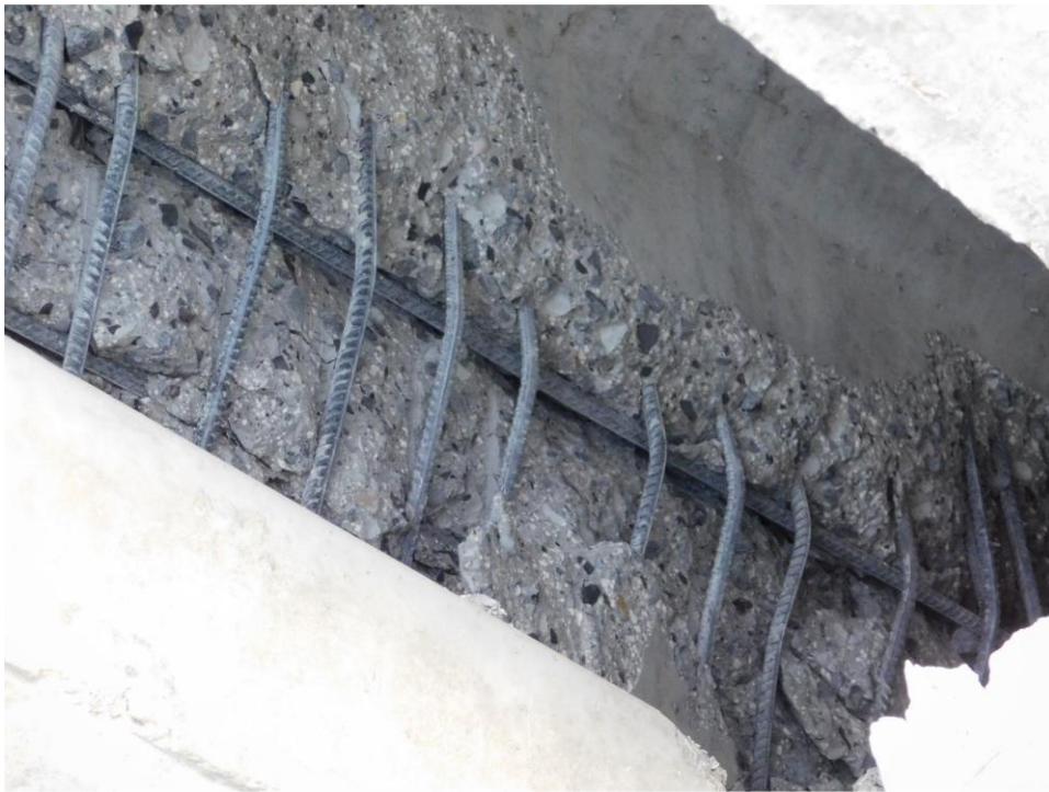
Figure 5-24 Close-up view of interior girder damage at end of precast girder, Bridge 2
