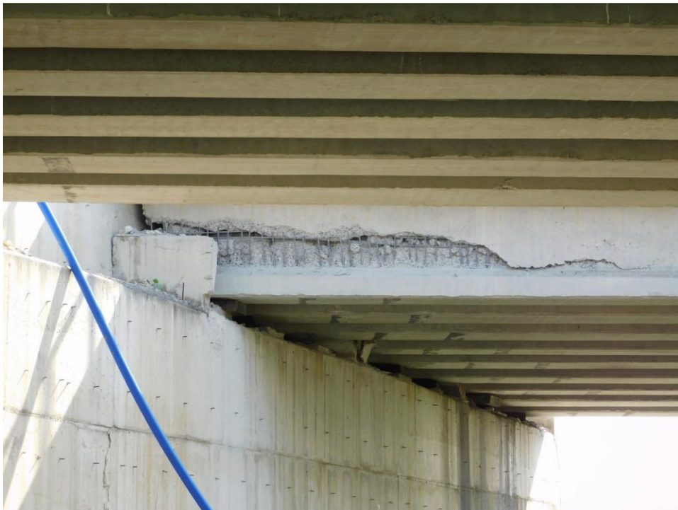
Figure 5-20 Damage over long range to end of exterior precast girder, Bridge 2
