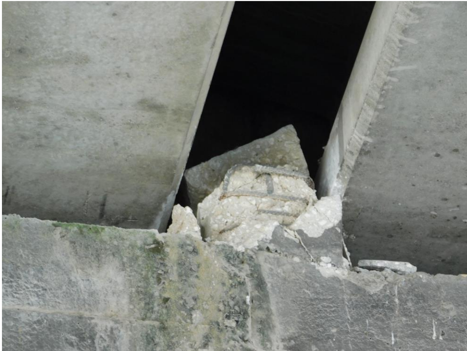
Figure 5-37 Damage of internal shear key at bent of Bridge 3
