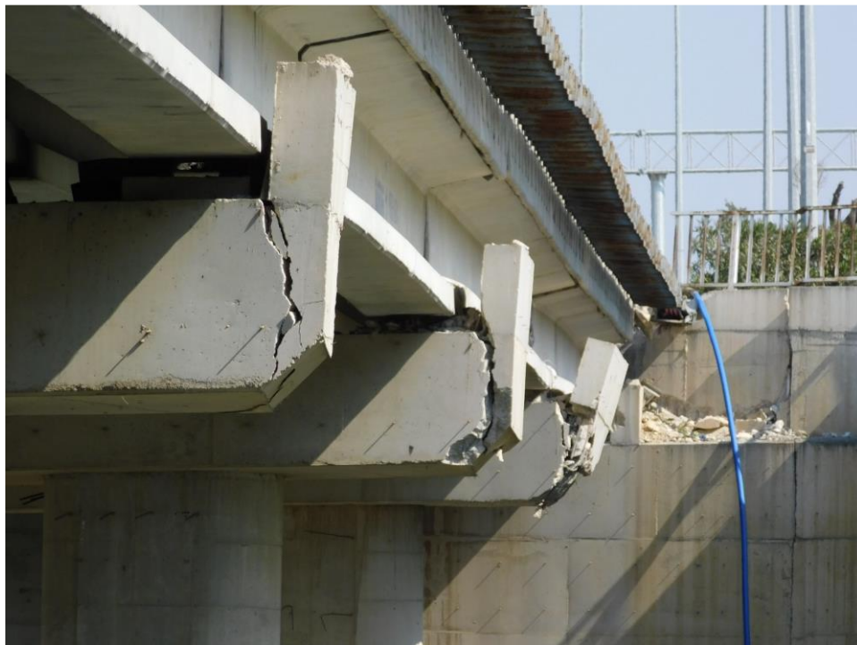
Figure 5-14 Failed exterior shear keys, Bridge 2
