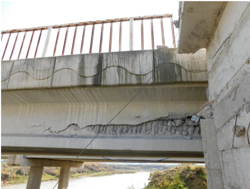
Figure 5-18 Damage to end of precast girder, Bridge 2
