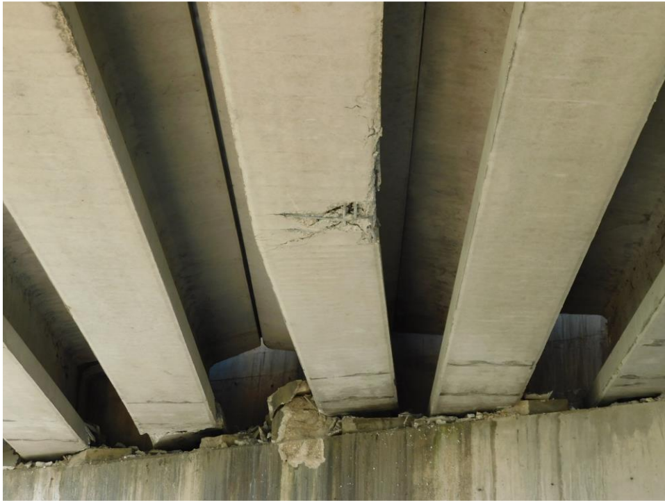
Figure 5-28 Lateral/vertical bending and damage of interior girder at mid-span and shear key damage at girder end, Bridge 2
