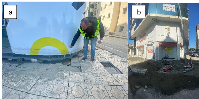
Figure 3-7 Liquefaction manifestation): a) Odeo Bank corner: sand ejecta and liquefaction induced settlements (~36°35'25.92"N/ 36° 10'25.46"E); b) Civilim building corner: sand ejecta (~ 36°35'23.48"N/ 36° 10'23.89"E).
