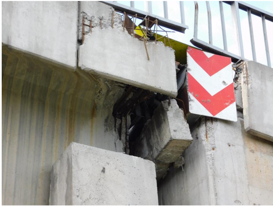
Figure 5-12 Damage at abutment, Bridge 1
