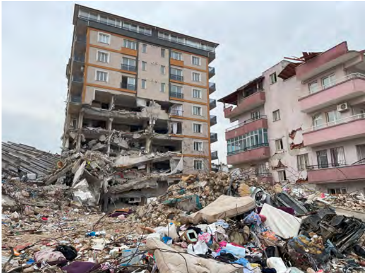
Figure 5.21. Structure impacted by neighboring buildings (pounding effect)
