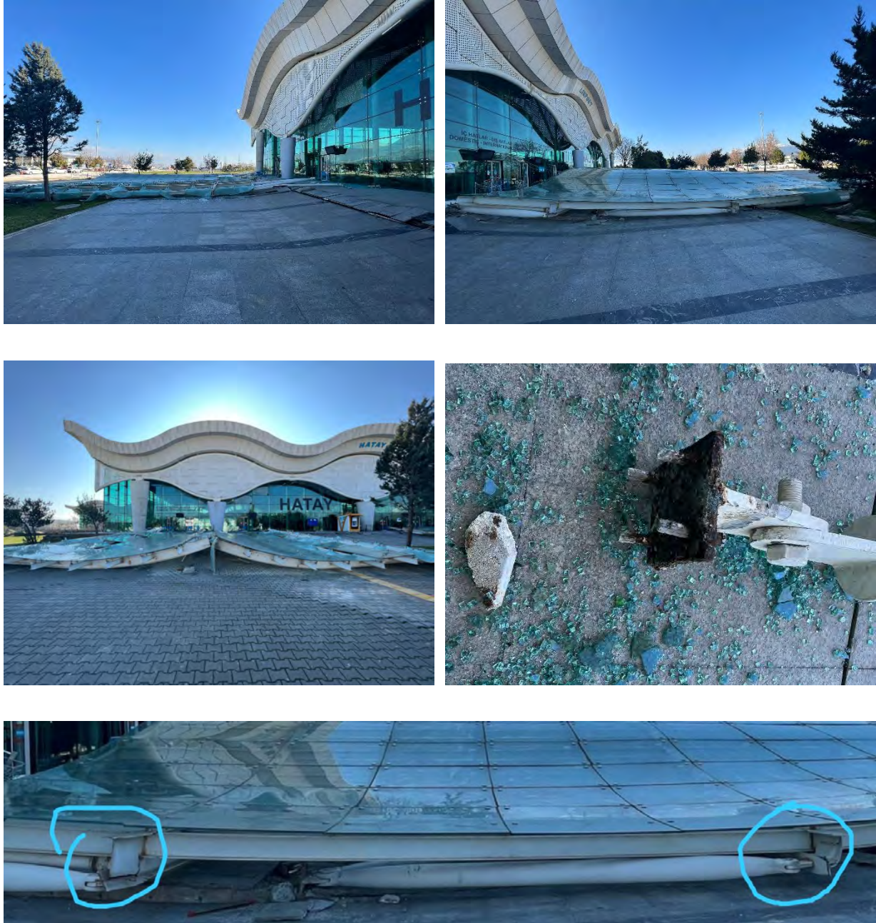
Figure 7.13. Collapsed canopy at entrance to Hatay Airport
