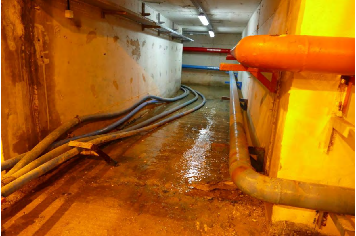
Figure 7.50. Observed water infiltration in below-ground utility tunnels believed by facility operators to be potentially an indication of damage and leaks in below-ground piping infrastructure.
