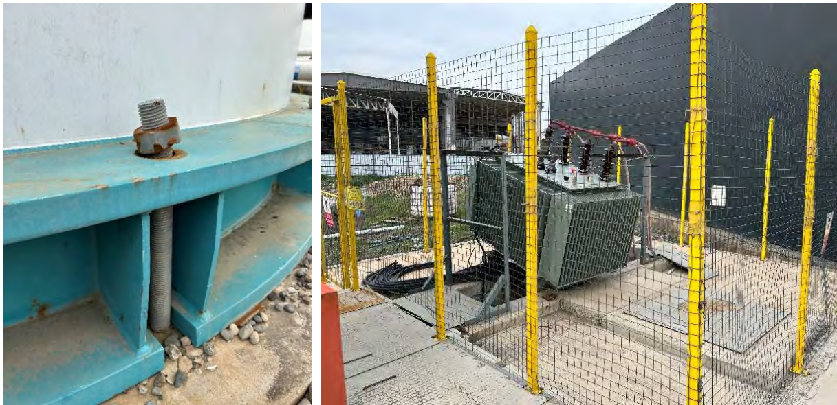
Figure 7.38. Deformed anchors and damaged generator at LPG production facility in Turkoglu (ID 144 in Appendix A).
