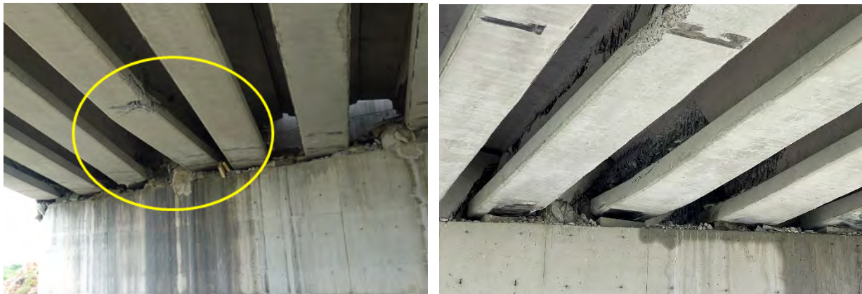
Figure 7.3. Severely damaged concrete bridge girders resulting in reduced load carrying capacity, (ID No. 33 in Appendix A).
