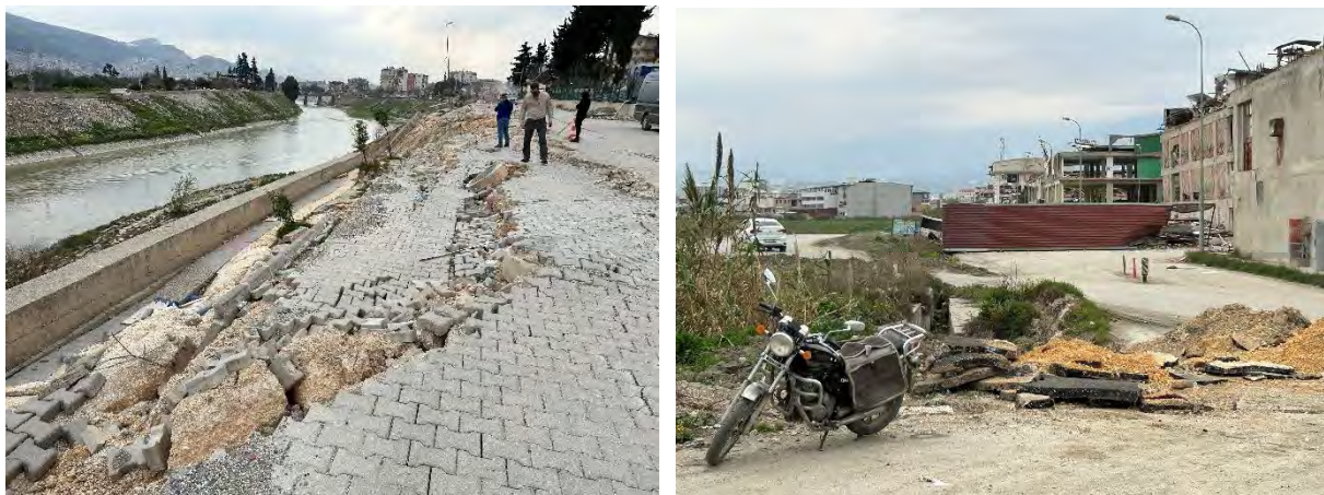
Figure 7.10. Embankment and roadway failure in Antakya (left, ID No. 19 in Appendix A), makeshift road around collapse debris in Antakya (right, near ID 20 in Appendix A).
