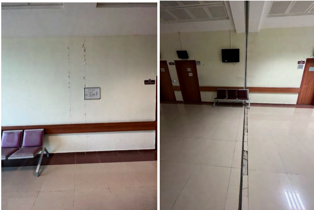
Figure 7.67. Cracking at joint between infill wall and column (left) and cracking of tiles at expansion joint (right)
