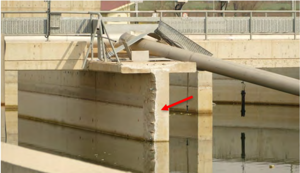
Figure 7.53. Concrete pour joint (arrow) dividing collapsed portion of interior wall (now below water surface) from surviving portion of dividing wall with stiffening walk bridges; no reinforcing provided across joint (Kırıkhan, Hatay) (ID No. 30 in Appendix A).
