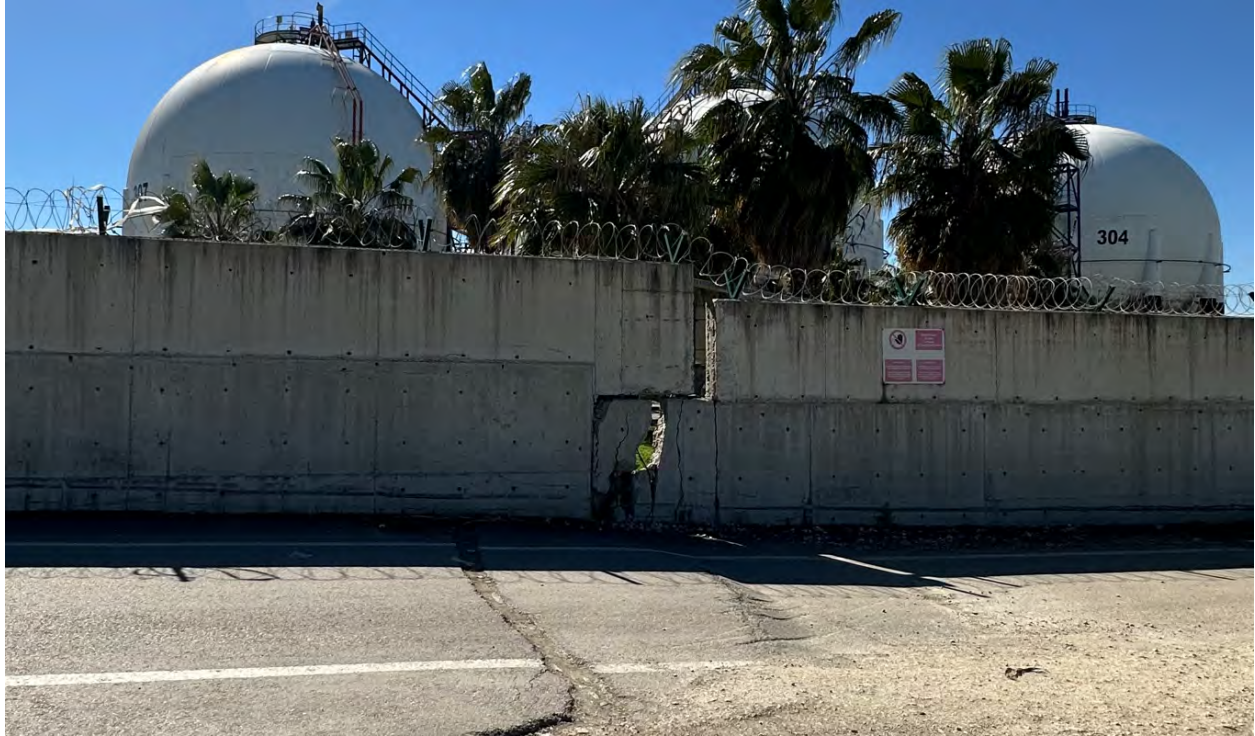
Figure 7.33. Lateral spread causing separation in the boundary walls at one of the LPG terminals due to lateral spreading.
