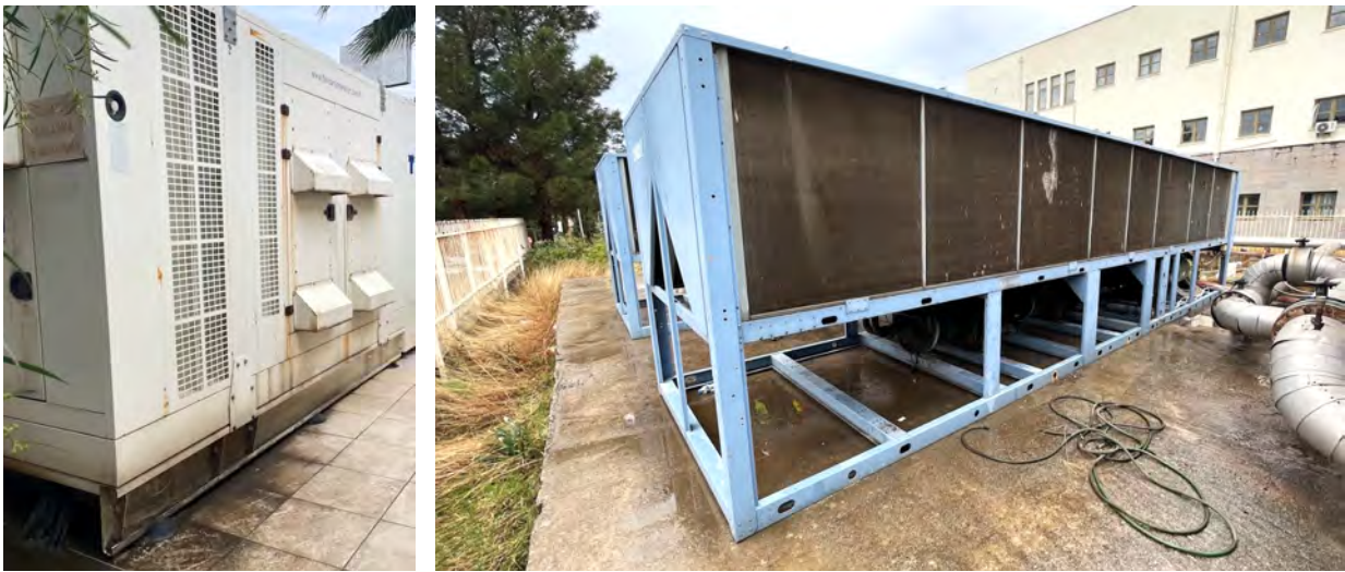
Figure 6.15. Unanchored generator (left) and unanchored chiller (right) in Iskenderun, Hatay province.
