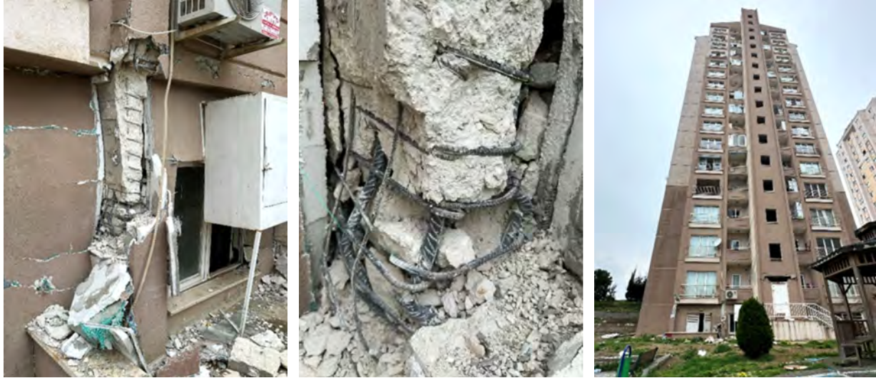
Figure 5.39. Damage in the first story of a tunnel-form shear wall building.
