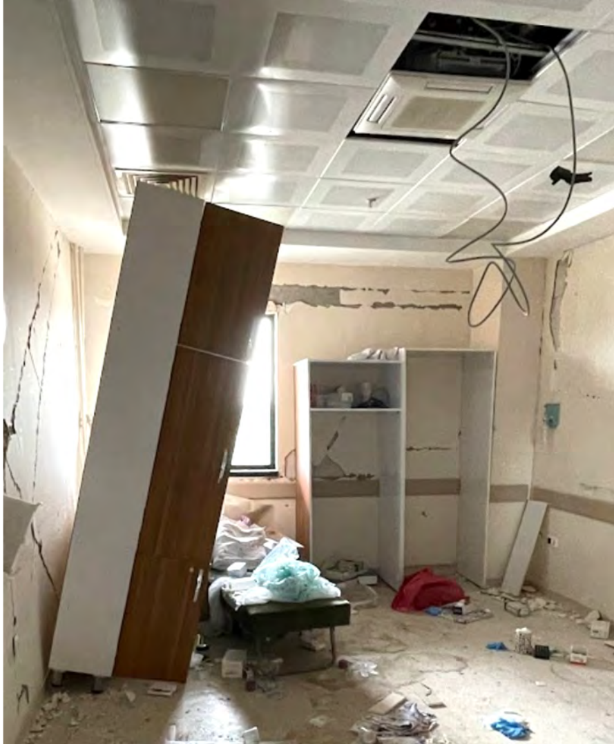
Figure 6.18. Cabinet failure at Nurdağı Government Hospital.
