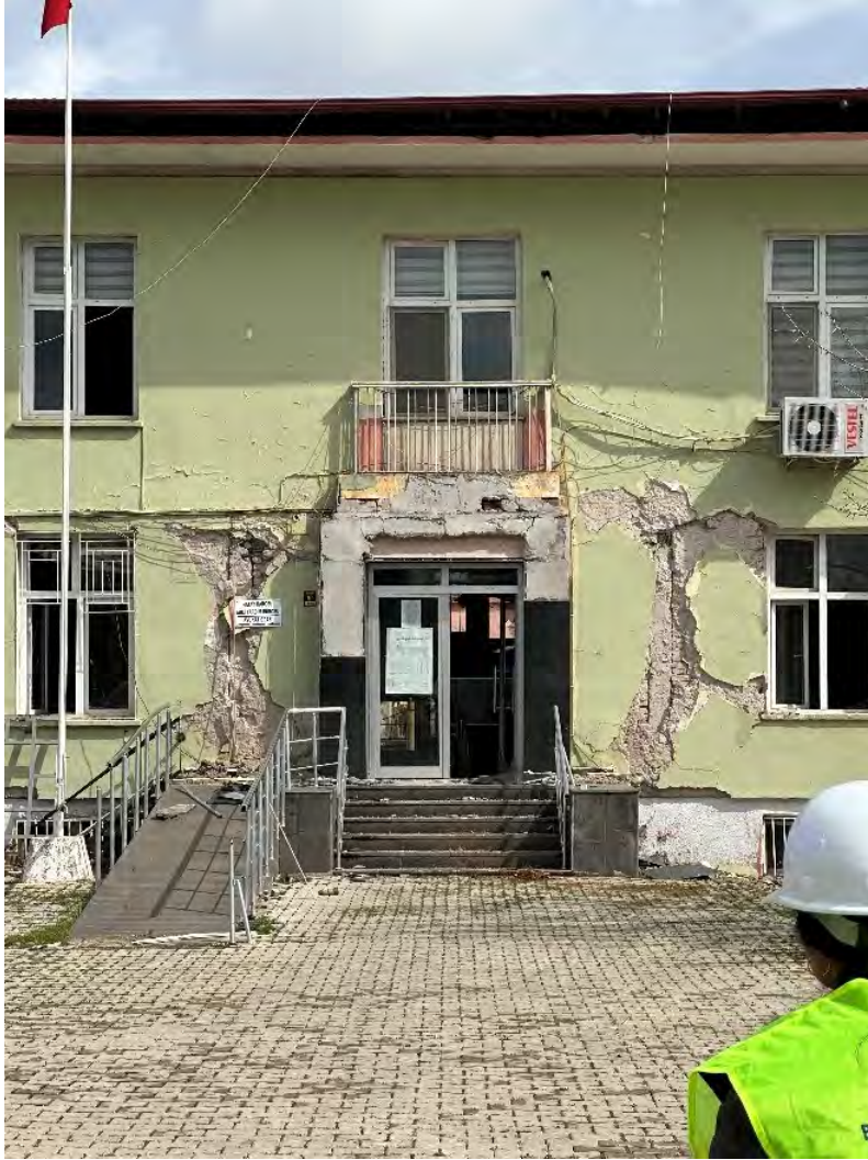
Figure 5.55. Damage to exterior walls of Hasa courthouse.
