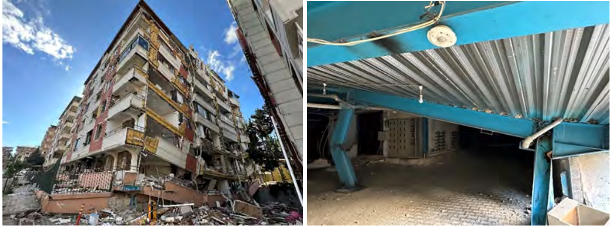
Figure 5.17. Steel-framed structure with failure at the base of the steel columns
