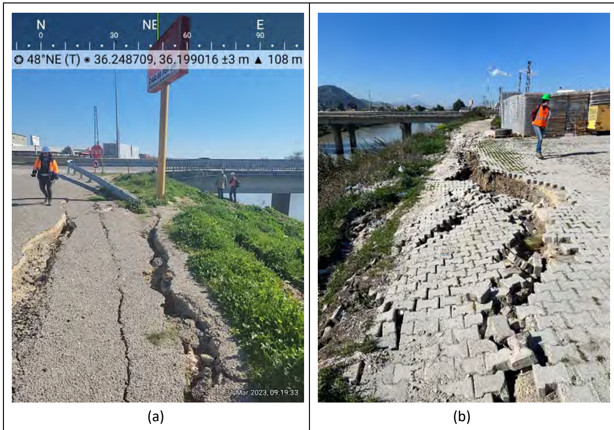
Figure 4.70. Local slope failures along northwest bank near the D817 Bridge: (a) southwest side of bridge with 30 to 40 cm lateral movement and 50 to 60 cm vertical movement (N36.248709°, E36.199016°), (b) northeast side of bridge (N36.249590°, E36.200036°).
