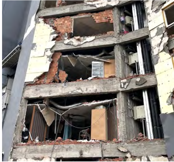
Figure 6.8. Exterior masonry infill wall damage at Megapark Private Hospital as observed on March 13, 2023, PGA = 0.34g, PGV = 51cm/s.
