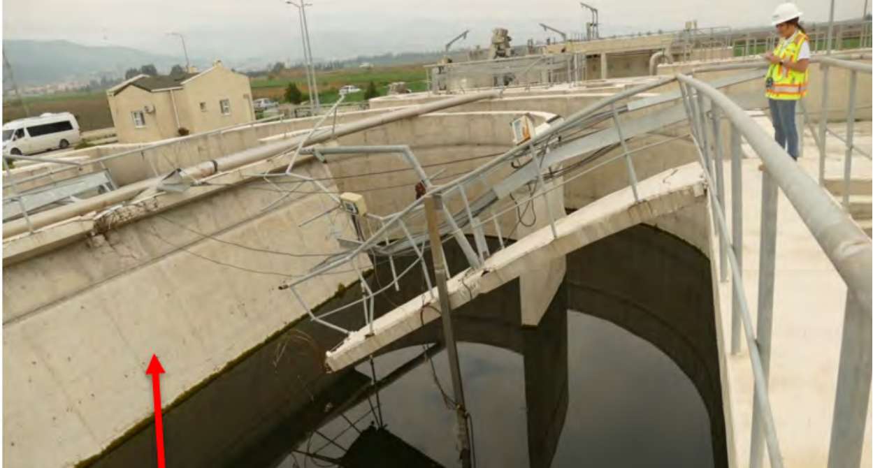
Figure 7.54. Partially collapsed dividing wall (arrow) where stiffening walk bridges existed only on one opposing side at each end of wall. Configuration promoted a torsional response of the dividing wall as bridges pulled out from the dividing wall in tension (Serinyol, Hatay) (ID No. 31 in Appendix A).
