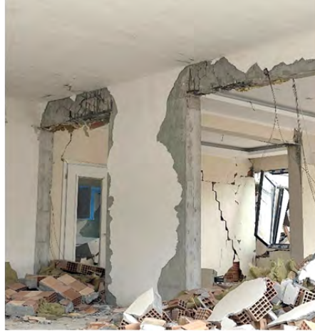
Figure 5.30. Damage distribution along the shorter beam including diagonal cracking.
