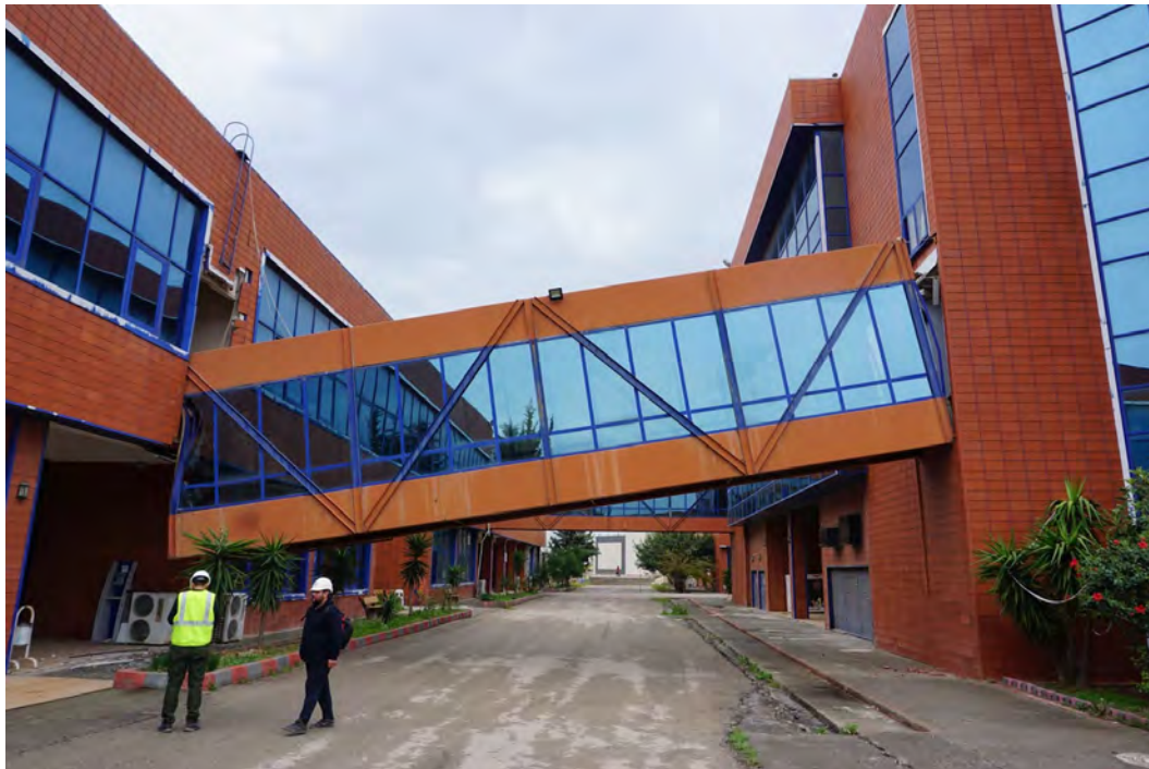
Figure 5.57. Collapse of a sky bridge at Iskenderun Technical University.
