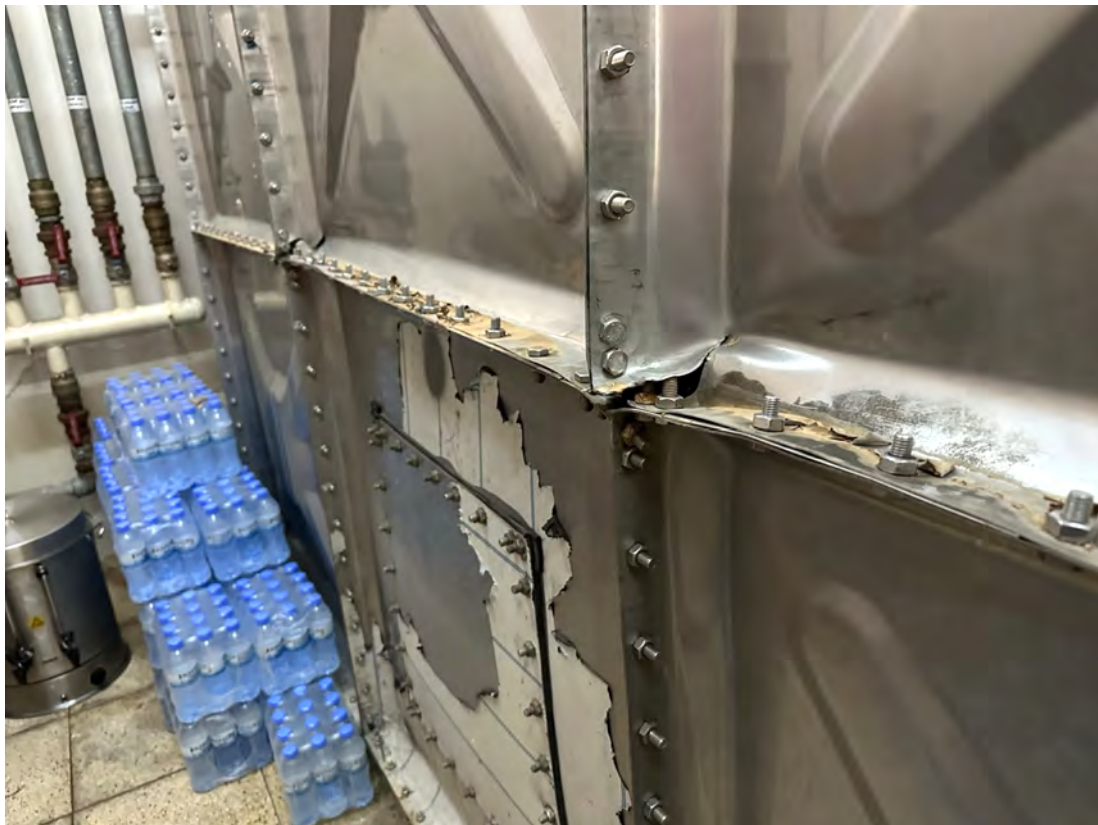
Figure 5.87. Damage to water tank in a school in Kahramanmaraş.
