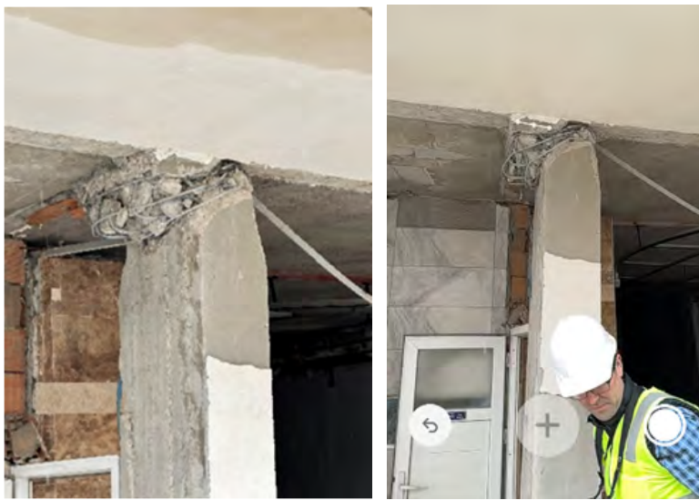
Figure 5.33: Column failure in the weak-axis direction.
