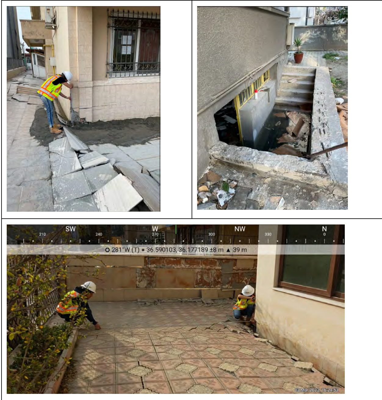
Figure 4.21. (5 images in all) Some four- to five-story buildings located to the northern end of the Atatürk Boulevard near Çay neighborhood experienced liquefaction induced settlement over 60 cm in some locations. Some of the buildings that included a basement experienced less liquefaction-induced settlement but the basement levels were flooded.
