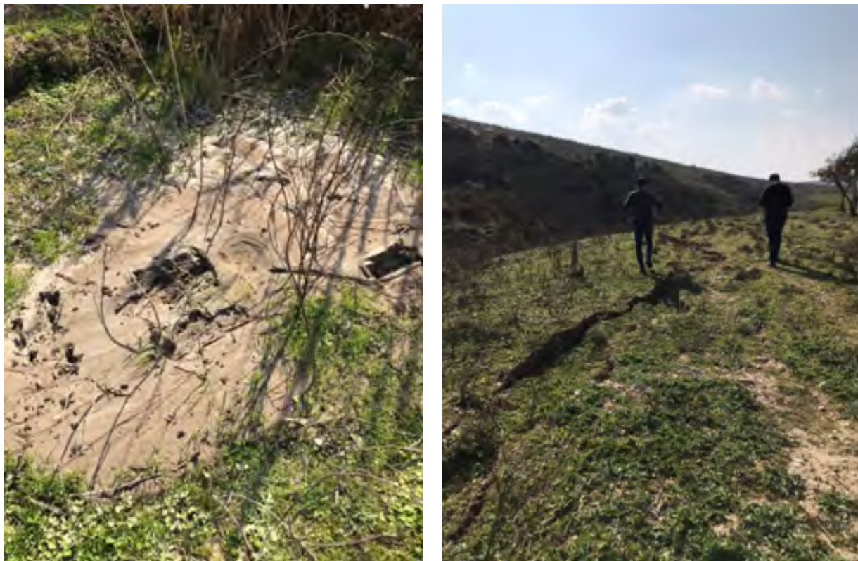
Figure 8.17. Sand boils and liquefaction-induced lateral spreading downstream near the dam body.
