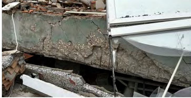
Figure 5.28. Uniformly distributed well-detailed transverse steel in a shear damaged beam in a collapsed building.
