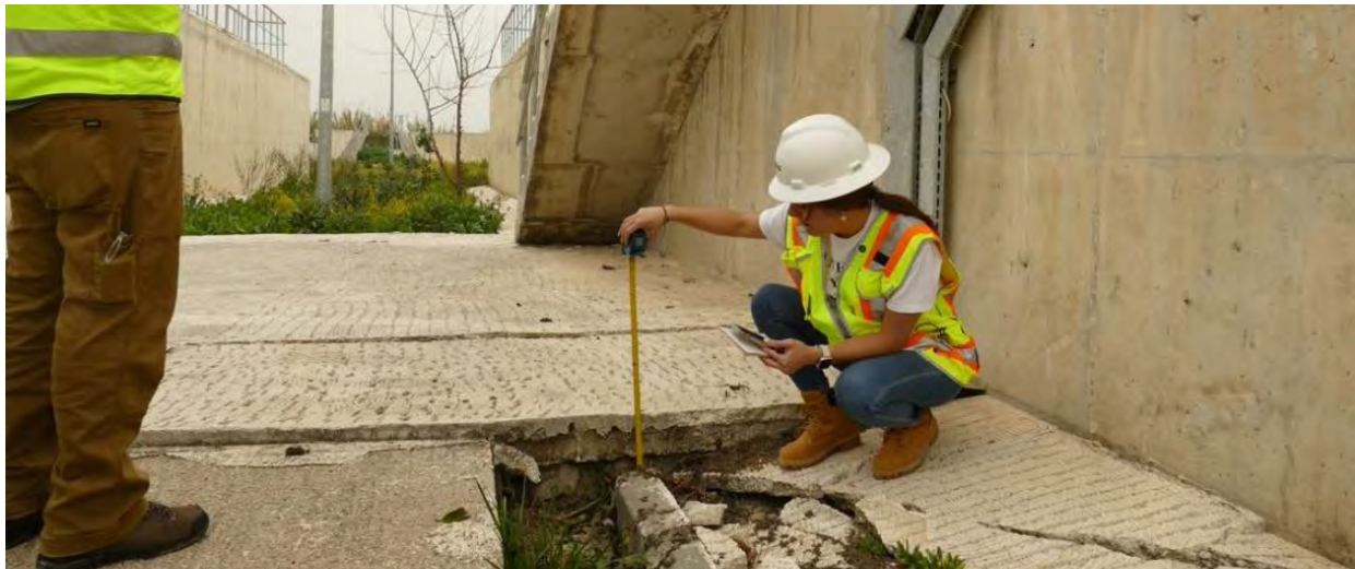
Figure 7.56. Free-field settlements of approximately 16 cm adjacent to tanks structures led to damage and leaks in below-ground piping (Serinyol, Hatay) (ID No. 31 in Appendix A).
