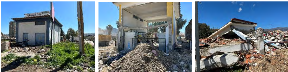
Figure 7.26. Example of range of damage to substation buildings in Antakya.
