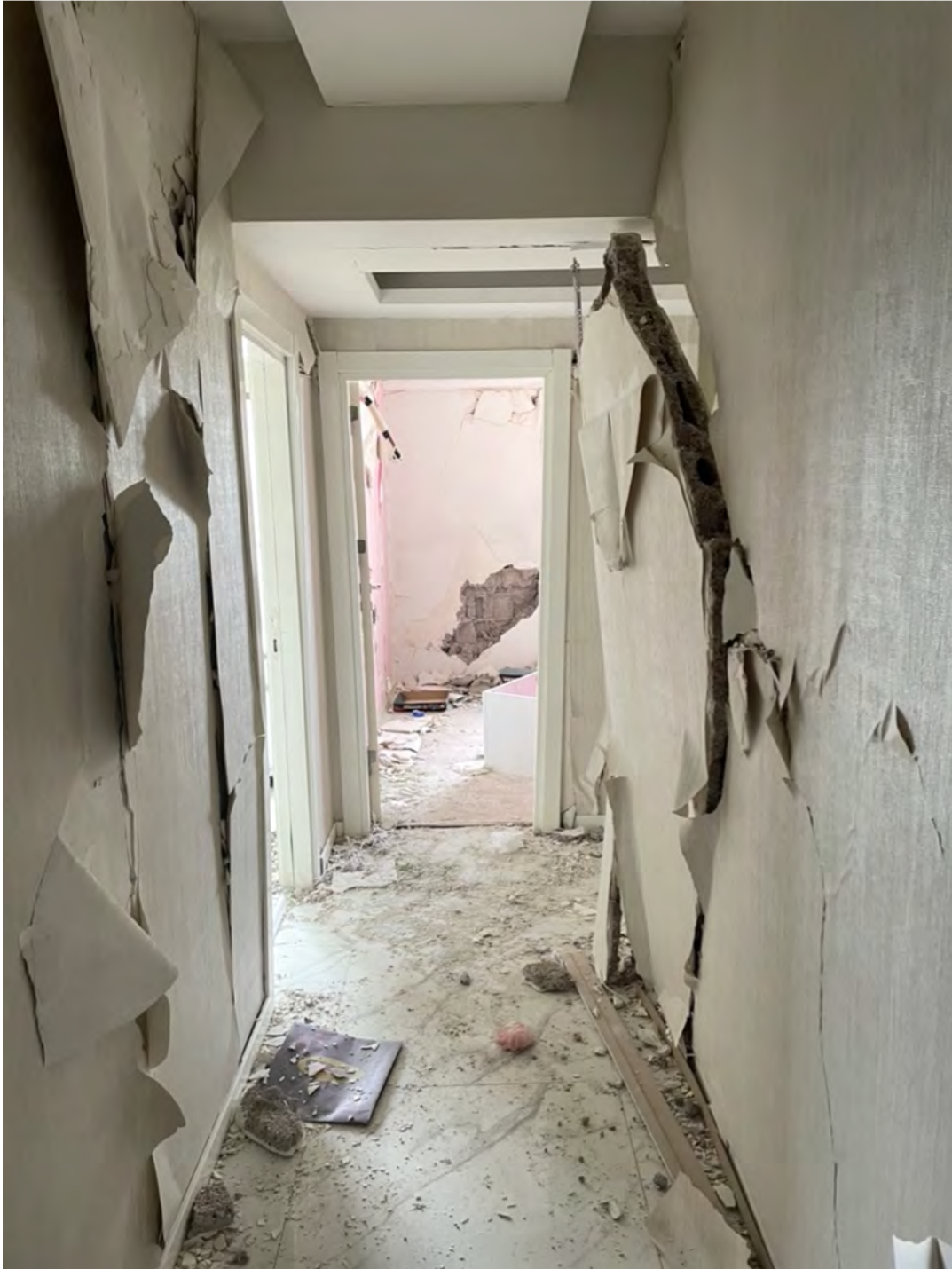
Figure 5.75. Infill partition damage in a residential building near Adiyaman.
