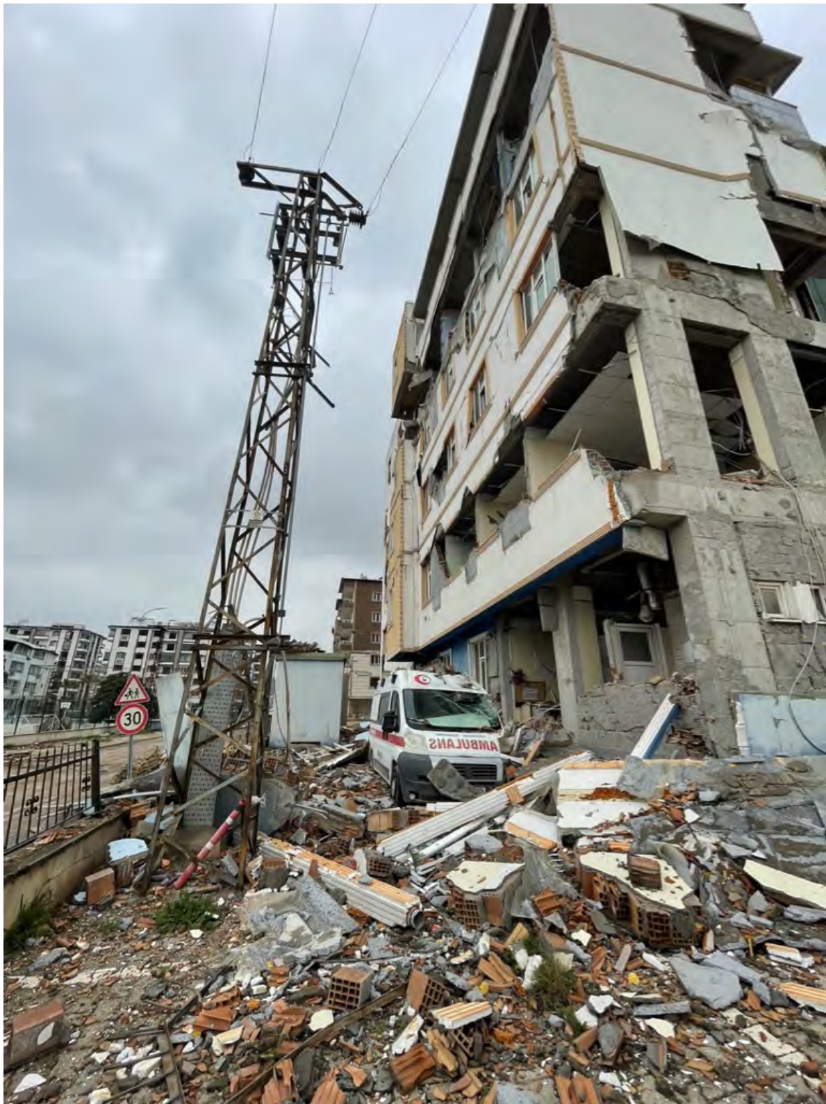
Figure 5.69. Failure of infill facade at a hospital near Kırıkhan that damaged an ambulance and the power feed to the building.
