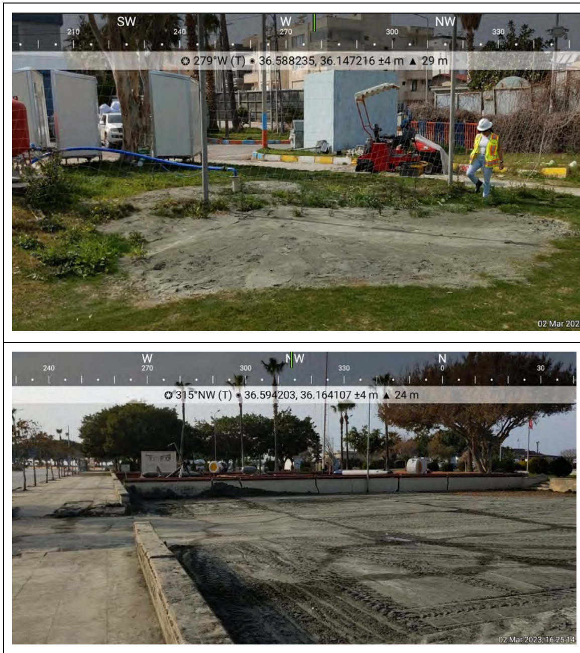
Figure 4.17. Liquefaction ejecta observed along the waterfront park along Atatürk Boulevard. (36.59431, 36.16419)
