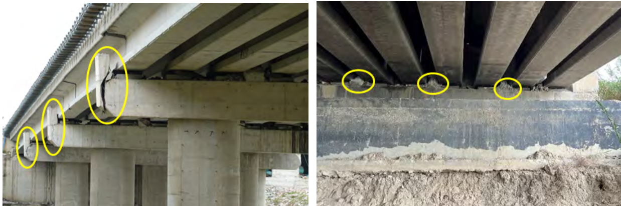
Figure 7.7. Damage to lateral support wings at bents (left) and to shear keys (right).
