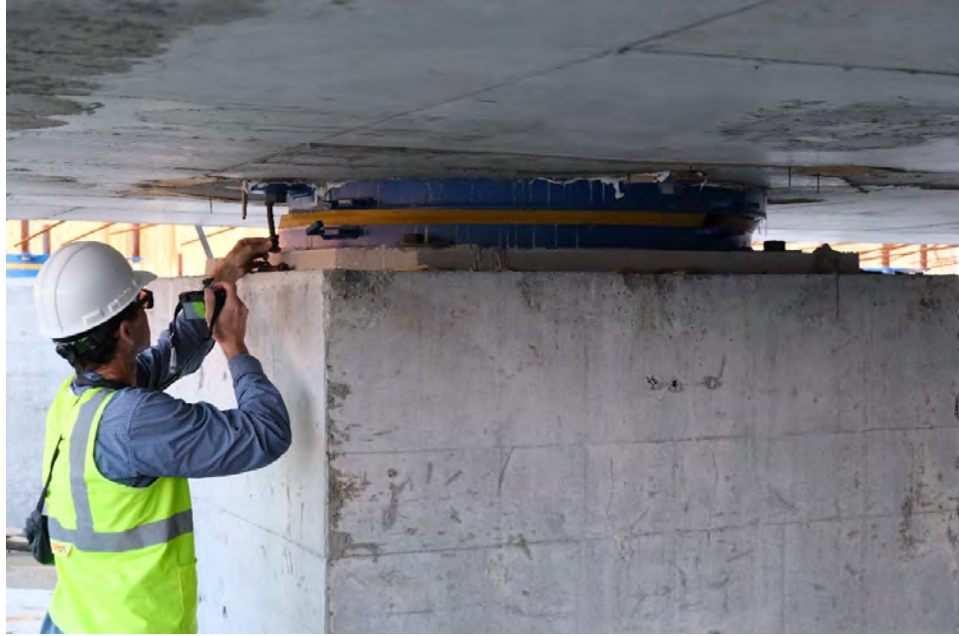
Figure 5.50. Residual displacement of friction pendulum type isolator in Kahramanmaraş. Note that the keeper bolts had not yet been removed and were deformed by the isolator motion.
