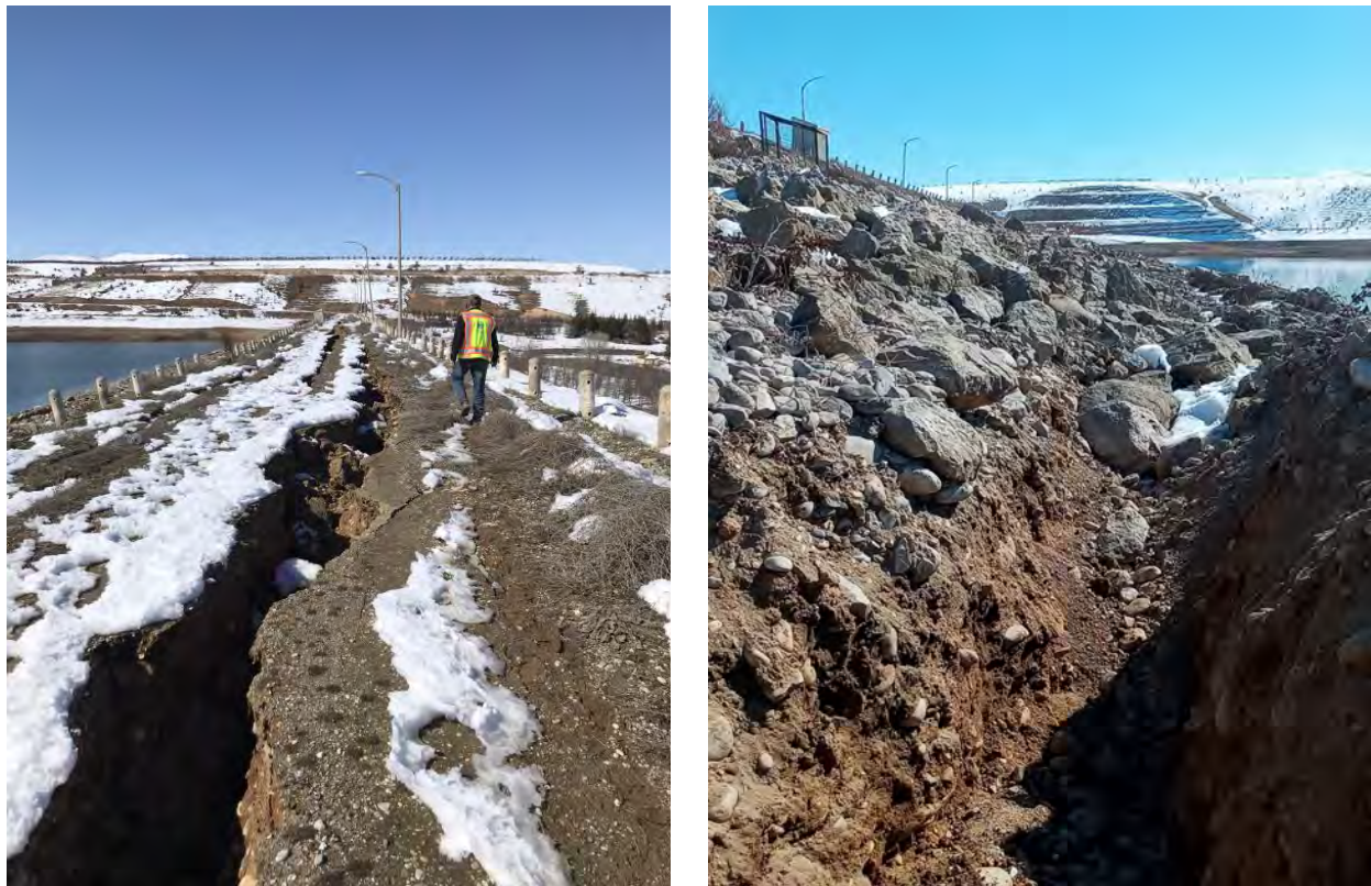
Figure 8.2. Left image shows crest cracking and deformations. Right image shows large face scarps on the upstream face rough half way down the face.
