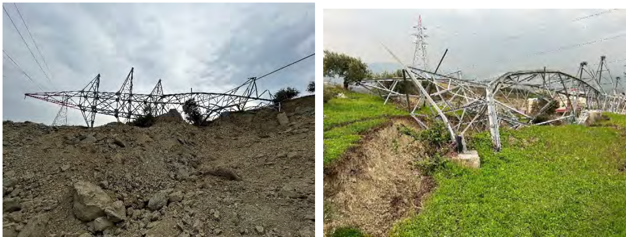
Figure 7.29. Collapsed transmission tower (ID No. 39 in Appendix A).
