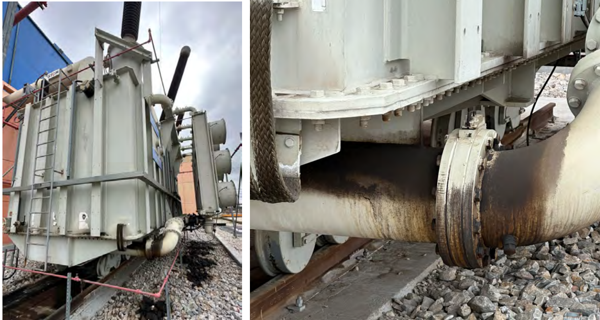
Figure 7.20. Afşin-Elbistan coal plant B transformer with oil leak at flange.
