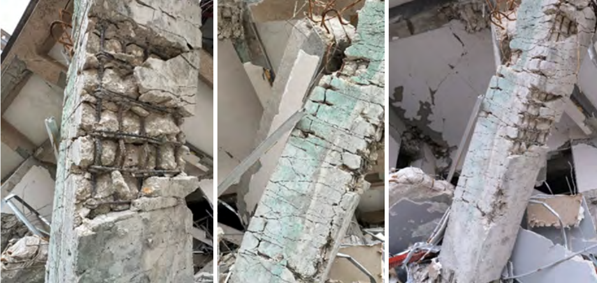
Figure 5.32. Column with overlapping ties experienced uniform cracking along its length.
