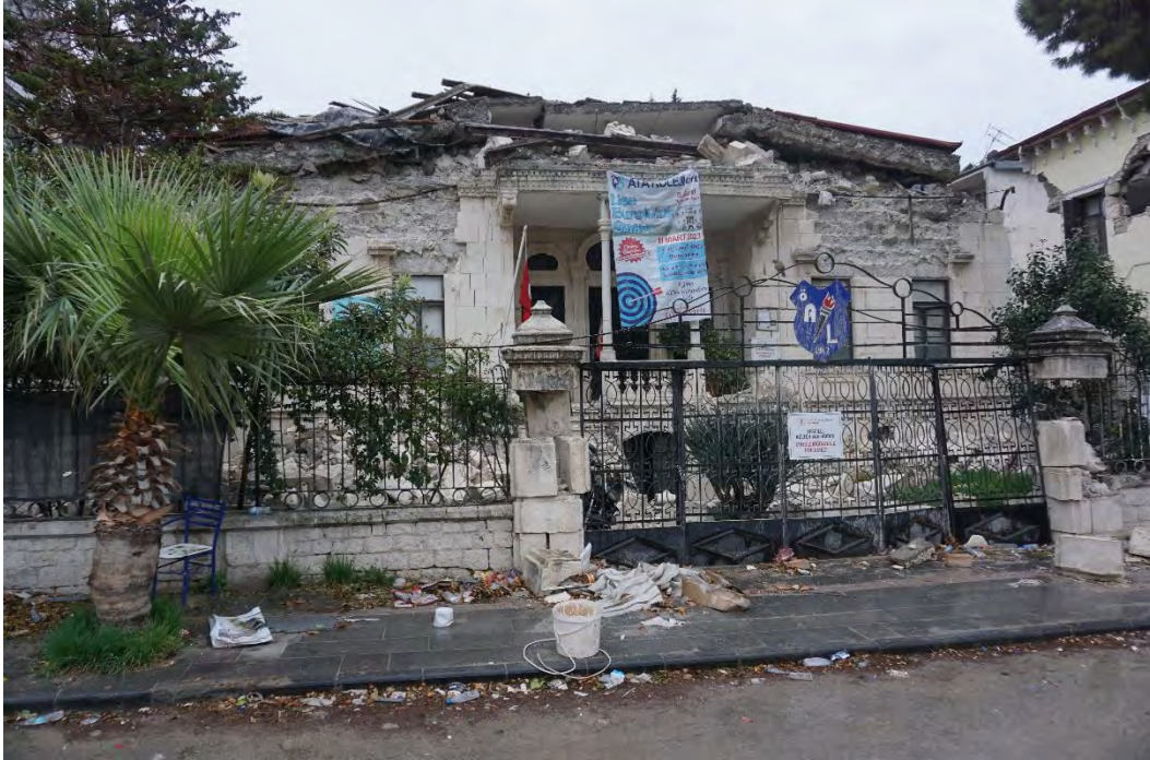
Figure 5.43. Collapse of the second story at a neighboring building.
