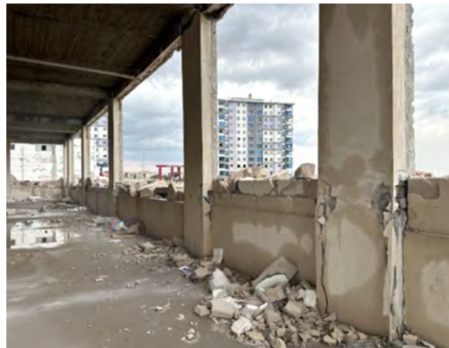
Figure 5.35. Short column effect and damage due to partial height infill walls.
