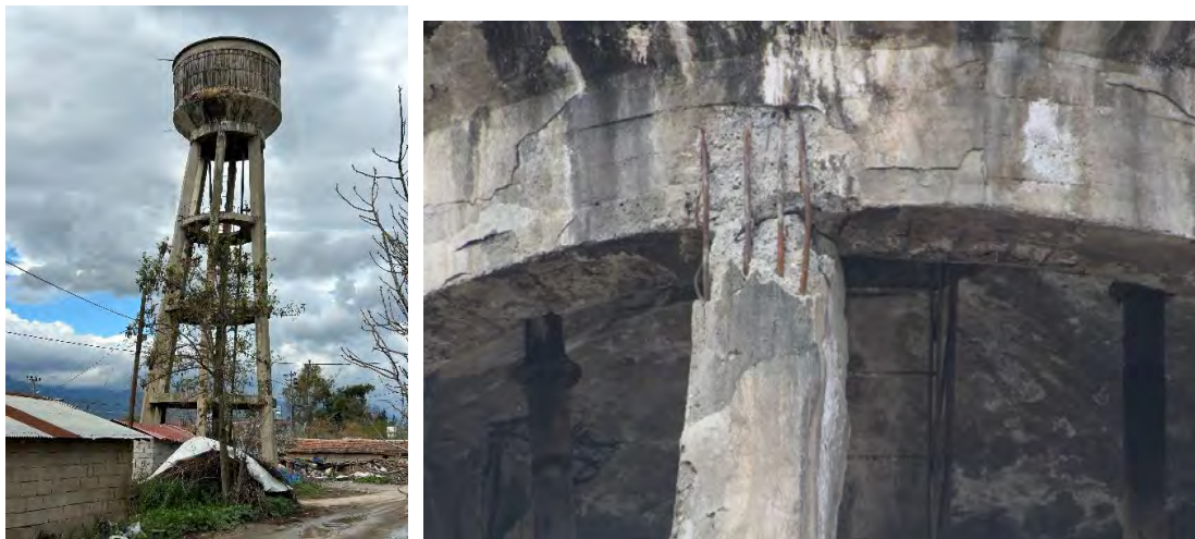
Figure 7.44. Water tower in İçada, Hatay, with significant residual drift and beam-column joint failures, several at joints with no transverse column/joint reinforcement visible (ID No. 100 in Appendix A).
