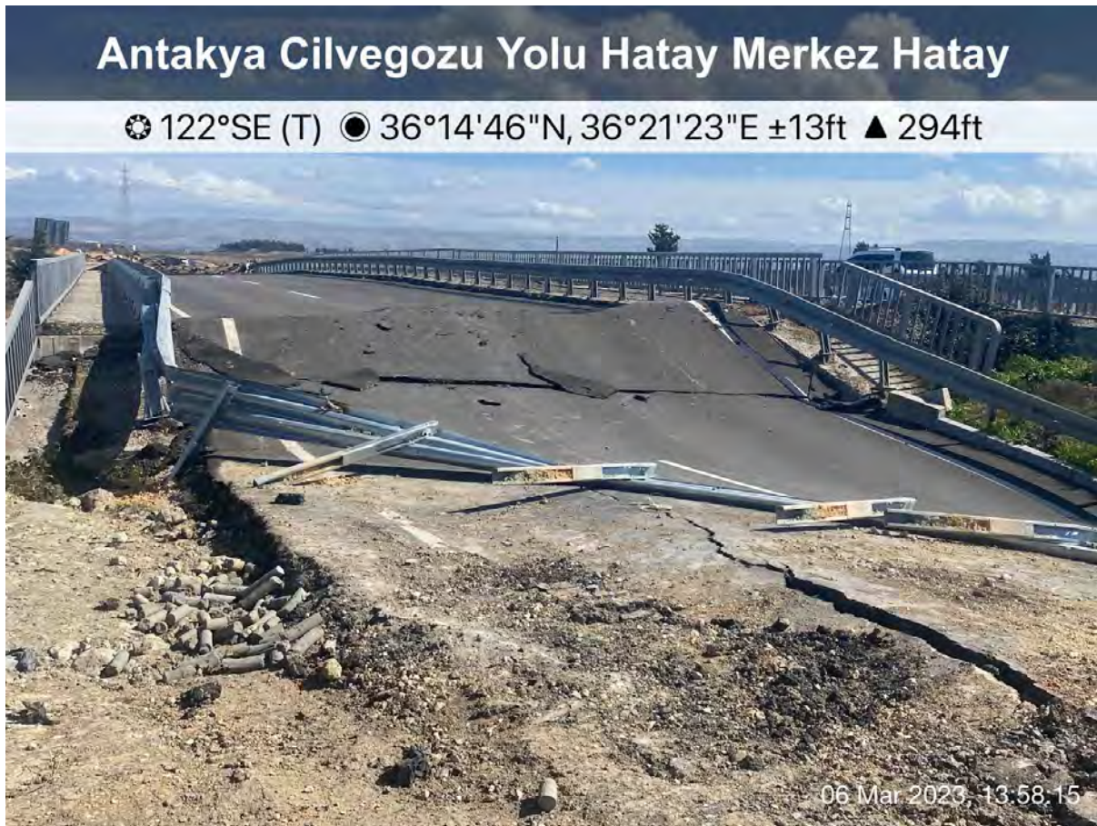
Figure 4.58. Bridge failure across the Orontes River in Demirköprü, Hatay Province on Highway D420.
