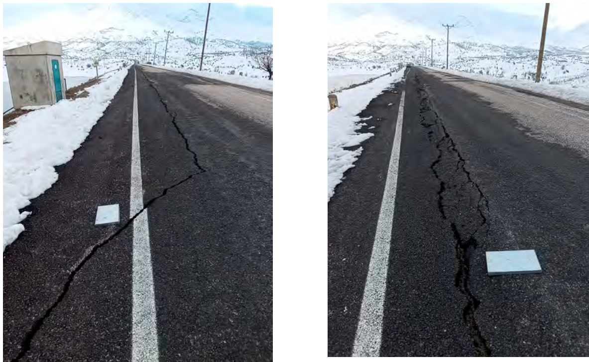
Figure 8.5. Crest cracking observed looking both directions along the crest.
