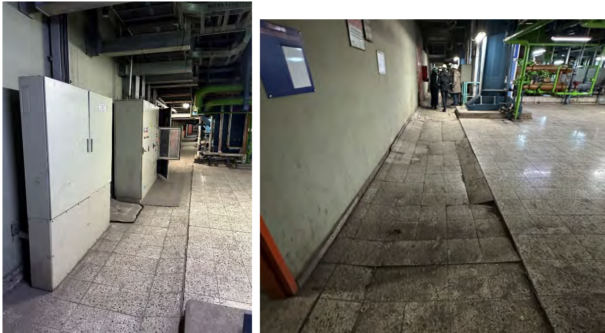
Figure 7.21. Afşin-Elbistan coal plant B – settlement observed in the powerhouse.
