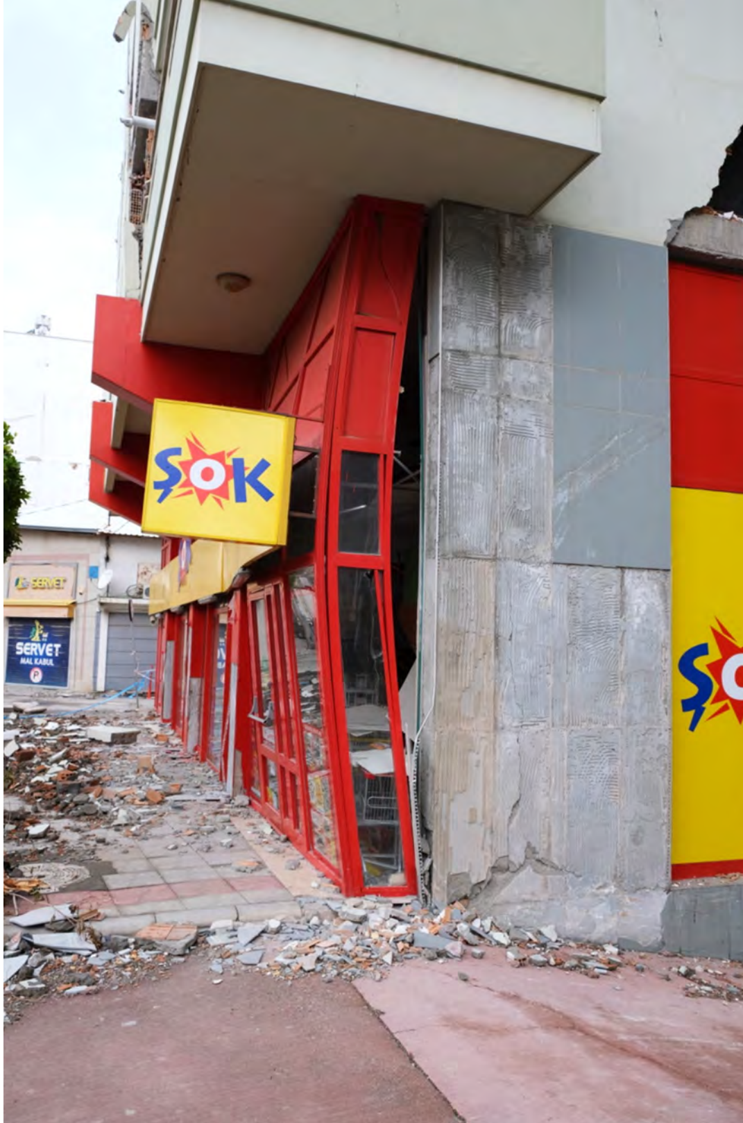
Figure 5.72. Global buckling of metal frame of storefront glazing at ground floor of mixed use building in Iskenderun.
