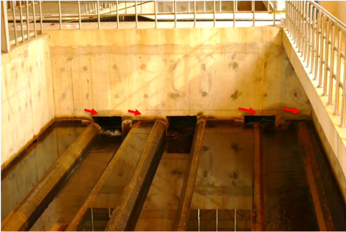
Figure 7.49. Displacement of concrete curbs under inertial forces caused sedimentation channels to leak and be bypassed entirely (arrows indicate displacement of curbs from original position)
