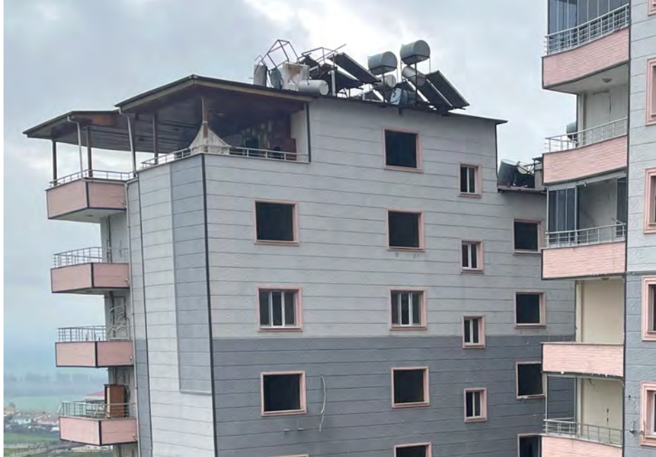
Figure 5.77. Varying levels of damage to rooftop solar water heaters in a residential building near Kırıkhan.
