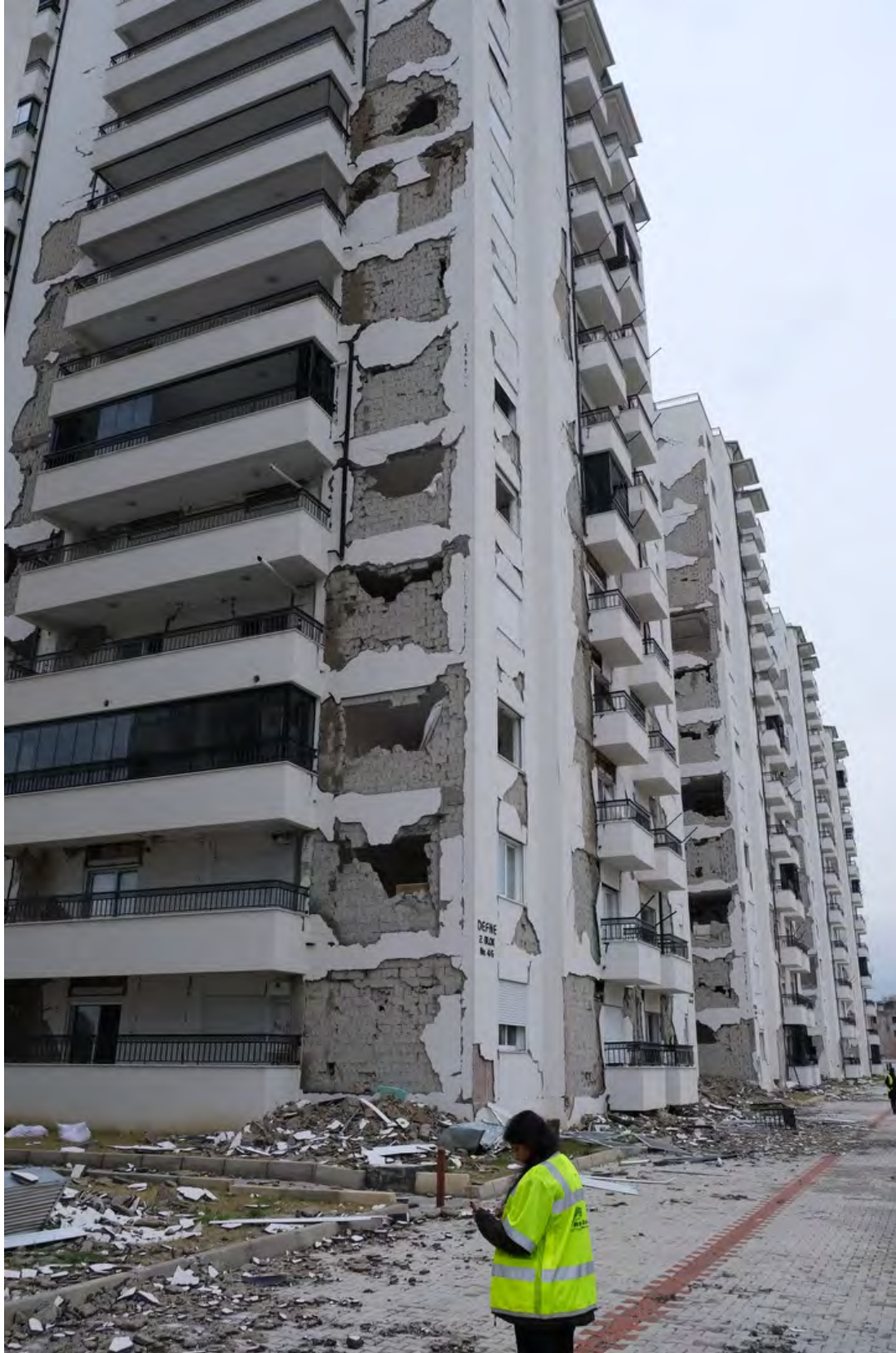
Figure 5.68. Infill facade damage up the height of a residential tower in İskenderun.
