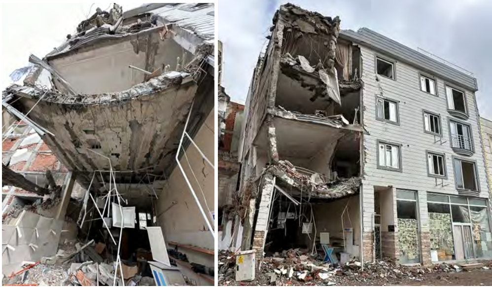
Figure 5.26. Large deformations in filler-joist (asmolen) floor system.
