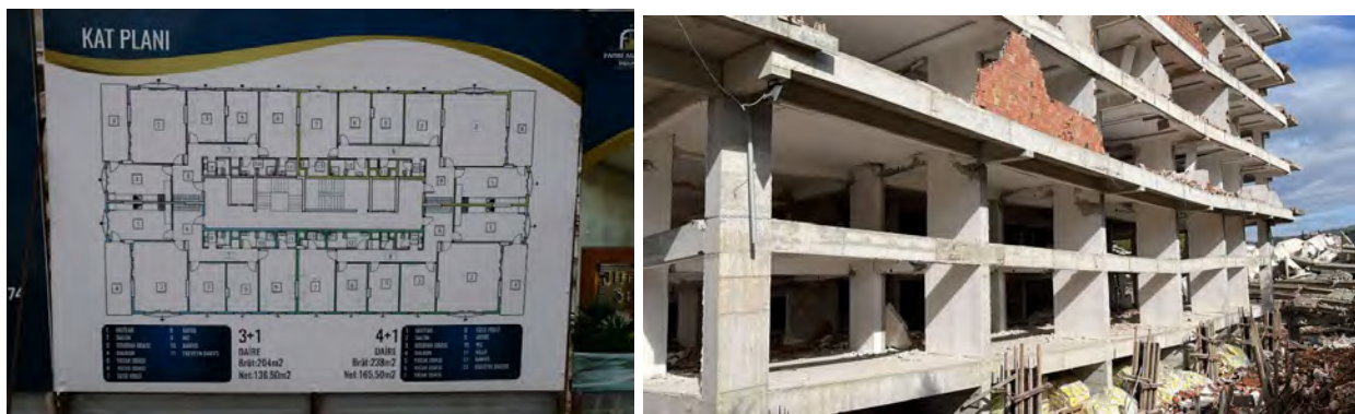
Figure 5.11. RC shear wall frame system building under construction, Antakya (plan on the left; floor plate on the right)
