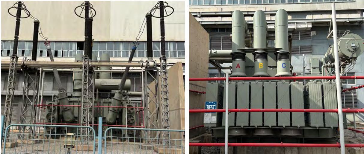
Figure 7.18. İskenderun plant a) example of transformer that sustained broken bushing and b) unanchored transformer that moved 10 cm laterally
