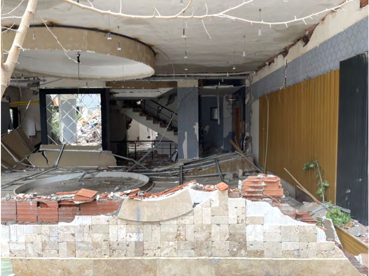
Figure 5.84. Loss of gravity support of suspended ceiling in residential building in Adiyaman.
