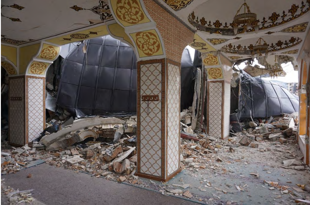
Figure 5.59. Interior of Odabaşı Camii mosque with collapsed dome.
