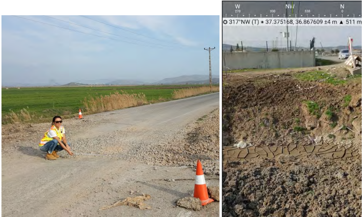
Figure 4.66. a) Observed damage to a 5.7 m-long section of road with a horizontal offset of 3.2 m (37.370574, 36.869232); b) possible ejecta with high fines near a culvert south of Lojistik (37.3752, 36.8676). Photos taken March 4, 2023.
