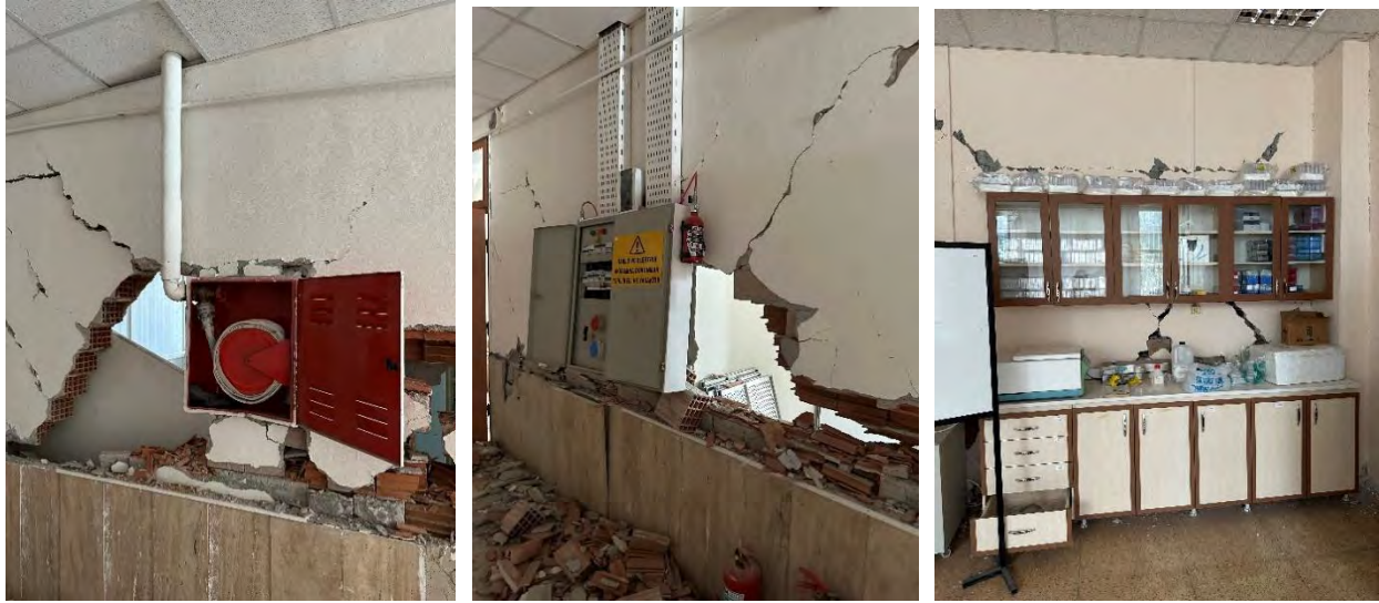
Figure 7.62. Example of equipment surviving masonry infill damage at the Agricultural Science building
