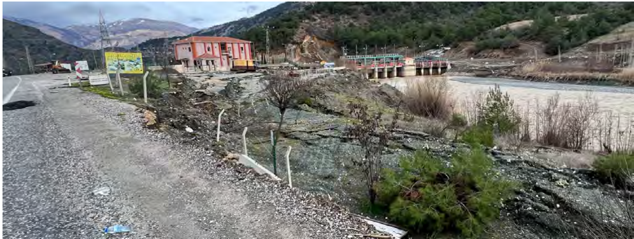
Figure 7.25. River bank failures at Alabalik dam.
