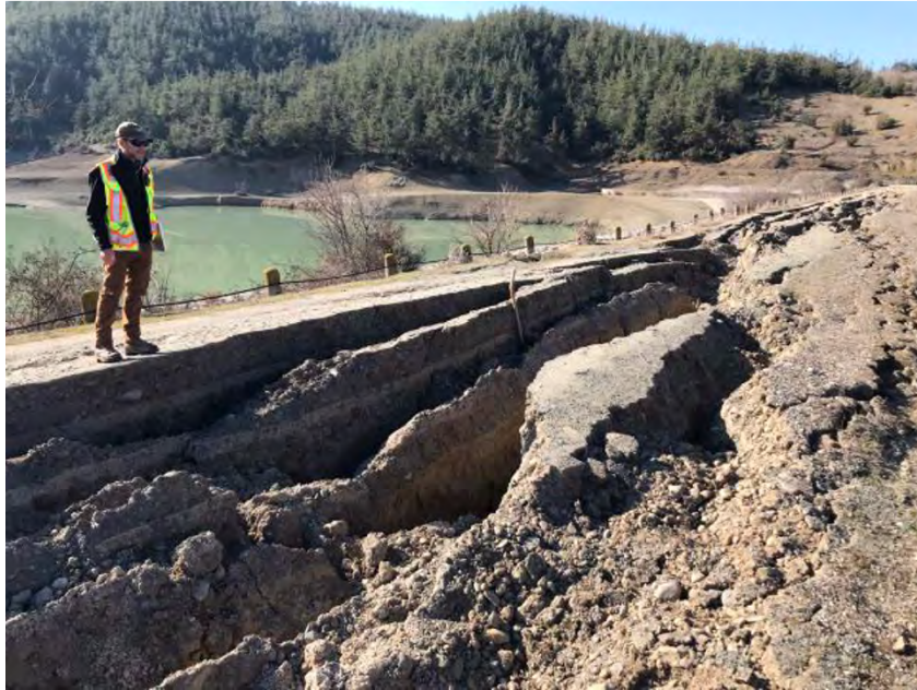
Figure 8.11. Significant crest cracking on Arıklıkış Pond earth dam.
