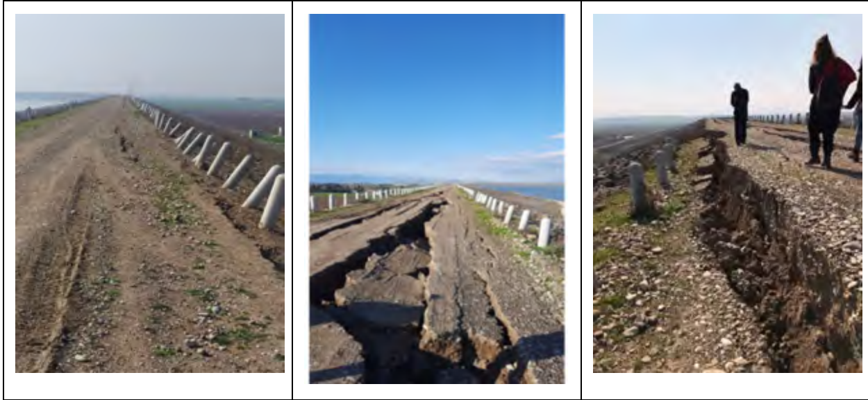
Figure 8.19. Deformations reported on the crest of the Reyhanlı Dam
