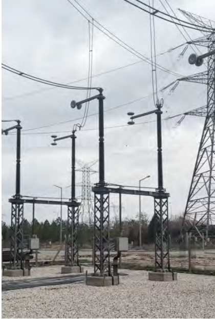
Figure 7.19. Afşin-Elbistan coal plant B switchyard equipment.
