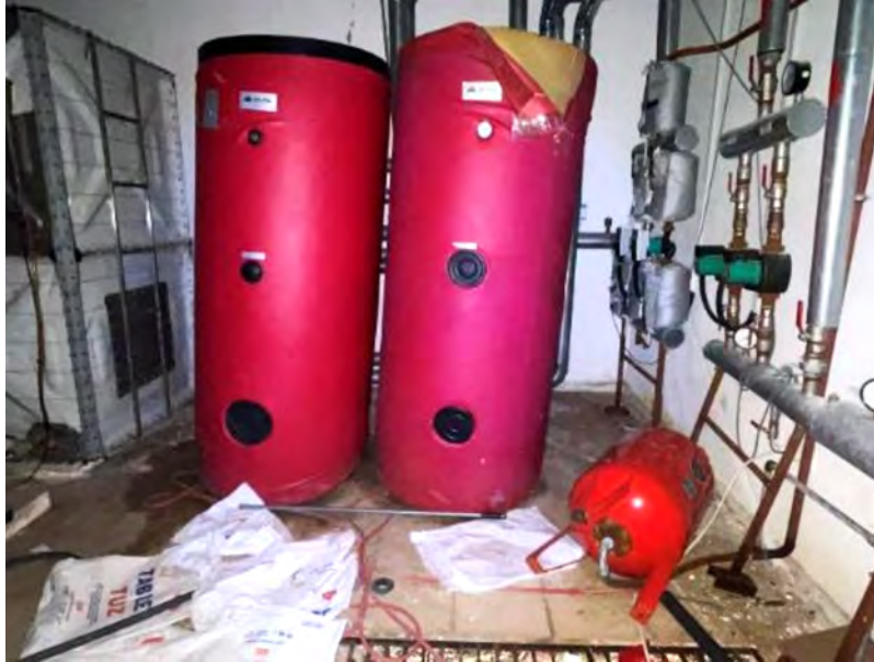
Figure 6.16. Toppled tanks in Nurdağı Government Hospital .
