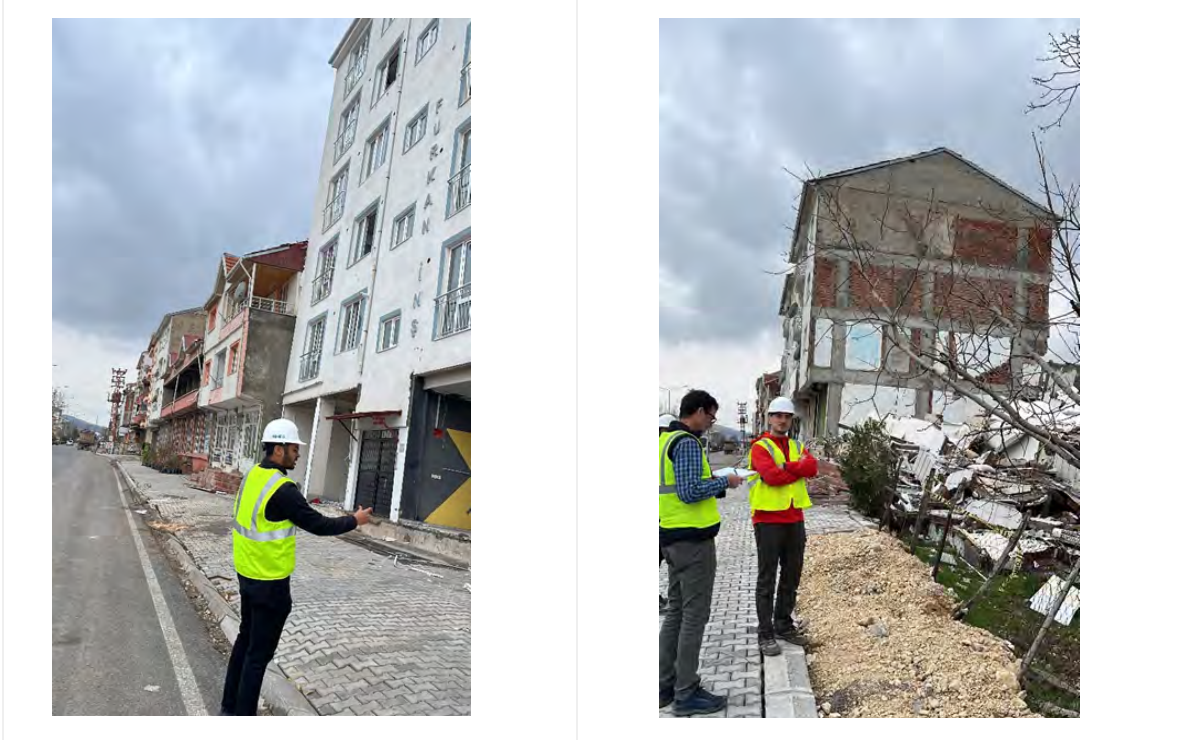
Figure 5.23. Permanent tilt in the structure due to liquefaction.
