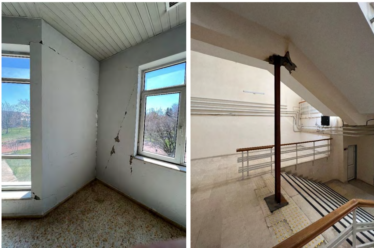
Figure 7.66. Cracking of infill wall in canteen (left) and spalling of underside of stair and steel shoring post in library (right).
