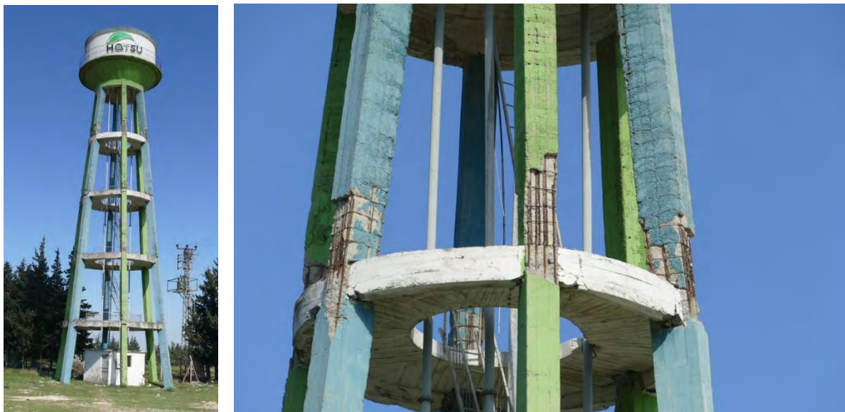
Figure 7.45. Water tower in Antakya with lesser residual drift and extensive cover spalling of concrete columns above upper ring beam levels (ID No. 109 in Appendix A).
