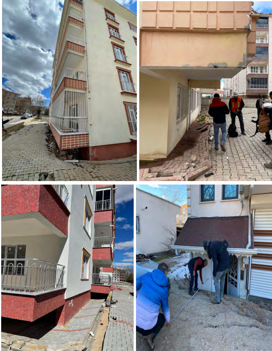
Figure 4.8. Buildings with uniform settlements in the Gölbaşı area (37.78686 N, 37.63738 E).
