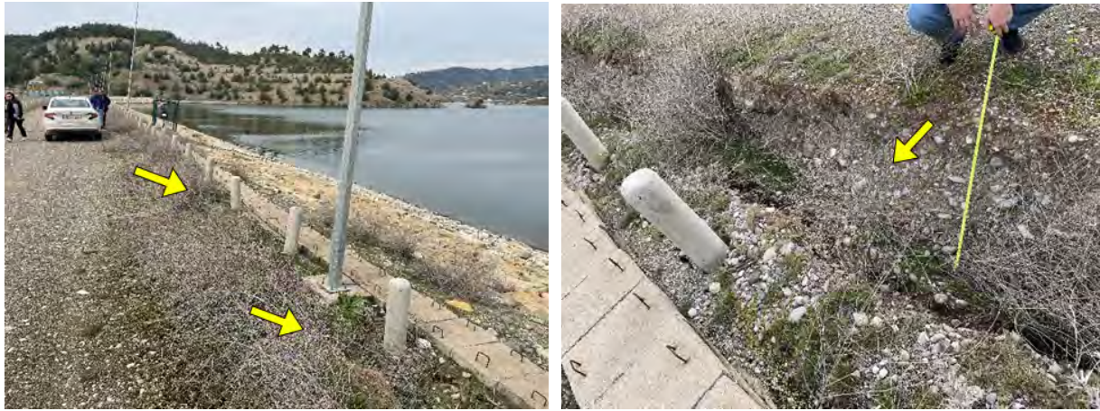
Figure 7.23. Lateral spreading of dam crest at Kilavuzlu dam.
