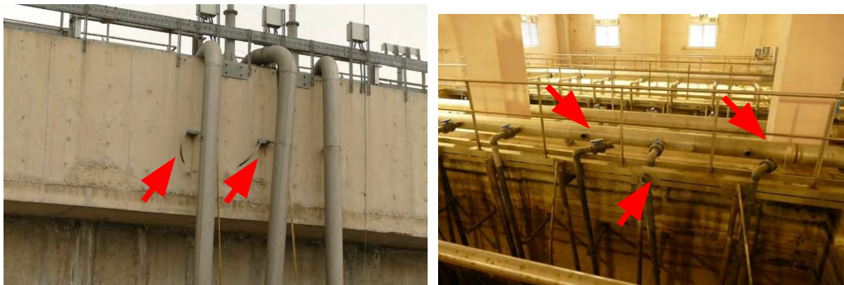
Figure 7.57. (a) Displaced large-diameter vertical pipes with fractured strap bracing (arrows). (b) Fractured vertical, plastic pipes (arrows) with long unbraced lengths (Narlica, Hatay) (ID No. 34 in Appendix A).
