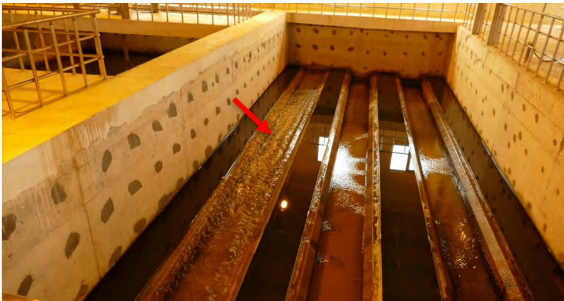
Figure 7.48. Sedimentation channel weirs rendered ineffective due to differential seismic settlements. Arrow indicates area of rapid flow (more settlement) with adjacent channels nearly stagnant (less settlement).
