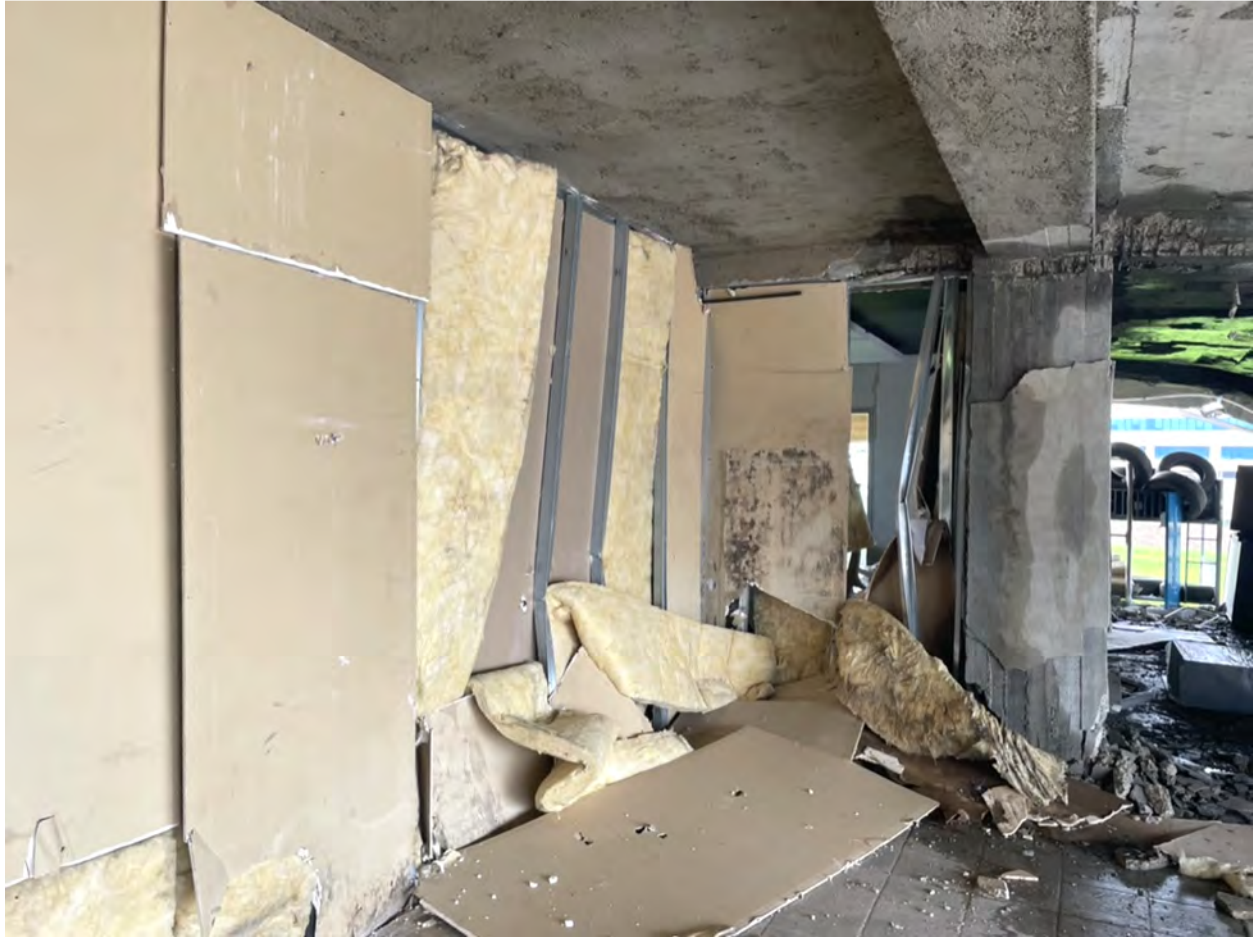
Figure 5.76. Damage to steel frame partitions with drywall sheathing in commercial building in Kahramanmaraş.
