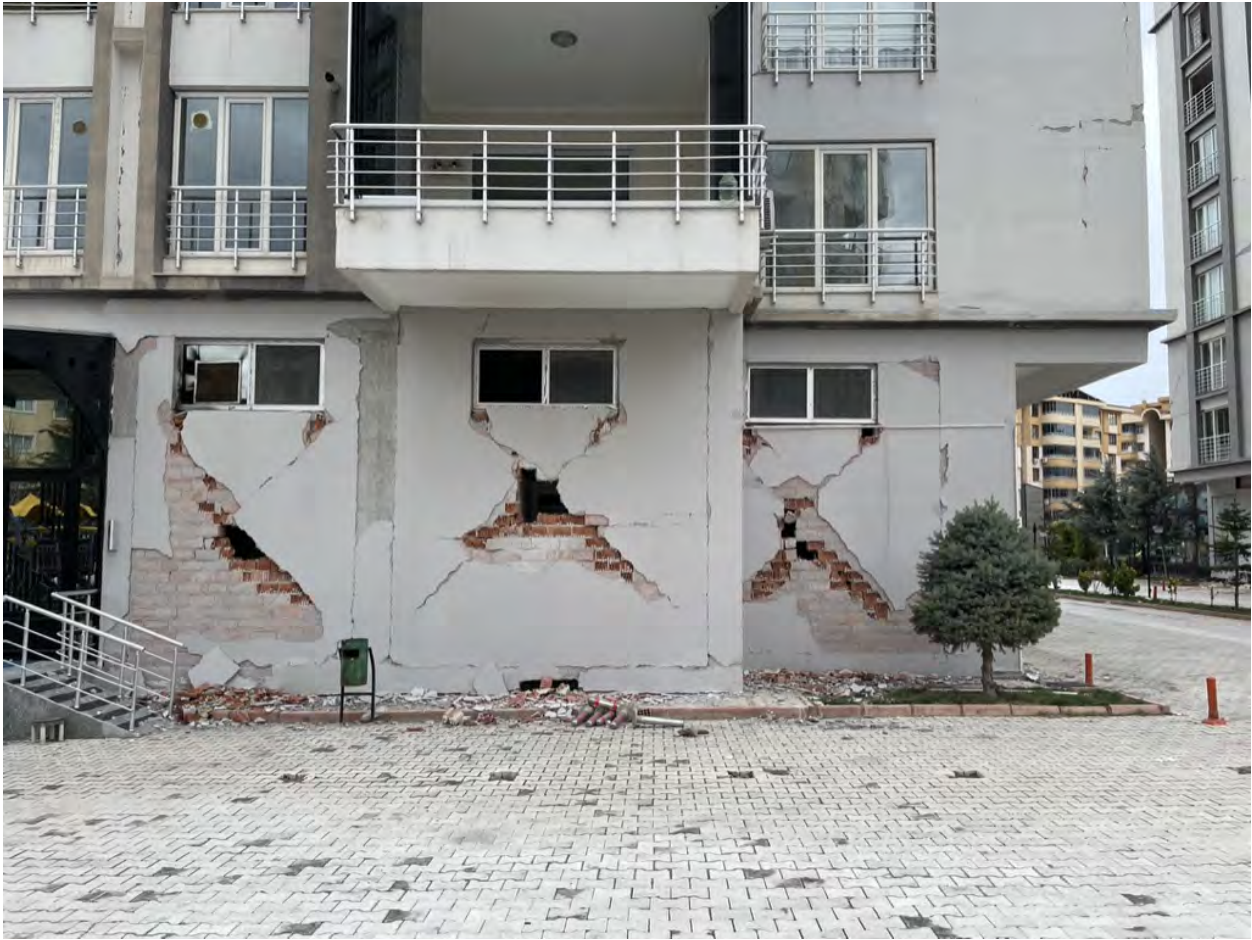
Figure 5.66. Shear cracking in infill partitions at ground floor of residential building in Malatya.
