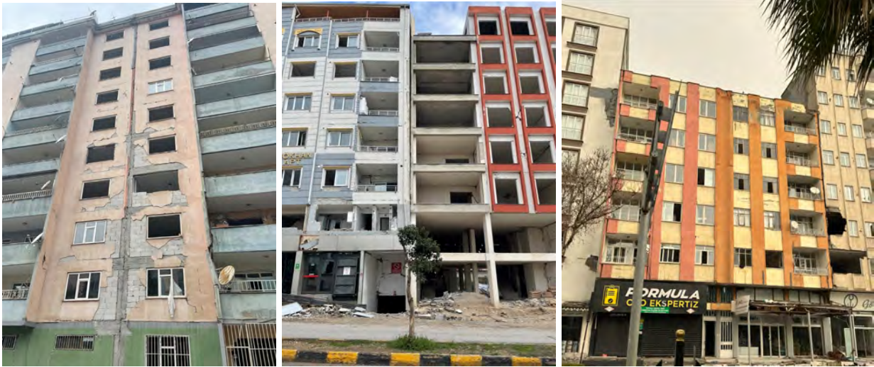
Figure 5.20. Insufficient separation in seismic joints between buildings
