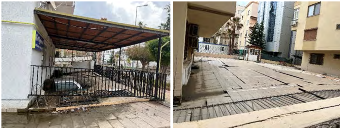
Figure 5.24. Settlement in the structure due to liquefaction.
