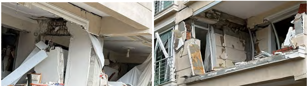
Figure 5.19. Significant structural damage to cantilever beams and coupling beams
