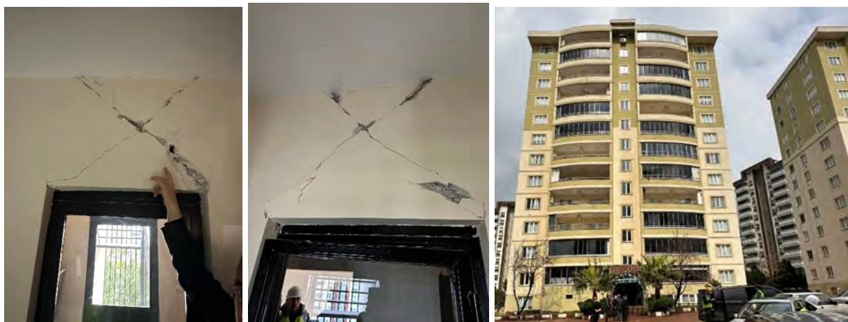
Figure 5.29. Diagonal cracks in beams connecting shear walls in a building constructed using tunnel forms .
