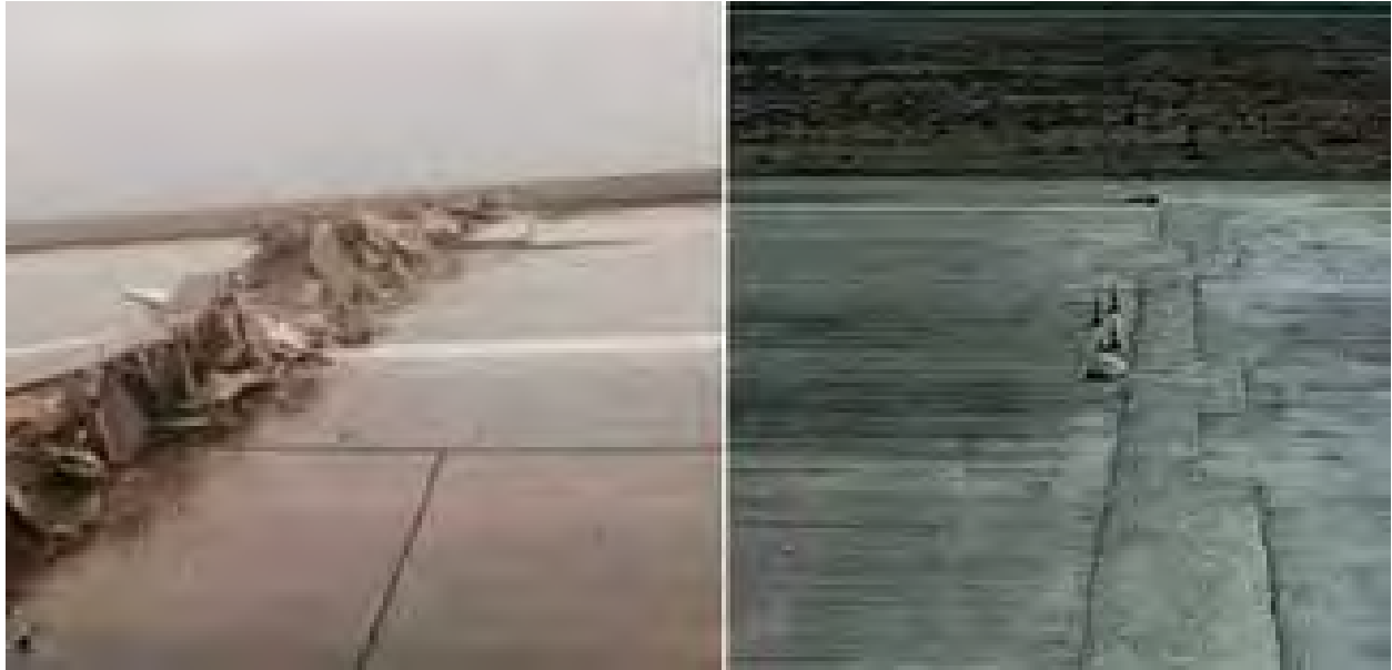
Figure 7.11. Condition of Hatay airport runway after earthquake sequence (left) and after repairs (right)
