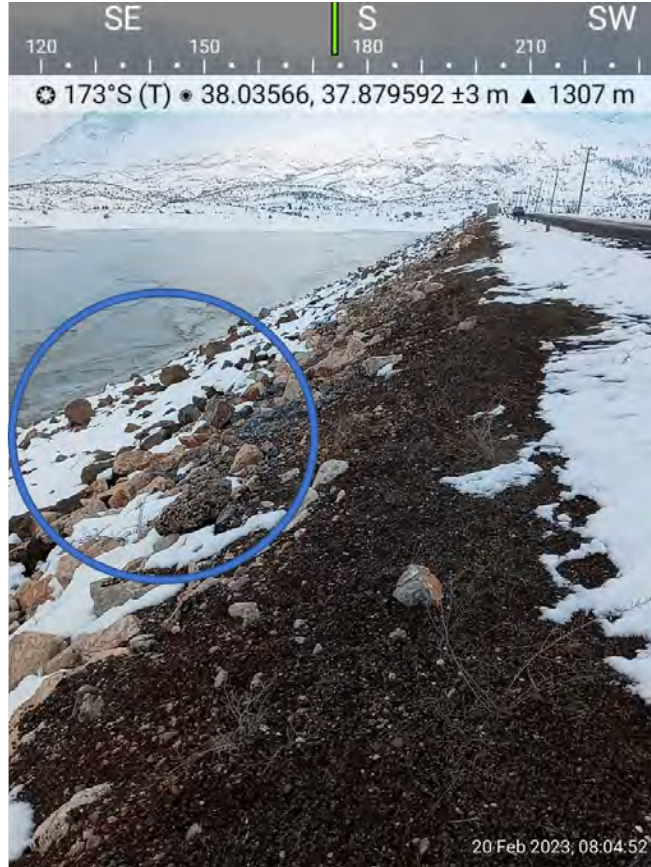
Figure 8.6. Bulging on the upstream face (circled) is coincident with the location of the crest cracking which may indicate seismic induced slope deformations.
