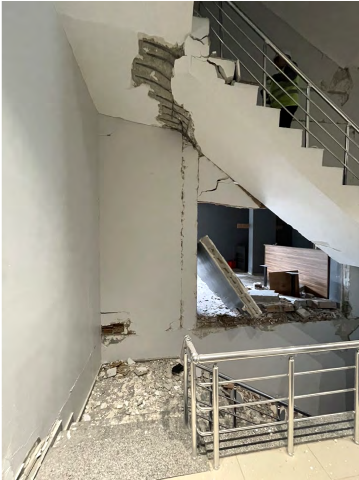
Figure 5.90. Structural damage to a stairwell in a residential buildings in Malatya (including debris from failed masonry infill wall)
