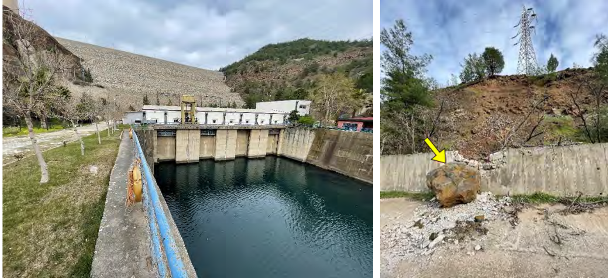
Figure 7.24. Example of rockfall at Menzelet dam.
