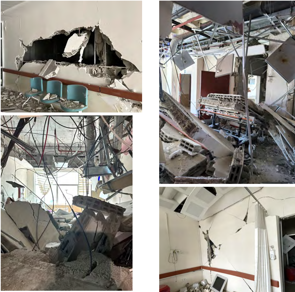
Figure 6.7. Masonry partition wall damage at Türkoğlu Dr. Kemal Beyazit Government Hospital as observed on March 13, 2023, PGA = 0.57g, PGV = 103 cm/s.
