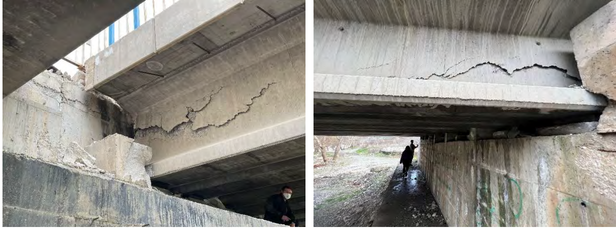
Figure 7.6. Longitudinal cracking at end of precast concrete girders.
