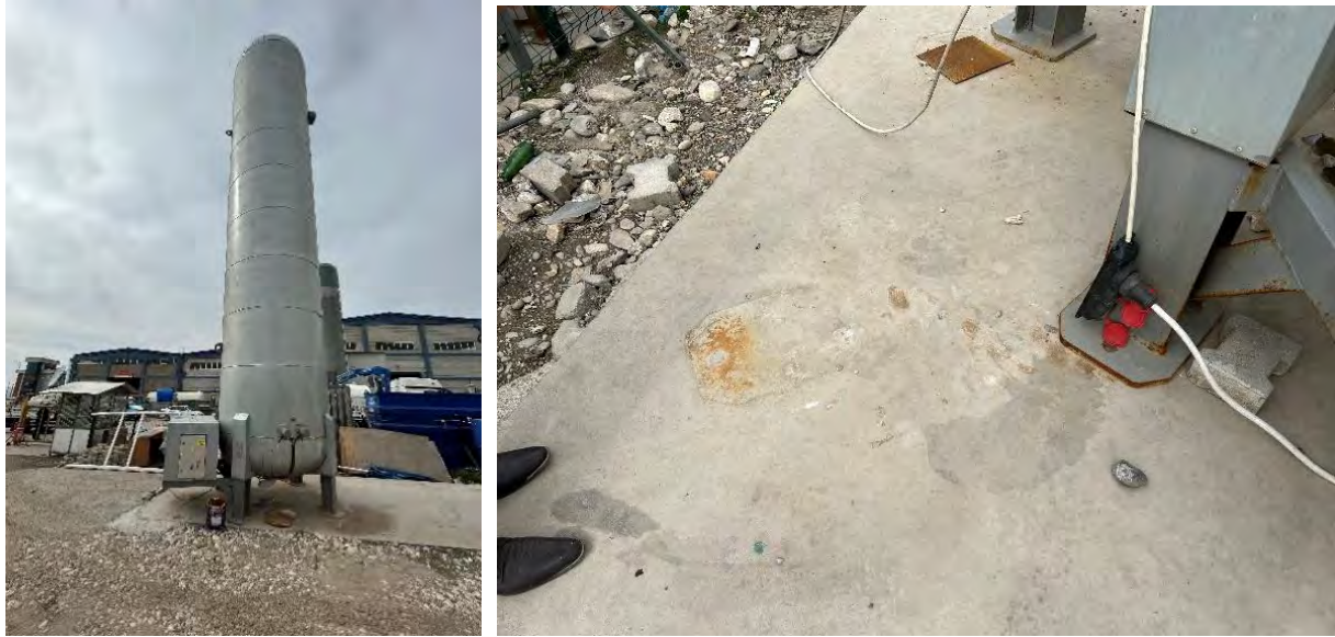
Figure 7.37. 45 metric-ton unanchored vertical tank moved 90 cm laterally at LPG storage facility in Kahramanmaraş (ID 143 in Appendix A).
