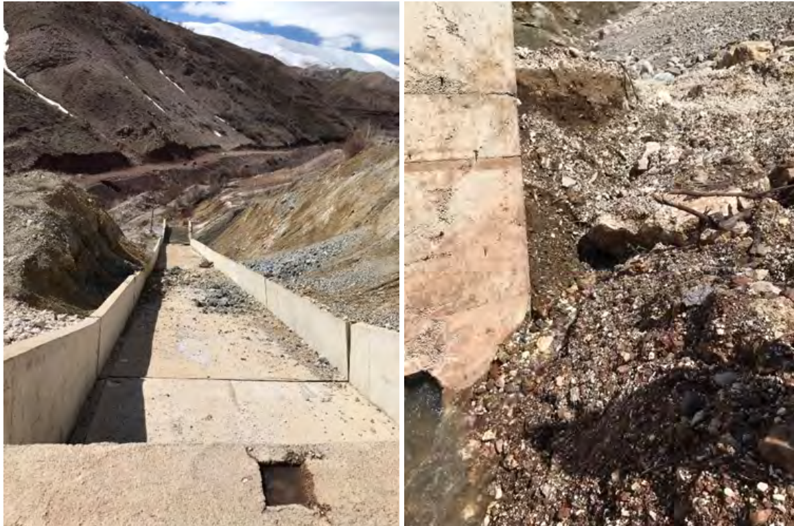
Figure 8.22. Left image, outlet structure of Erkenek dam. Right image, water issuing from the base of the outlet structure that appeared after the events.
