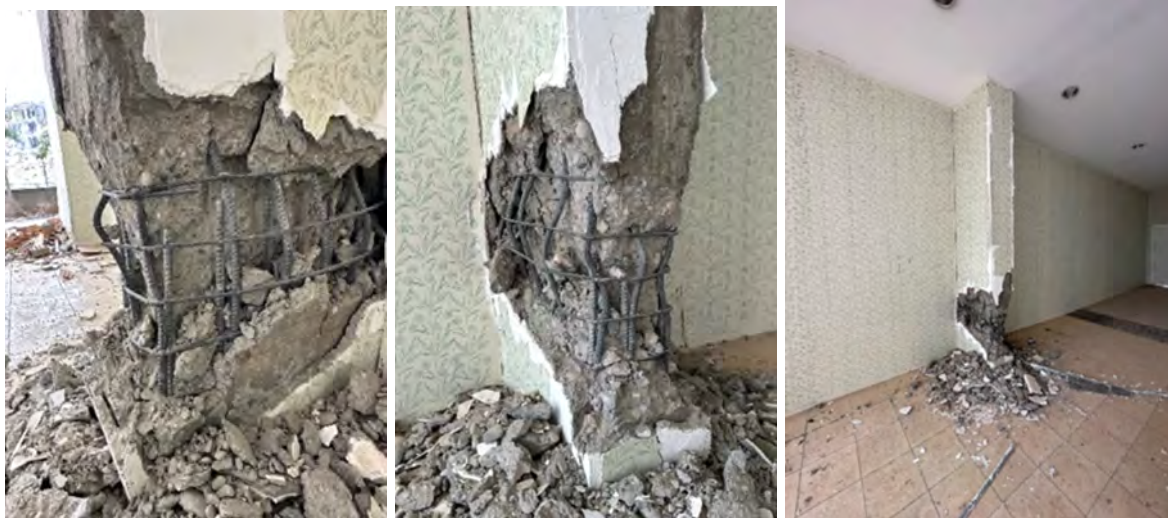
Figure 5.34: Failure of a column with lap splices near the bottom and insufficient transverse steel.
