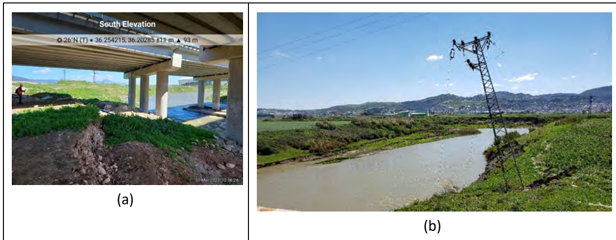
Figure 4.80. Local slope failures near Hatay Stadium Bridge: (a) slumping beneath west end of bridge (N36.254215°, E36.20285°), (b) translational stability failure on east bank and rotational failure affecting transmission lines on west bank of Karasu river (N36.253994°, E36.202873°).
