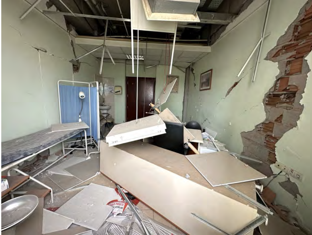
Figure 5.85. Toppling of large storage shelf in a hospital room in Kırıkhan (along with damage to masonry infill walls and suspended ceilings).
