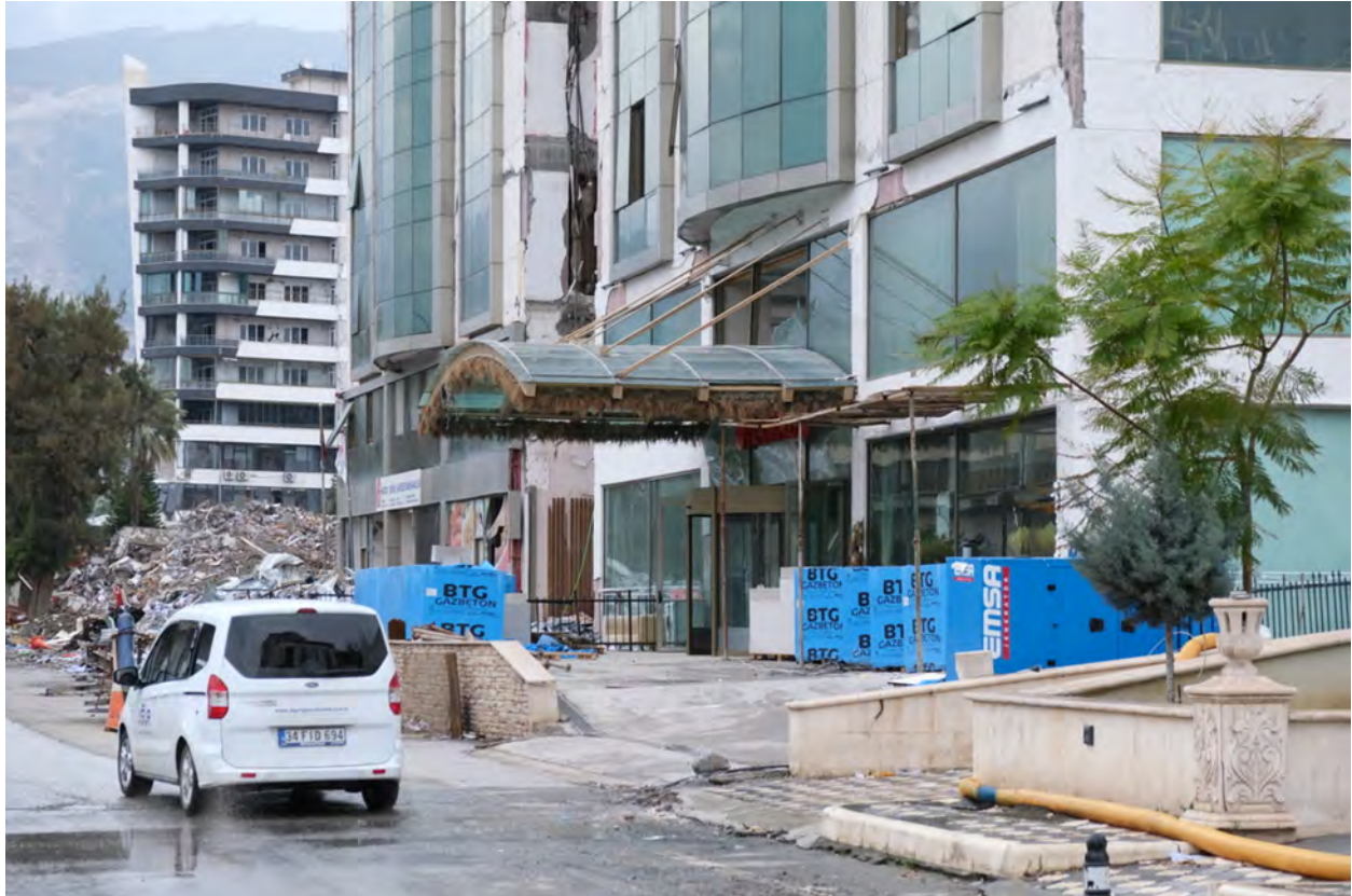
Figure 5.70. Damage to individual glass panels in storefront glazing facade in commercial building in Iskenderun.
