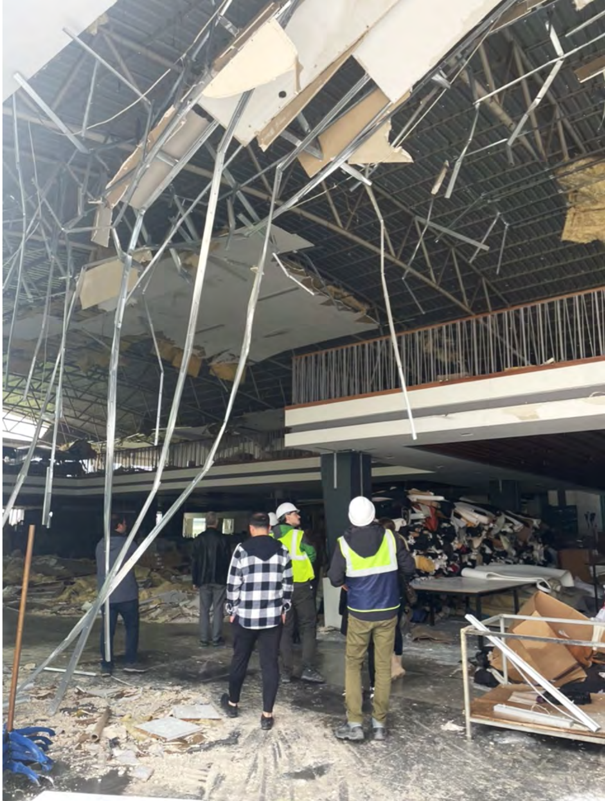
Figure 5.83. Loss of gravity support of suspended ceiling in commercial building in Kahramanmaraş.
