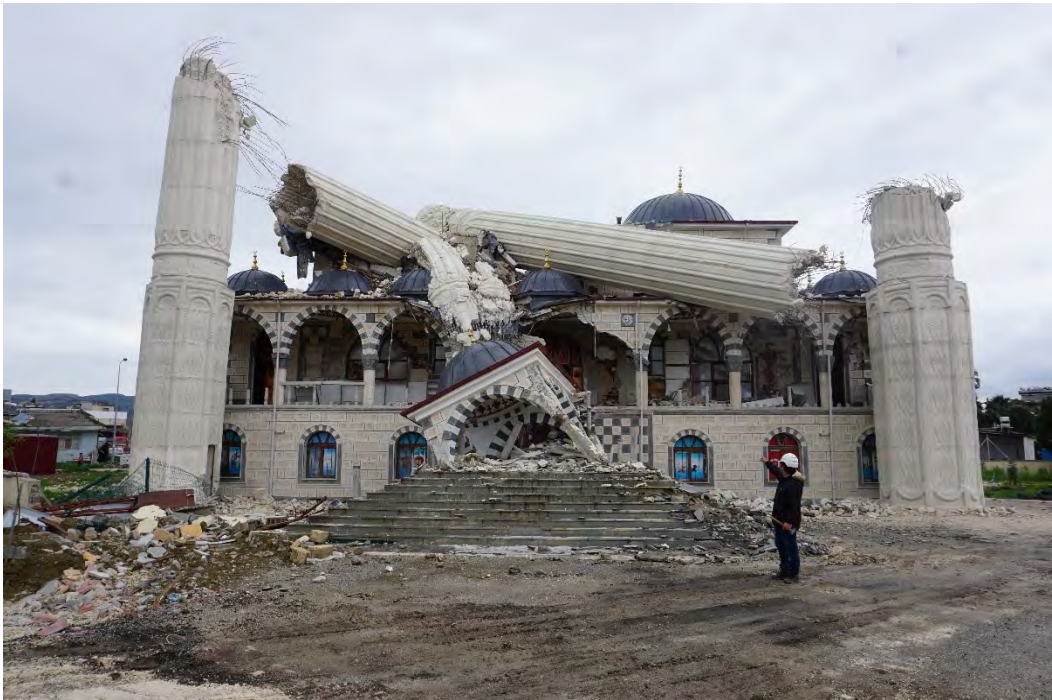
Figure 5.53. Damage to the Odabaşı Camii mosque north of downtown Antakya.
