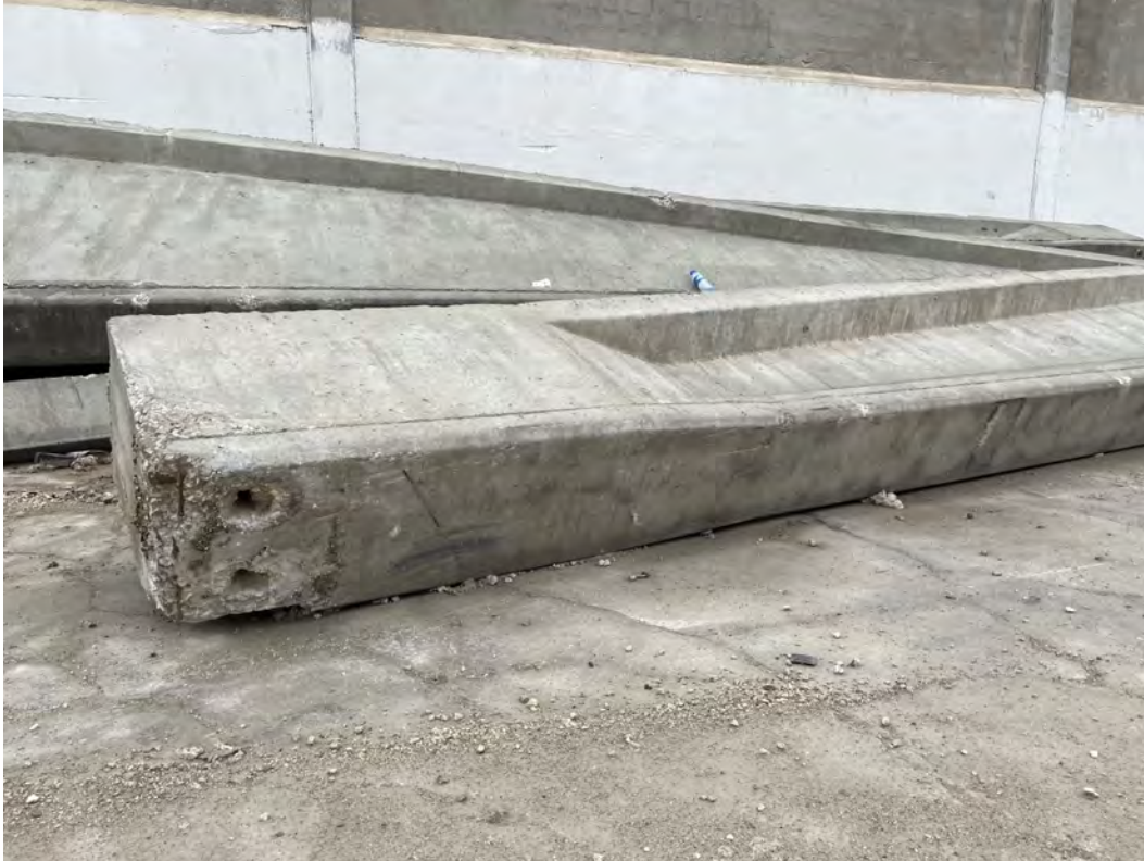
Figure 5.63. Precast connection at failed girder of Kırıkhan industrial building shown above.
