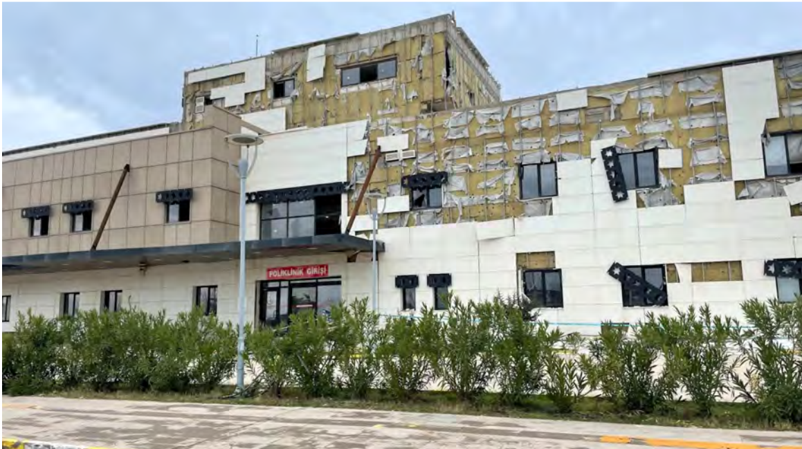
Figure 6.5. Nurdağı Government Hospital as observed on March 17, 2023. PGA = 0.55g , PGV = 86 \text{ cm/s} . This small local hospital (25 beds) was only one year old at the time of the earthquake. It suffered widespread nonstructural damage, but only limited structural damage. It was immediately evacuated and closed. An emergency tent hospital was set up on the premises to serve the community.
