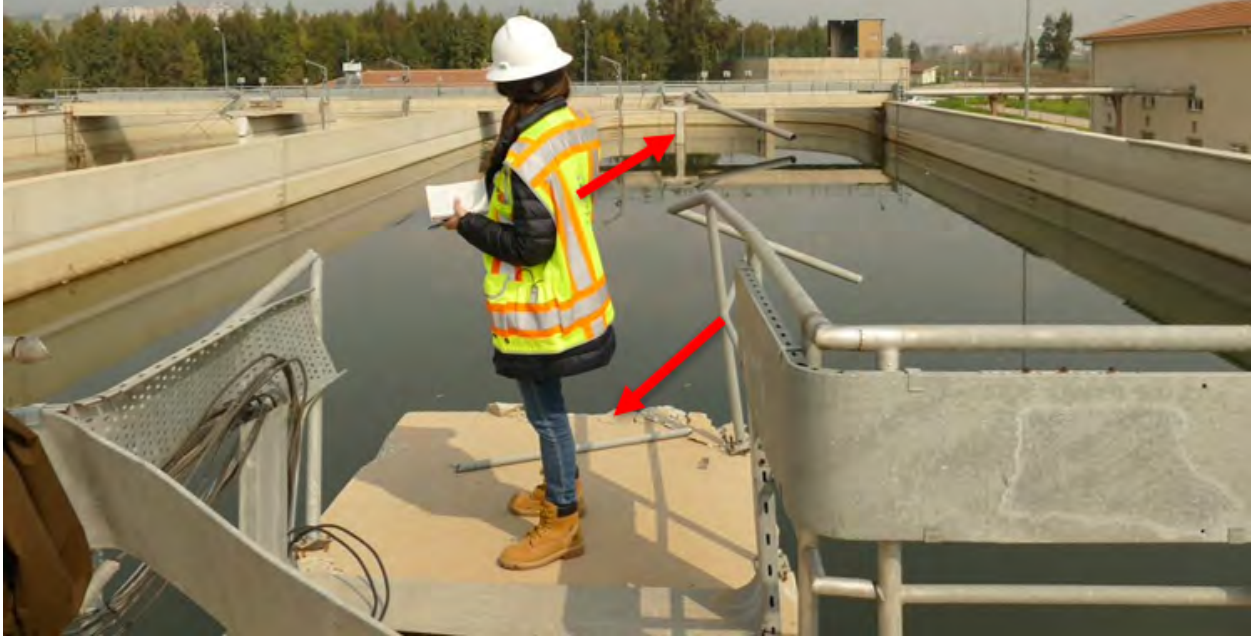
Figure 7.52. Collapsed central dividing wall (between arrows) and damaged piping now submerged within aeration tank (Kırıkhan, Hatay) (ID No. 30 in Appendix A).
