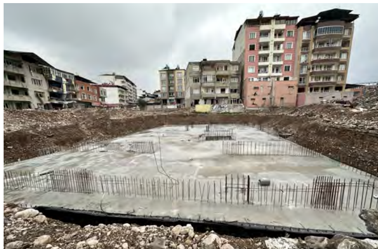
Figure 5.36. Short lap splices above the foundation at the bottom of first columns and story shear walls in a building under construction.
