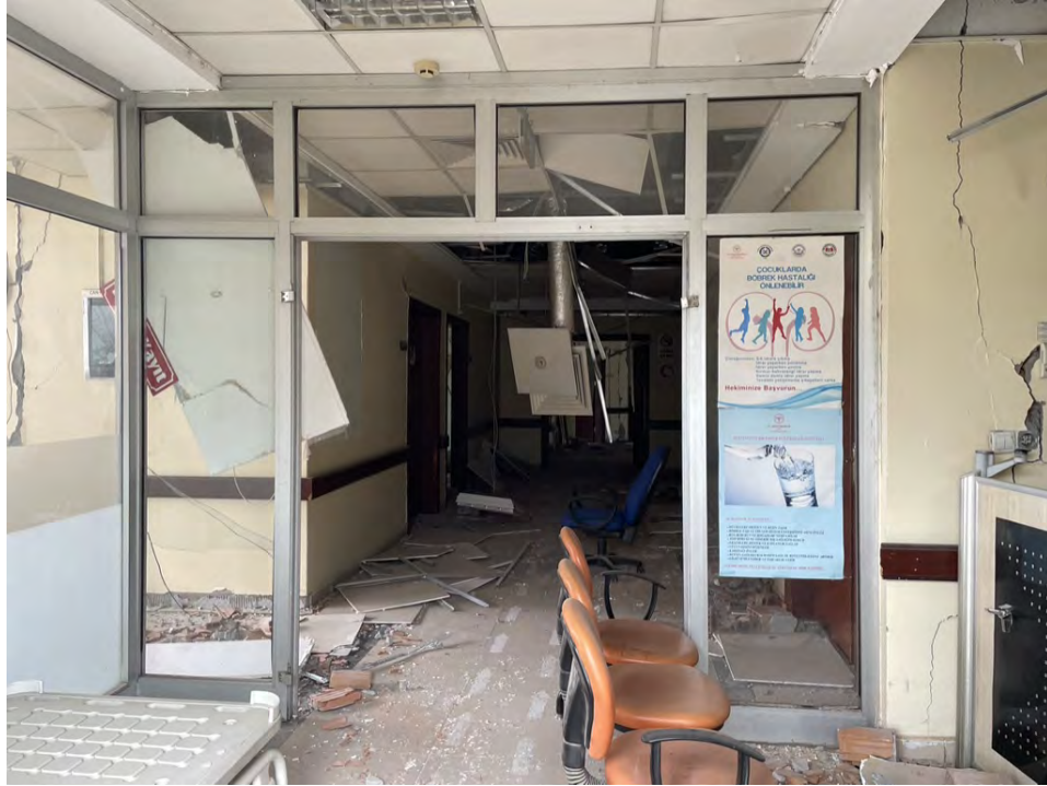
Figure 5.80. Fallen ceiling tiles and HVAC ducts near a hospital entrance in Kırıkhan.
