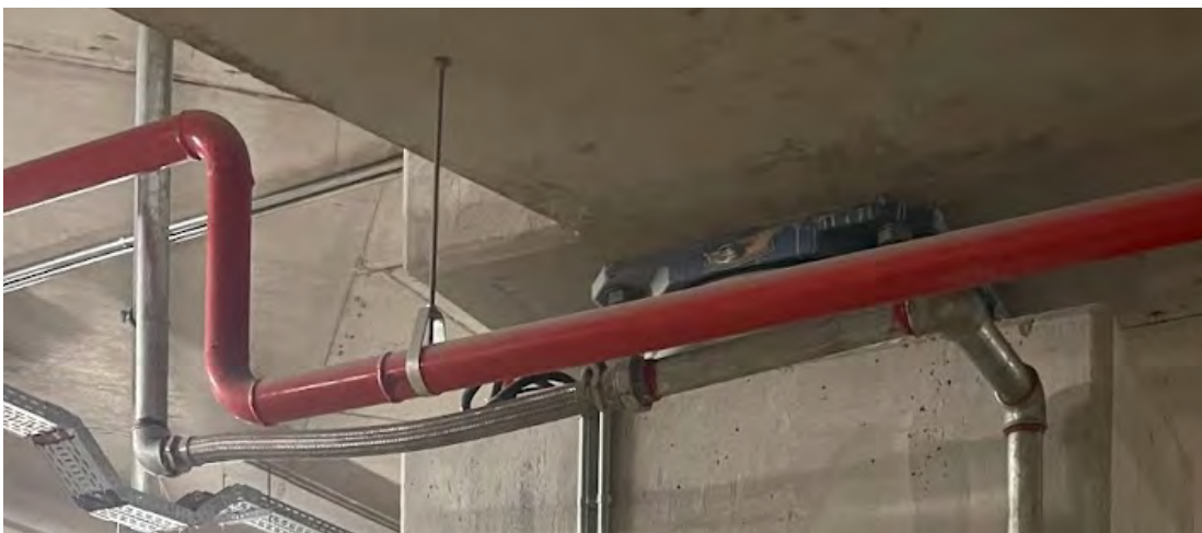
Figure 6.22. Utilities crossing isolation plane as observed at the Adana City Hospital on March 16, 2023.
