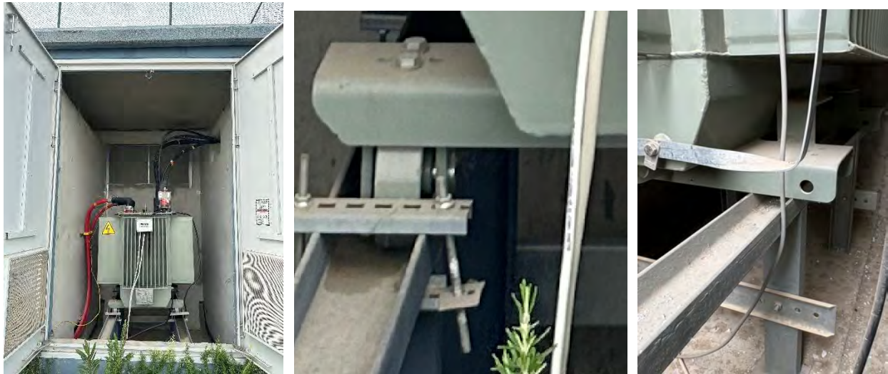
Figure 7.65. Example of transformers without vertical restraints that were undamaged
