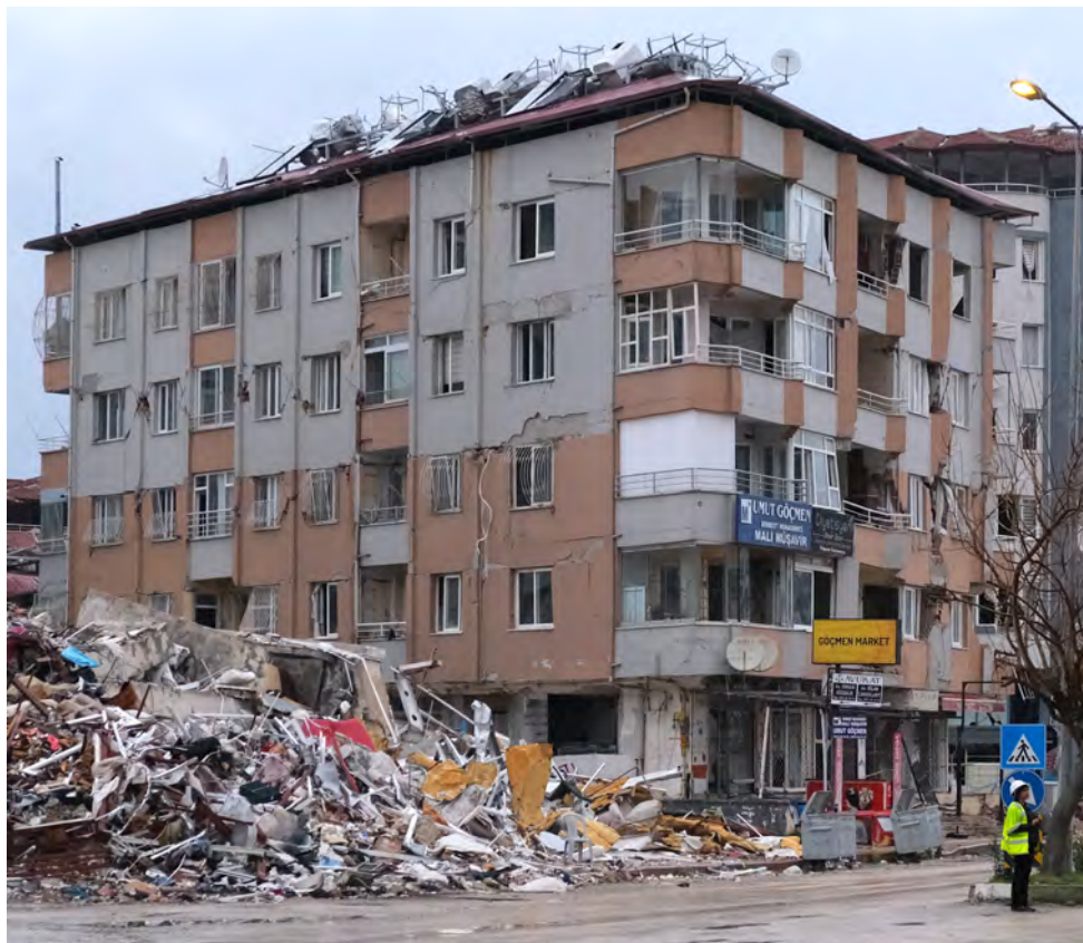
Figure 5.78. Failure of rooftop solar water heaters in Antakya.
