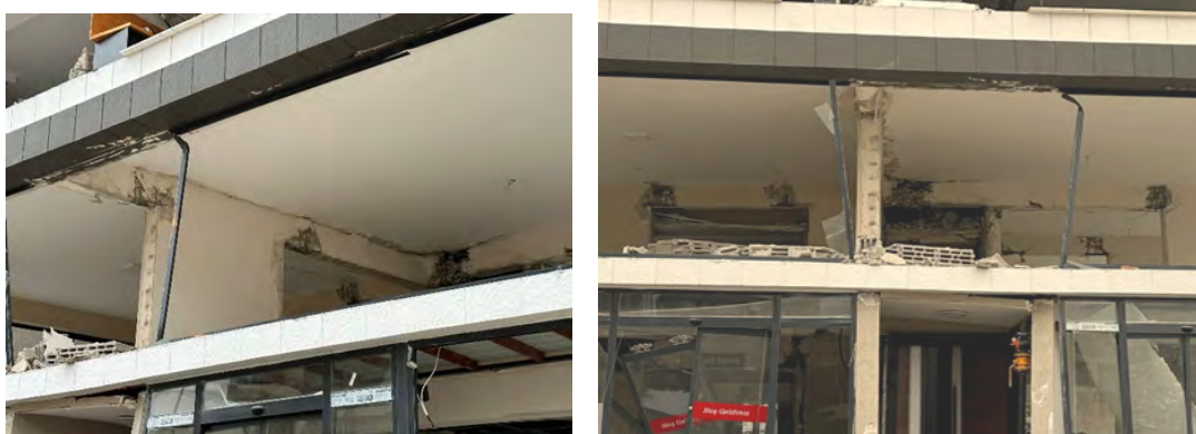
Figure 5.27. Plastic hinges at beam ends.
