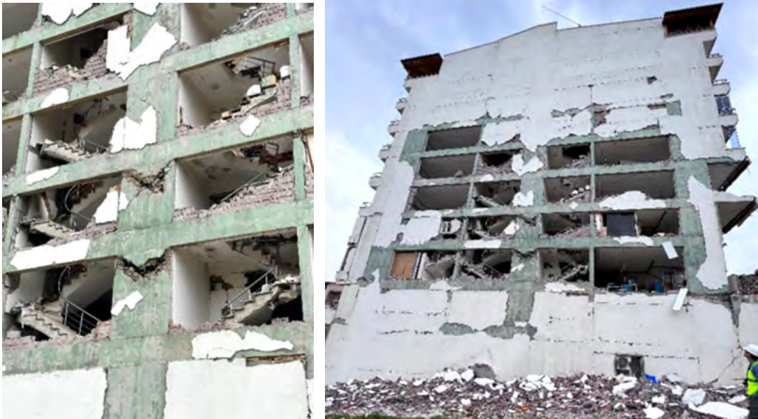
Figure 5.38. Damaged shear walls in the lower stories of a building.
