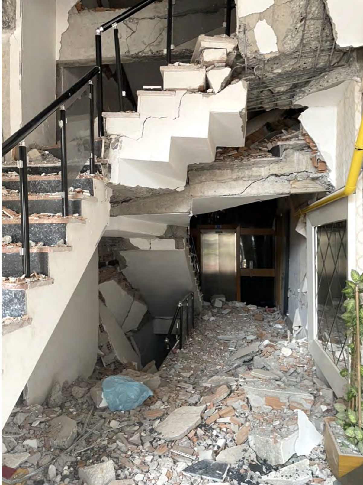
Figure 5.89. Structural damage to a stairwell in a residential buildings in Adiyaman (including debris from failed masonry infill wall)
