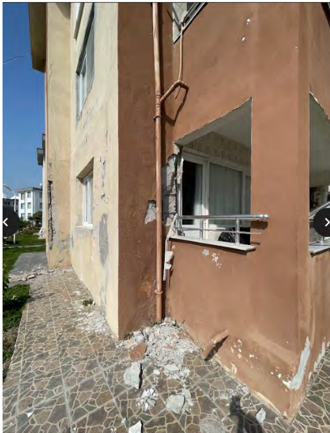
Figure 4.57. Building damage in the Öğmeiř neighborhood related to settlement. Photo taken March 3, 2023 (Coordinates: 36.79628, 36.19710).
