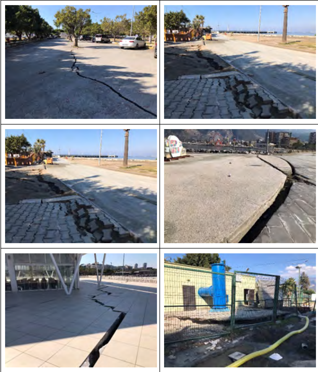
Figure 4.25: Examples of liquefaction-induced lateral spreading at Atatürk Boulevard (36.59147 N, 36.174378 E).
