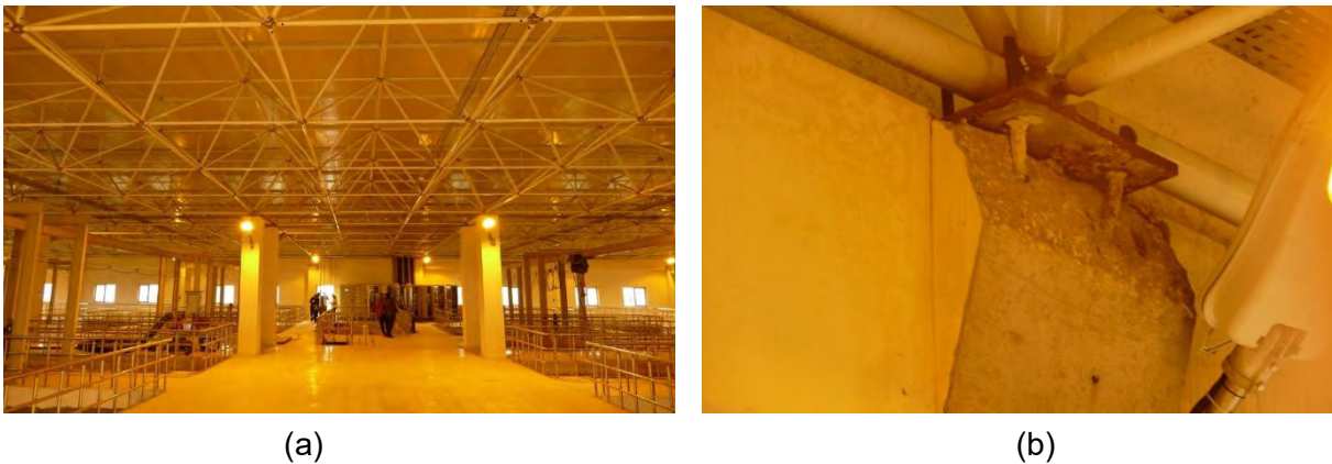
Figure 7.46. (a) Interior overview of light-weight, space truss roof framing system within sedimentation-tank building. Truss is uniform with no enlargement of cross-tie chord members. (b) Concrete breakout damage at anchorage of roof space truss node to corbel at the exterior concrete wall. Anchorage damage beyond minor cracking was observed in very few locations.
