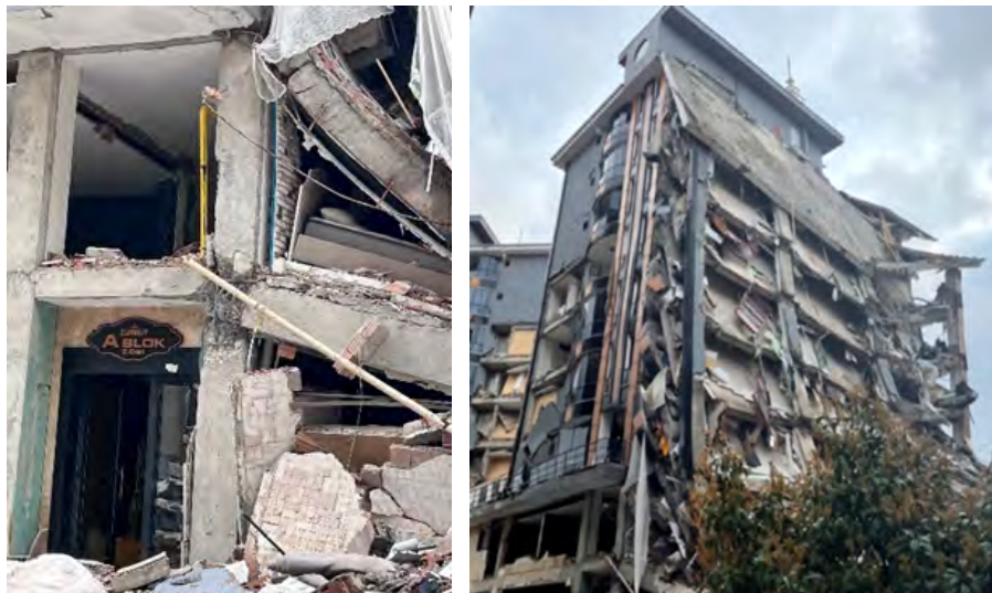
Figure 5.31: Column joint region with no transverse steel, which is exposed after the right side of the building collapsed.
