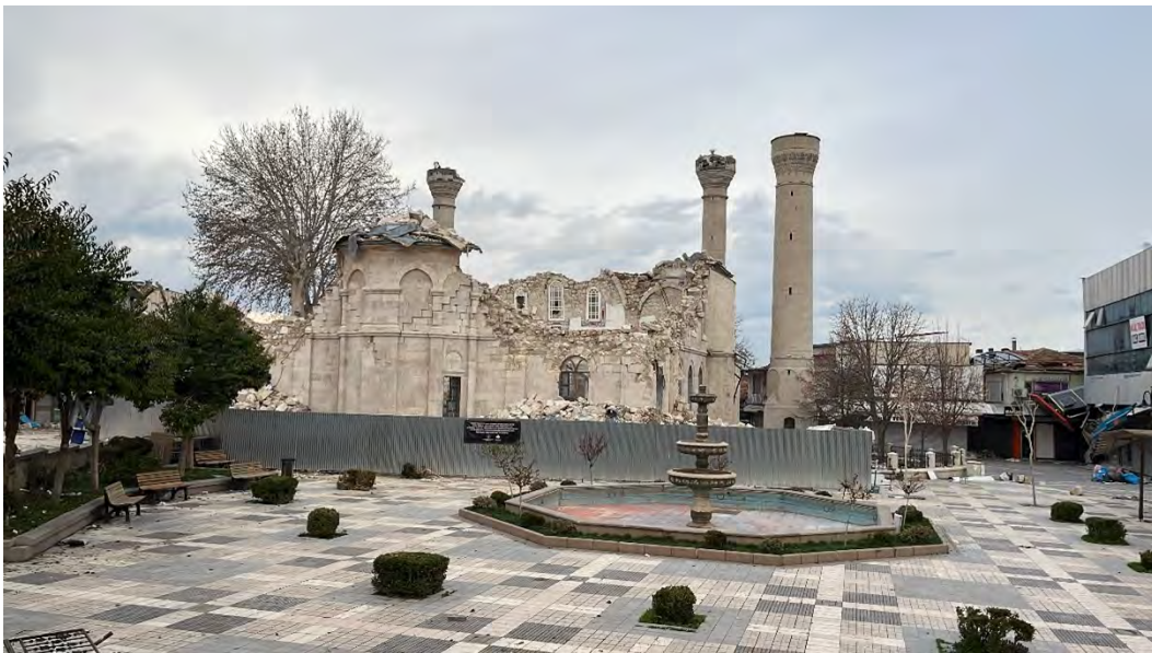
Figure 5.60. Damage to Yeni Cami mosque in Malatya.
