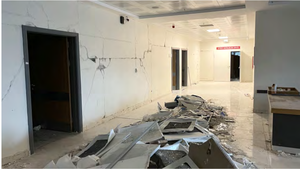
Figure 6.13 Interior partition damage and ceiling repair.
