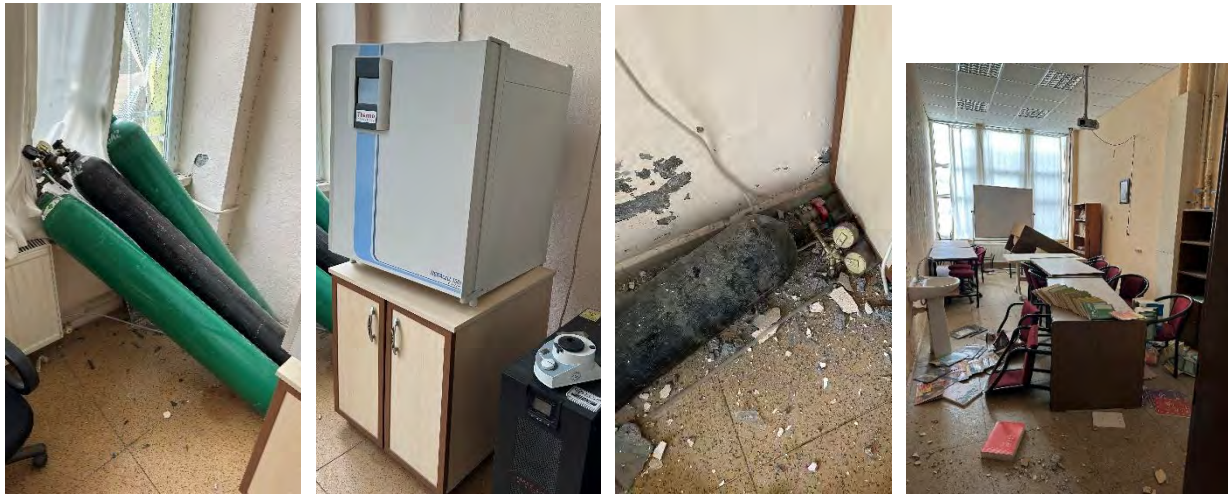
Figure 7.63. Example of displaced and toppled equipment at the Agricultural Science building.
