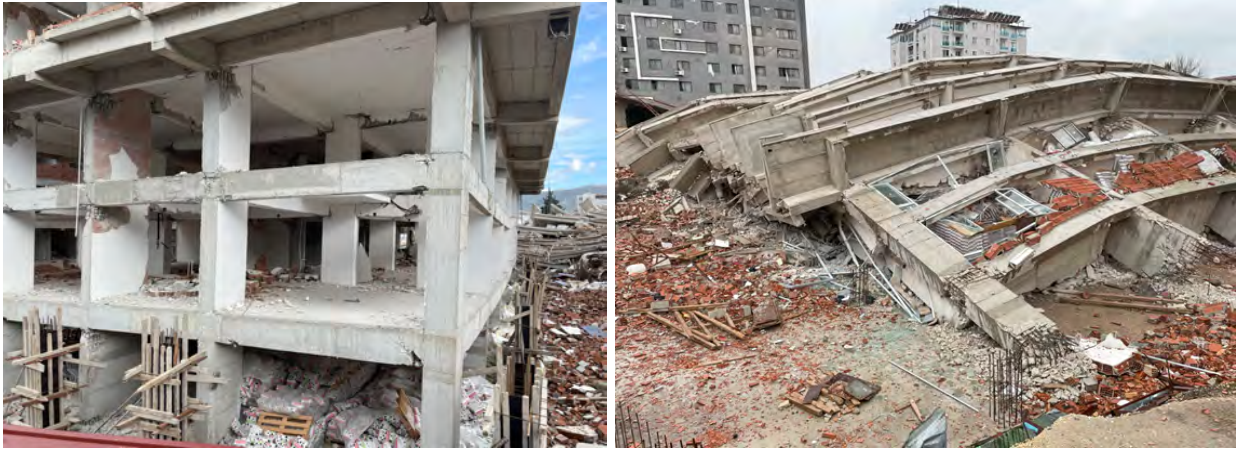
Figure 5.12. RC shear wall frame system building under construction, Antakya (yielding in beams and shear walls on the left; collapsed structure on the right)
