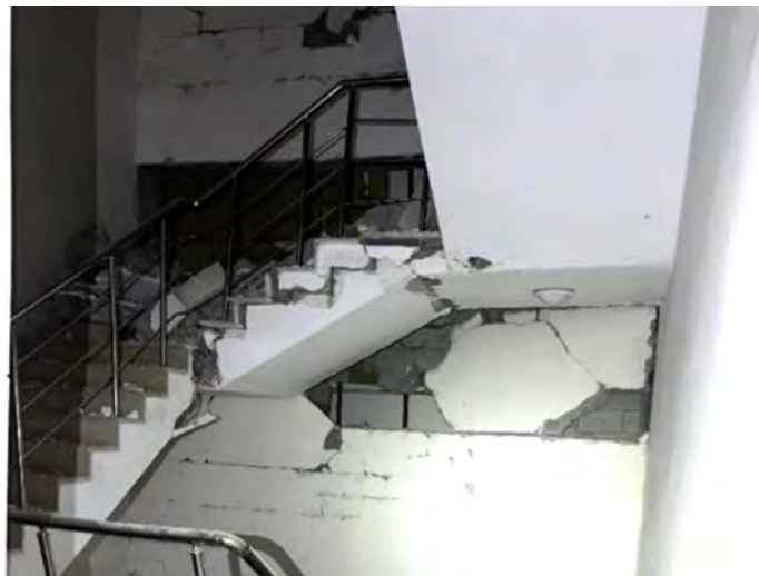
Figure 6.9 Egress stair adjacent to masonry wall at Türkoğlu Dr. Kemal Beyazit Government Hospital as observed on March 13, 2023.
