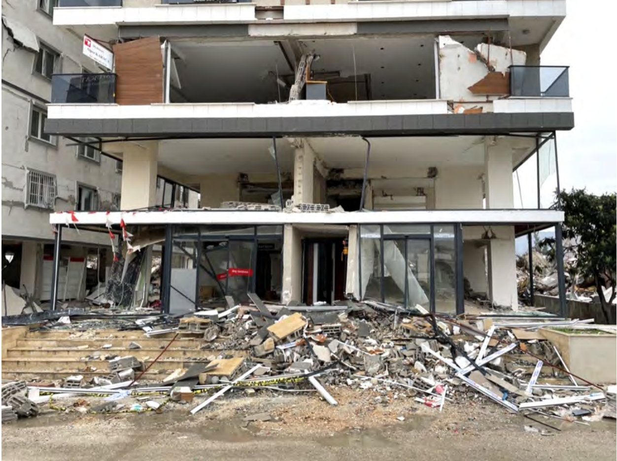
Figure 5.71. Damage to metal frame and glass panels in storefront glazing facade in mixed use building near Antakya.
