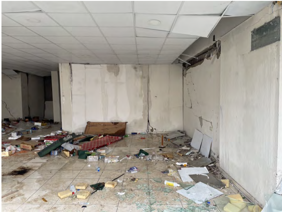
Figure 5.81. Failure of perimeter metal framing of suspended ceiling in mixed use building in Hassa.
