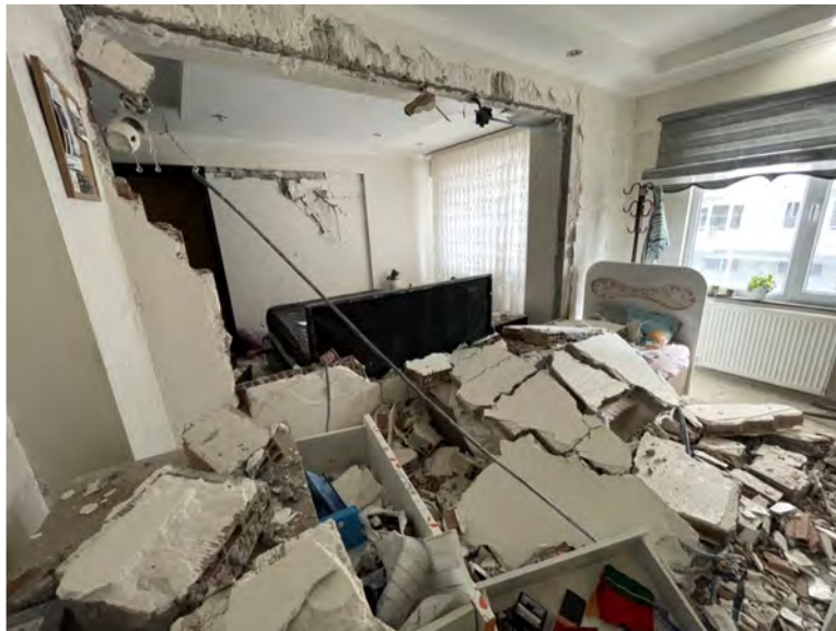
Figure 5.74. Failure of infill partition in a residential building near Malatya.
