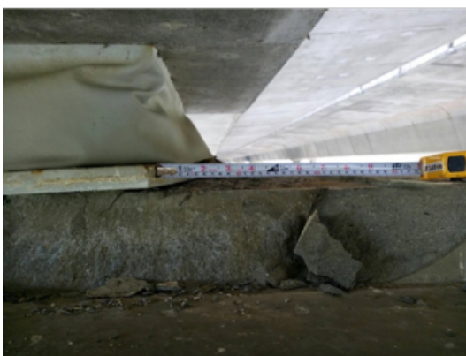
(c) Damages caused by excessive displacement of bridge bearings
