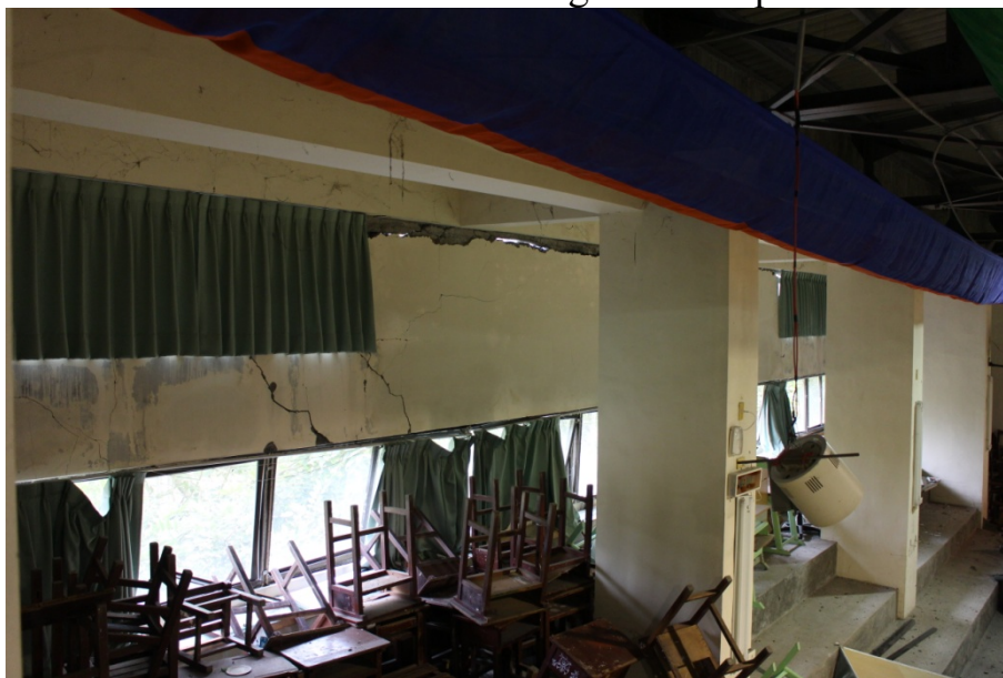
Figure 2.14 Activity Center. Cracks at the interface between the bottom of the beam and the brick wall at the bottom
