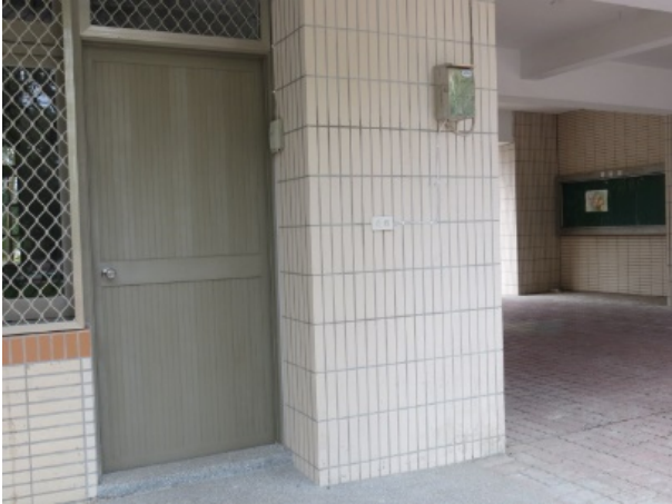
Figure 2.22 Yangming Building. No structural damage.
