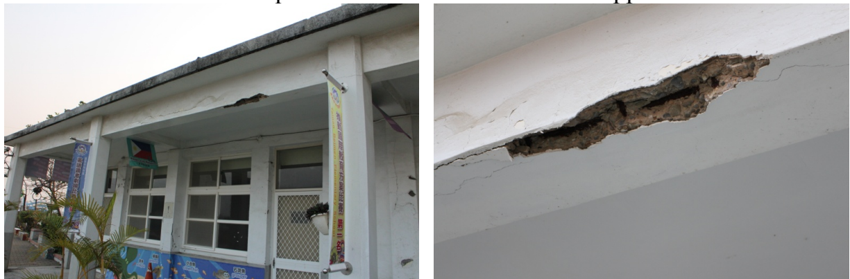
Figure 2.21 West Block. Concrete peeling off from at the bottom of a column at the corridors. The exposed reinforcements were rusted which was probably not caused by this earthquake.
