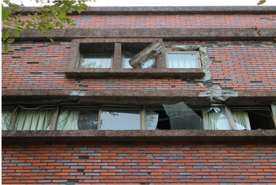
Figure 2.17 Activity Center. Concrete blocks forming the windows' outer frames hanging precariously as well as broken window panels.
