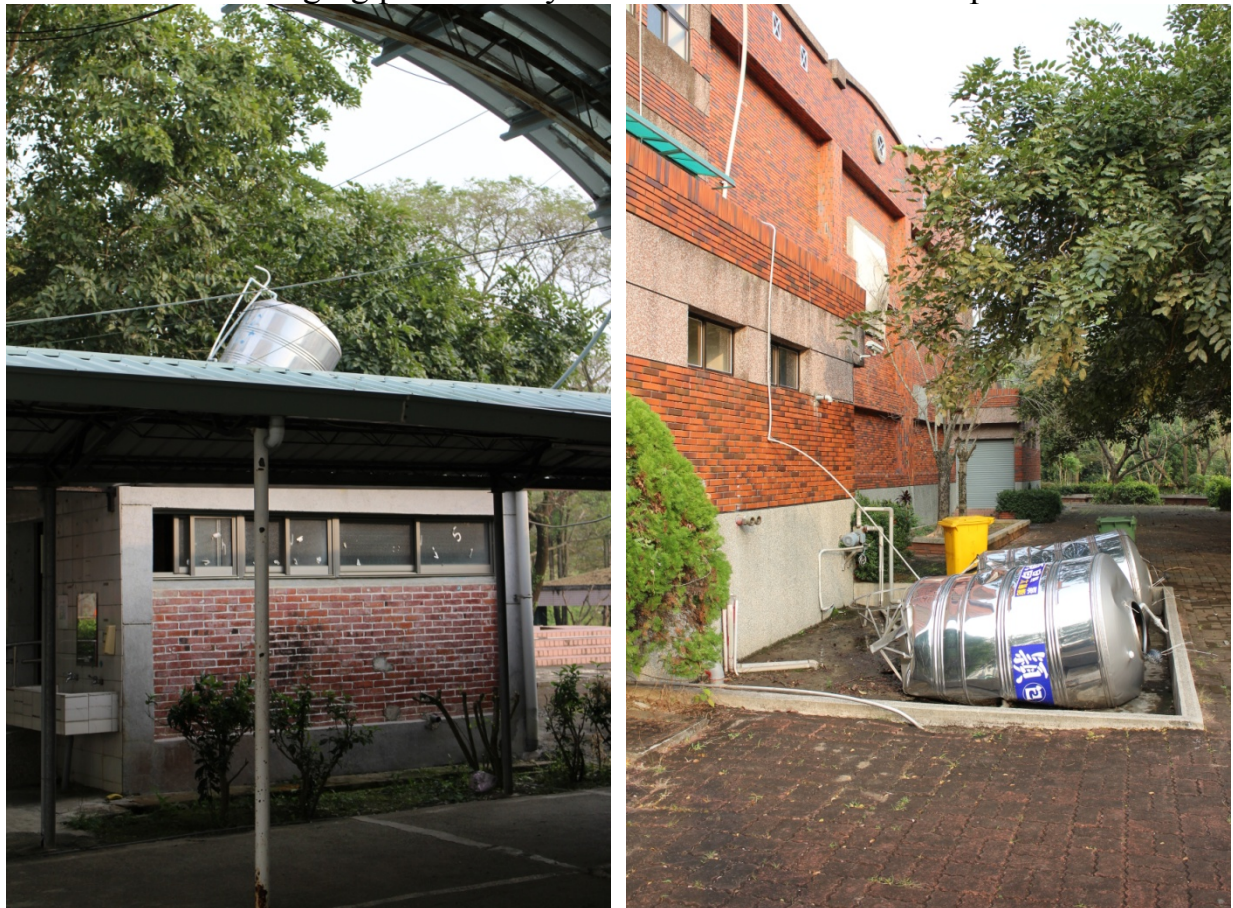
Figure 2.18 Failure of many stainless steel water tanks at Yujing Junior High School
