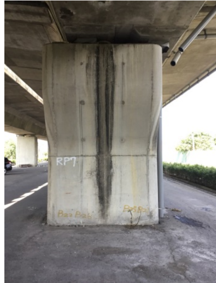
(b) Damages to drainage pipelines caused by excessive displacement of bridge decks
