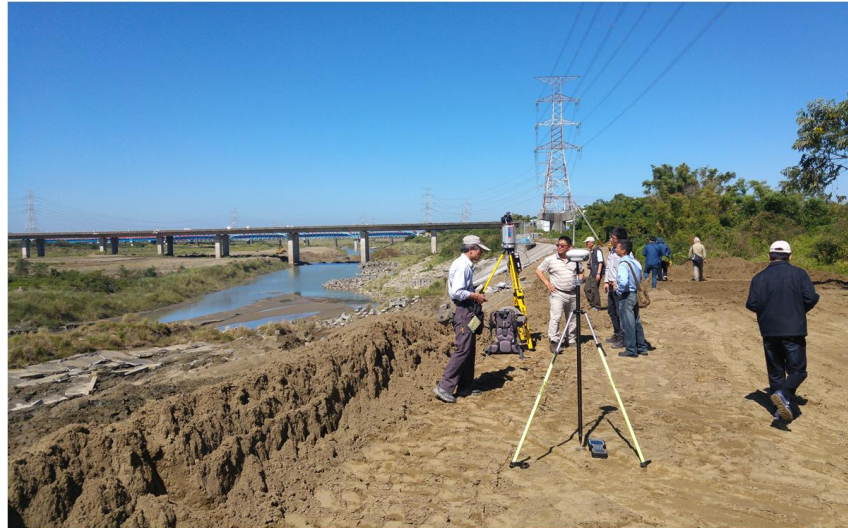
Figure 4.3 Supporting companies conducting digital topographic scanning and mapping at the lateral spreading site of Rixin embankments (provided by Shang-Yi Hsu)
