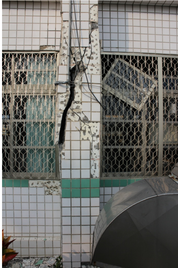
Figure 2.11 Severe shearing damages at the backside of the window columns
