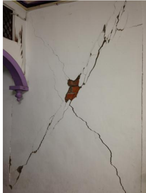
(b) X-shaped shearing cracks on the brick walls
