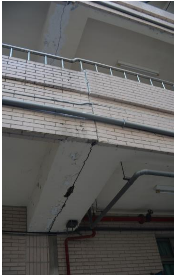
Figure 2.28 Gezhi Building. Damages to the expansion joints
