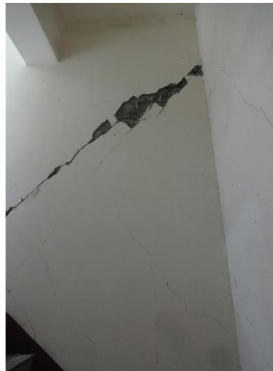
(b) Shearing damages of staircase walls
