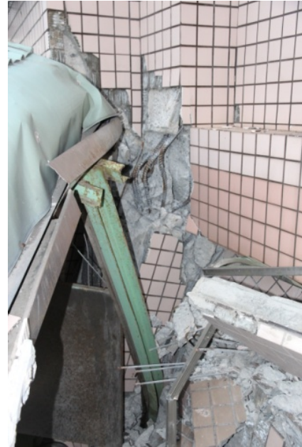
(b) Damaged connectors at the columns and beams
