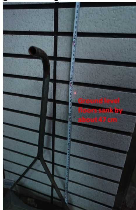
(C) Ground level floors sank by about 47 cm
