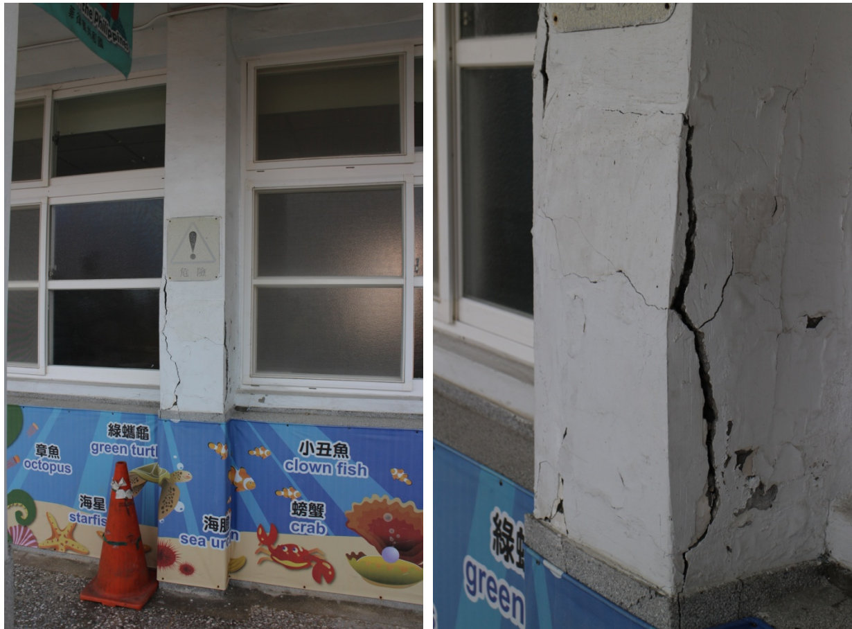
Figure 2.20 West Block. Vertical cracks on the building's columns probably caused by corrosion and swelling of the steel reinforcements contained within. This earthquake than caused the cracks to appear.
