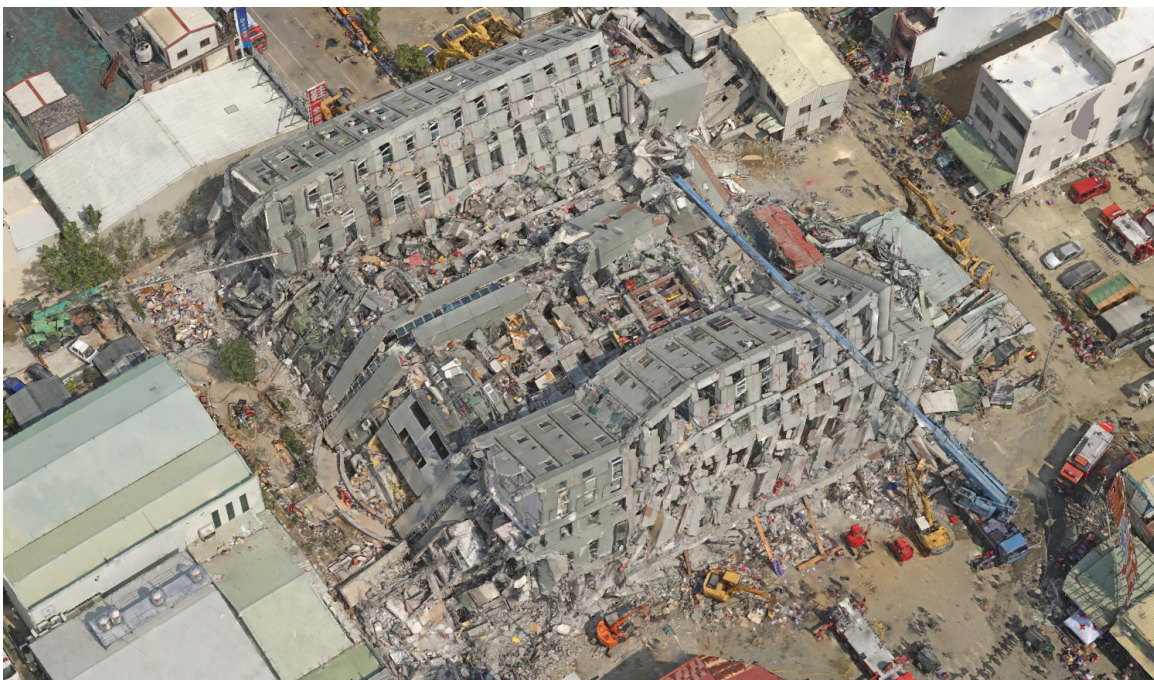
Figure 2.1 Aerial photographic view after the collapse of the Weiguan Jinlong Building in Yongkang District (provided by Ren-Zuo Wang)
