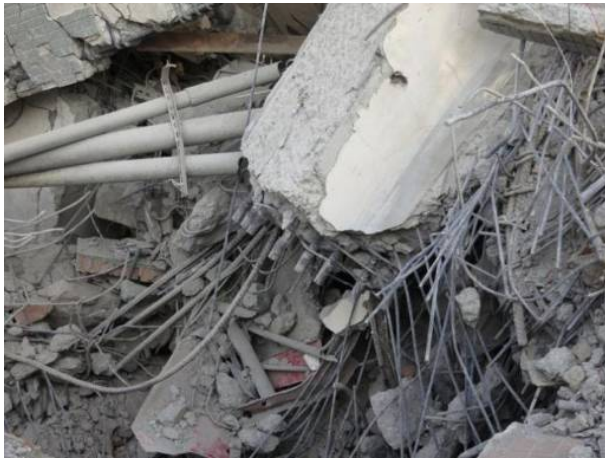
(a) Rebar coupler splices were located in the same elevation
