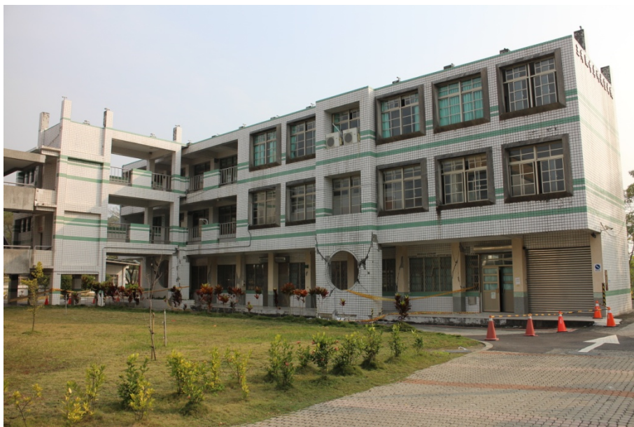
Figure 2.10 Diagonal cracks caused by shearing damages at the 1st floor window columns of the subject classrooms
