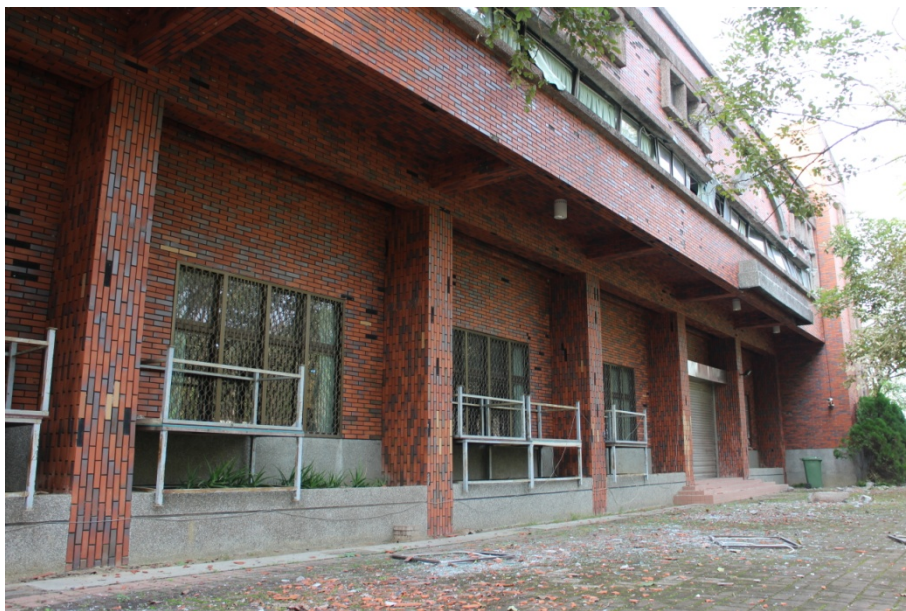
Figure 2.16 Activity Center. Tiles had fallen off the wall surface. A number of windows panels had been subjected to compression and fell onto the ground
