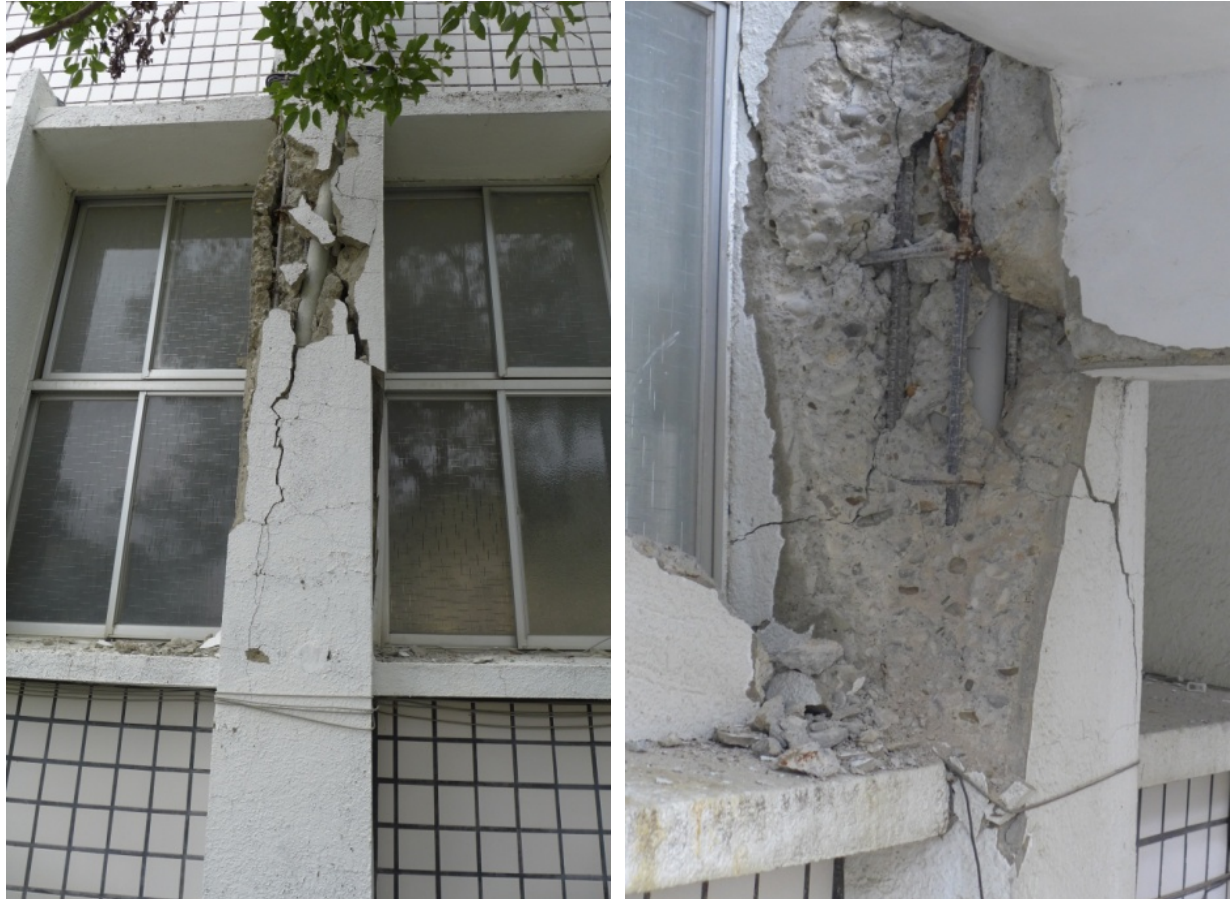
Figure 2.30 Windows have led to short column effects that led to shear failure to a large number of columns during the earthquake
