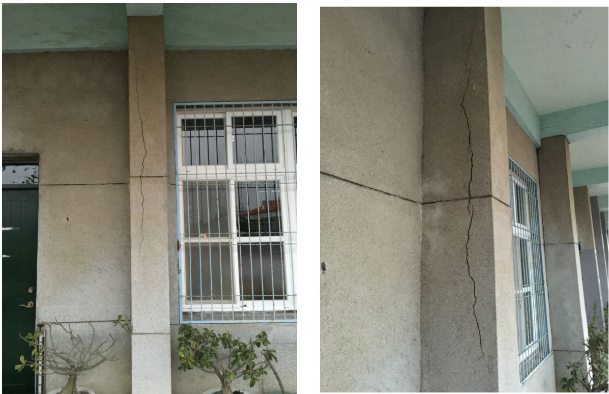
Figure 2.19 West Block. Vertical cracks along the columns. It was suspected that the internal steel reinforcements have become corroded and swollen. The earthquake simply enlarged the cracks.
