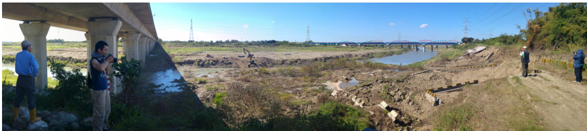
Figure 4.4 Lateral spreading damages at the embankments of Zengwun River Bridge at Freeway No. 3 (provided by Shang-Yi Hsu)
