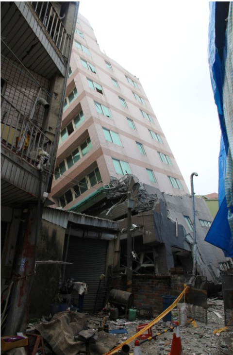
(a) Damages to the vertical elements at the bottom floors
