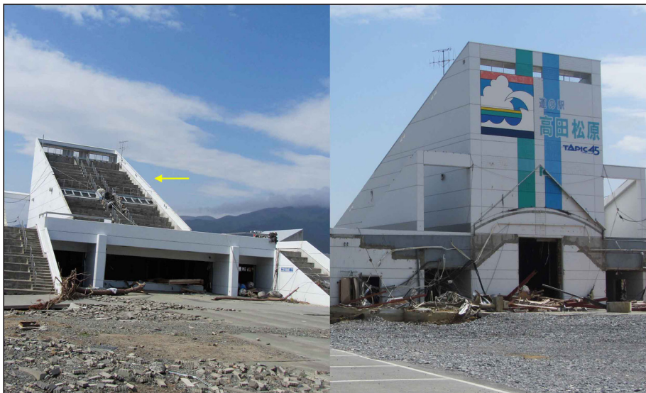
Figure 5. Tsunami evacuation building, Rikuzentakata. Measured water levels were 19 m, shown by the yellow arrow (photos: L. Dengler).
