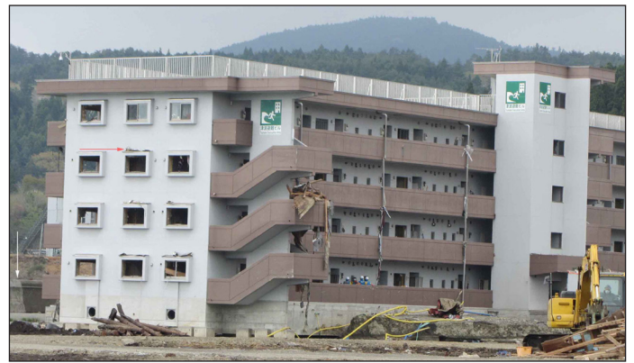
Figure 25. Tsunami evacuation building in Manamisanriku (B on map, Figure 8). The building is adjacent to the sea wall (white arrow on the left). The tsunami left debris on the fourth floor windows (red arrow) (photo: L. Dengler).
