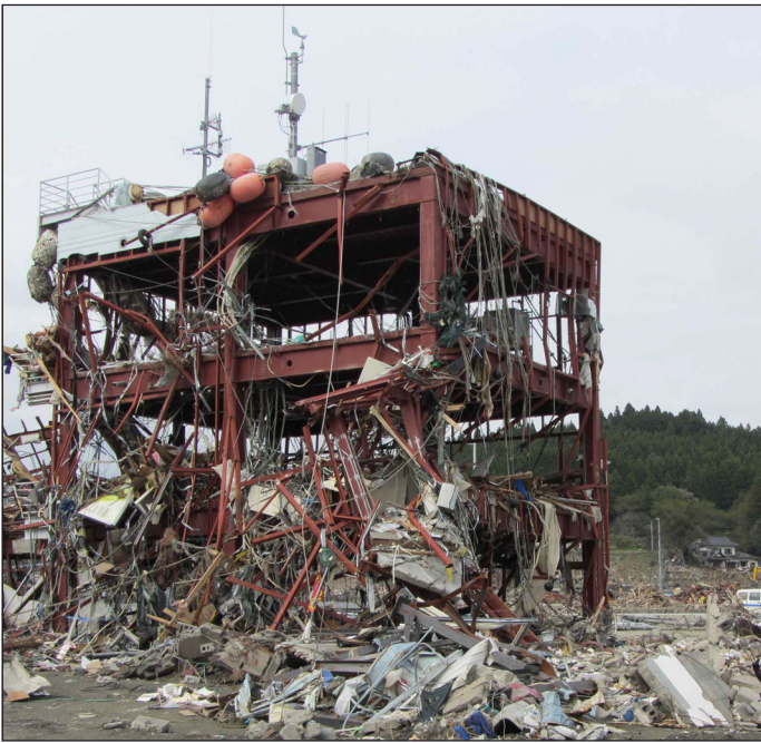
Figure 10. The disaster management headquarters for the town of Minamisanriku. About 30 officials gathered on the upper floor and roof on March 11. The tsunami completely flooded the structure and only 11 people survived. Note the location of high ground in the background (photo: L. Dengler).
