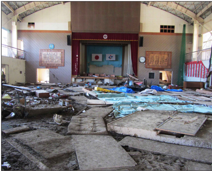
Figure 13. The multipurpose room of the Higashimatsushima elementary school, where 200 people gathered after the earthquake. The site was flooded to the base of the windows and most of the evacuees did not survive. The floor was used as morgue after the tsunami (photo: L. Dengler).
