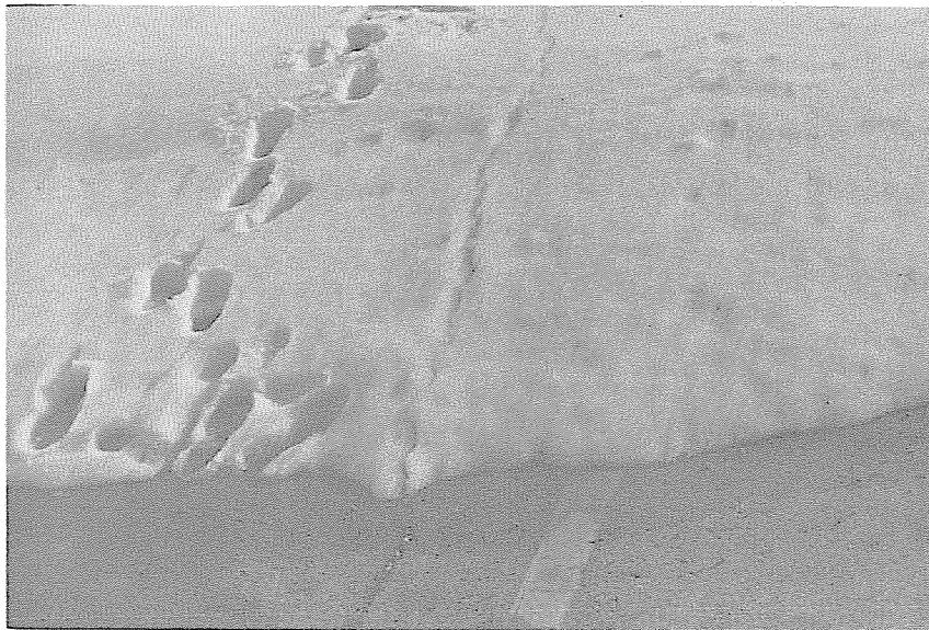
Photo 5 Cracks in parking lot paving projected through snow Former Mammoth Elementary School
