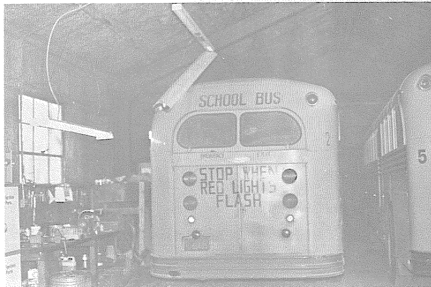
Photo 2 Displaced light fixture in bus garage. Former Mammoth Elementary School
