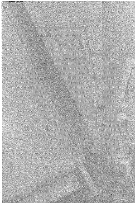
Photo 1 Toppled water tank. Former Mammoth Elementary School
